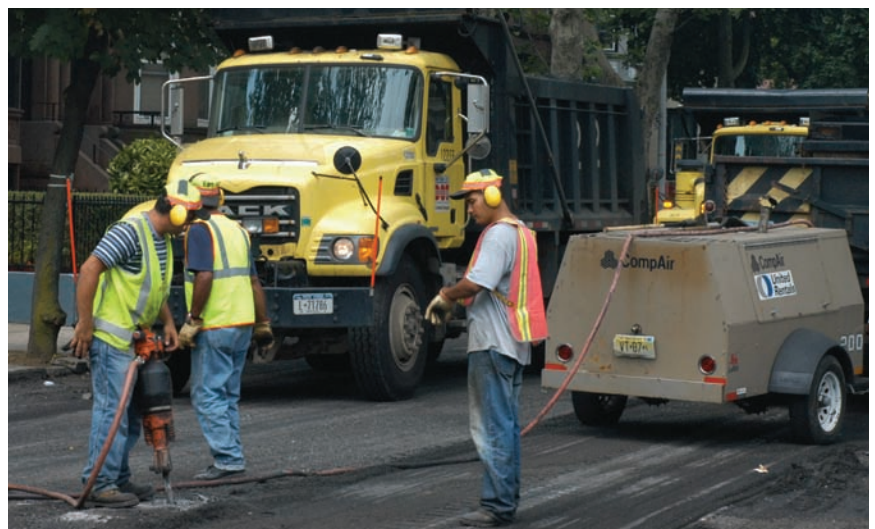
Street resurfacing in progress. NYC DOT’s street reconstruction and resurfacing programs include nearly 6,000 miles of city streets.
