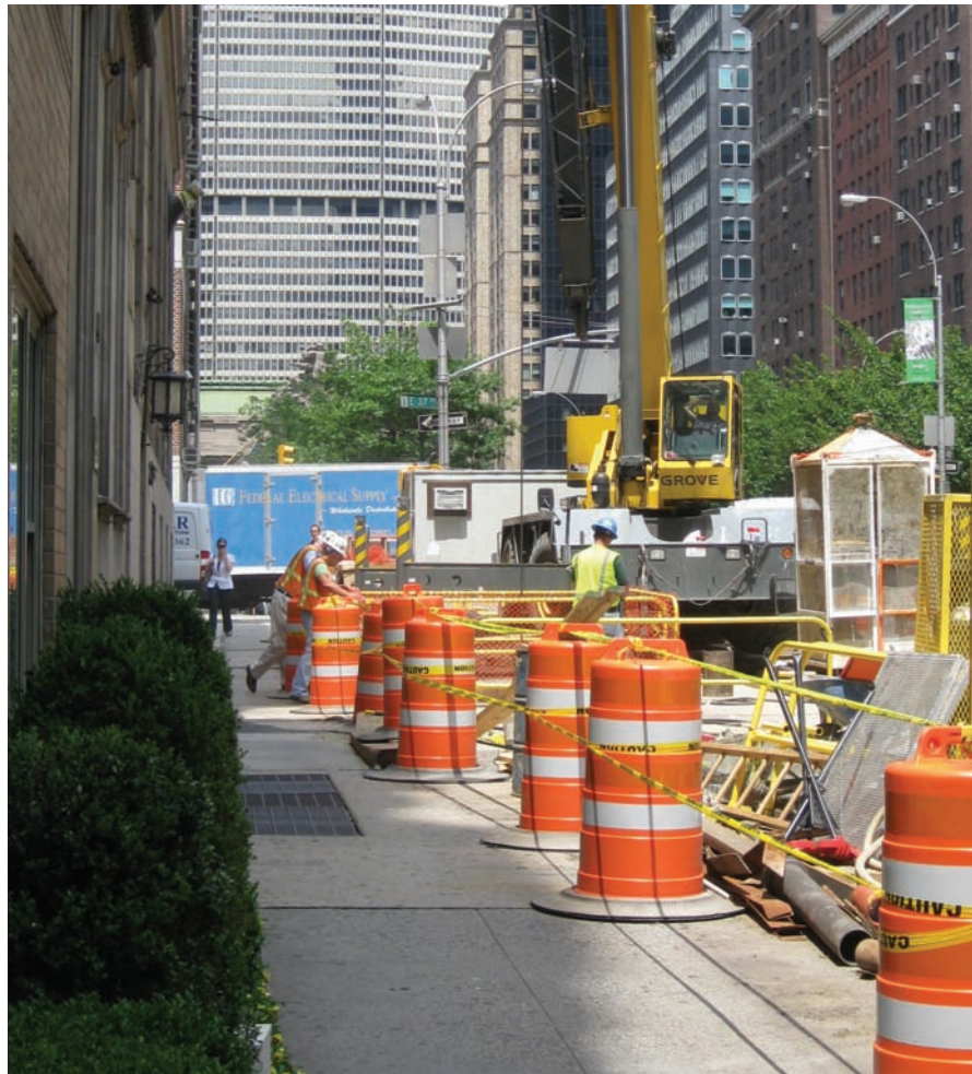
Crane placed on the street for construction activity. Cranes may require permits from DOB in addition to NYC DOT.
