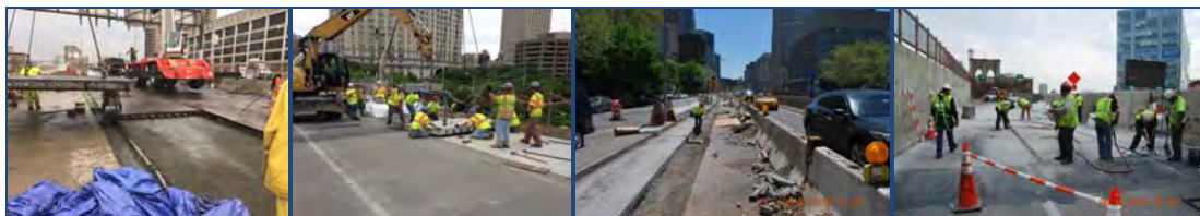
May 2015: Manhattan-Bound Approach SuperSlabs. New Curb Mall and Barrier on Adams Street Access Road. Brooklyn Approach Concrete Headers.
