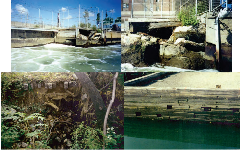
From Study of FDR Drive: Location #2 – Damaged Seawall at Segment #5. Sinkhole at Location #6 at East 59 th Street. From Study of Carroll Street Bridge: General View of the Southwest Crib Wall With the Delamination of the Timber Stretchers in the Tidal Zone.
