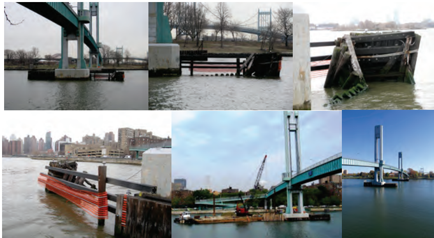
2014 - Wards Island Pedestrian Bridge – Collapsed Fender. July 2015 – Work Barge. November 2015. (2015 Credit: Jitendra Patel)
