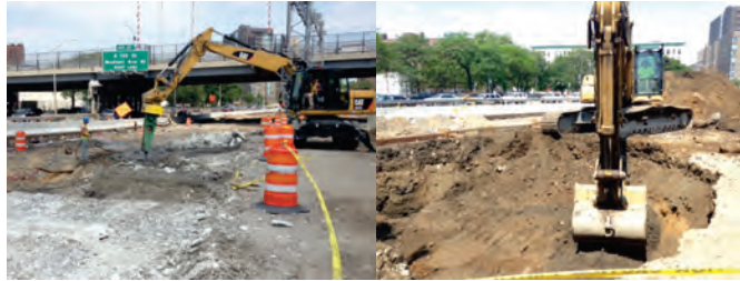
February 2015: Removing the Massive Reinforced Concrete Substructure Near the Third Avenue Bridge. Excavating and Removing Big Rocks. (Credit: Artemio Angeles)
