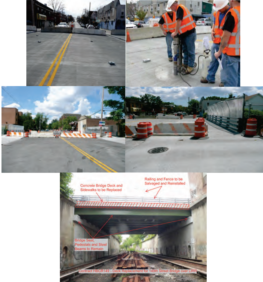
2014: Monitoring the Deck With Sensors. Taking Core Samples for Testing. Bridge is Closed to Traffic but Reopened for Pedestrians in June 2012.
