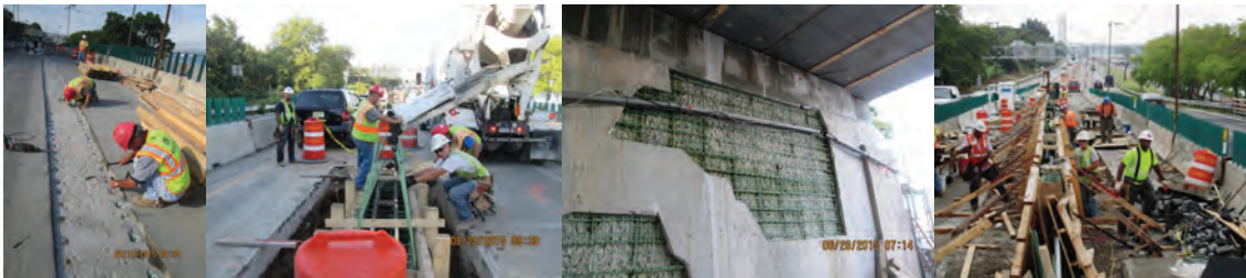
August 2015: Stage V Preparing Bridge Deck for Placement of Final Median Barrier. Placing Concrete for Final Median Barrier During Stage V - Facing East at East Approach. Epoxy Coated Reinforcing Mesh at Future Abutment Wall Repair. September 2015: Forming Operations at Final Median Barrier at East End of Bridge - Facing East.
