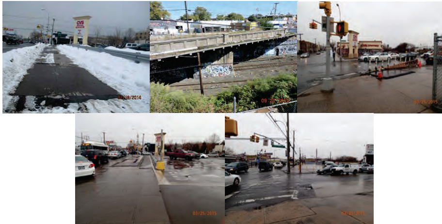
February 2014: View of Plates on Left Sidewalk (Fresh Pond Road). September 2014: Spans 1 and 2 Right Concrete Parapet. (Parapet Credit: NYSDOT) March 2015: Looking West, South, and East Across Bridge Deck.
