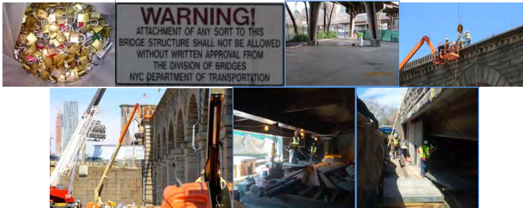
April 2015: Division Crews Removed another 450 (75 pounds) of "Love Locks" in One Day. The Locks Pose a Danger to the Infrastructure and the Cars on the Brooklyn Bridge - 9,363 Locks Were Removed From January 1 to September 25 in 2015. (Warning Sign Credit: Eugene Parker). Cleaning at Drumgoole Park. Working on the Stone Balustrade at Arch Block II. After Removing it in Sections, the Granite was Either Repaired and Reinstalled or Replaced With Completely New Granite. Sand Street Structure Curtain Wall Installation.
