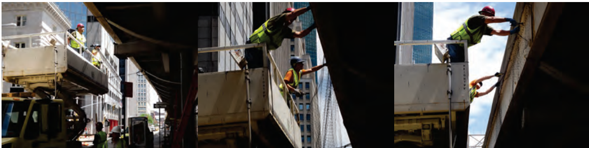
Installing Pigeon Netting at Old Slip (FDR Drive at the South Street Viaduct) in June 2012: Carpenters Stephen Buckley, William Sic, and Joseph Moschella, and Supervisor Carpenter Joseph Vaccaro. (Credit: Thomas Whitehouse)
