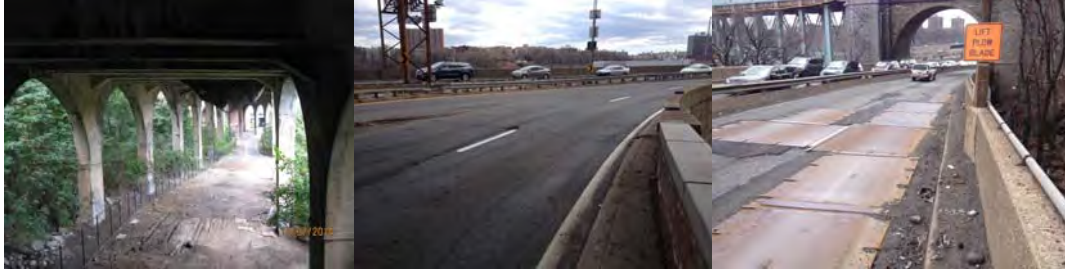
Span 42, Netting at Deck Underside, Looking Ahead. (Credit: NYSDOT) March 2015 Field Inspection.
