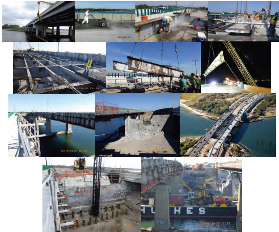
August 2015: Parapet Coating Operation at Westbound Bridge. Applying Sealing Compound to the Westbound Bridge Deck Prior to the Stage 2 Traffic Shift. Saw Cutting Deck of Bridge Prior to Removal. September 2015: Removing Saw-Cut Deck Panels. Deck Removed Prior to Steel Removal. Removing Stringers. October 2015: Removing Girder Over the Westbound Roadway With a Crane Mounted on a Barge on the North Side of the Bridge. Bridge After Removal of Steel Superstructure From North Side of Existing Bridge. South Half of Old Bridge at Right - Facing East. Partially Demolished Pier - Facing East. New Westbound Bridge at Left, Old East Bound Bridge at Right. Stage 2 Traffic Pattern. Westbound Traffic at Right on New Bridge. Eastbound Traffic at Left on Existing Bridge. December 2015: Driving 14-Inch Diameter Steel Shell Piles at East Abutment - Facing East. Barge-Mounted Hoe-Rams Demolishing Old Piers – Facing East.
