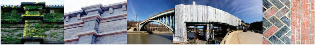
Masonry Arch Before and After Cleaning. Scaffolding and Containment. New Brick Pavers. (Credit: A.A. Mallick - NYCDDC)
