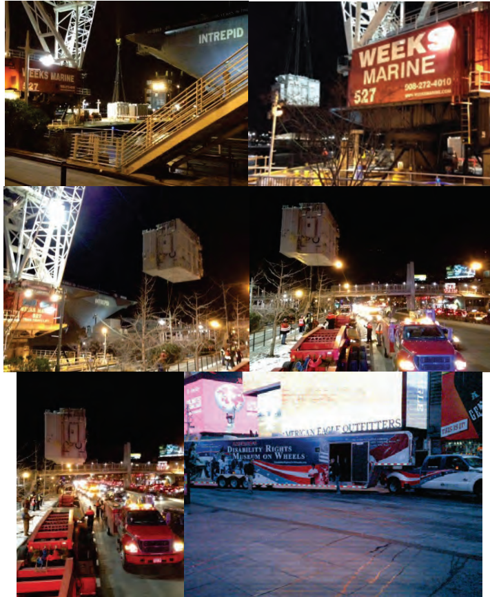
January 2015: Consolidated Edison Super Move. Shutting Down the West Side Highway on a Saturday Night to Unload a Transformer From a Barge Crane on the Hudson River (Over the Linear Park) to a Waiting Super-Load Trailer Sitting on the West Side Highway. (Credit: Scott Davis – Peak Engineering) Times Square in October 2015: 48-Foot Long Interactive Traveling Museum Touring America, the “Disability Rights Museum on Wheels” Tells the Story of the Fight for Equal Rights by People with Disabilities in the United States.
