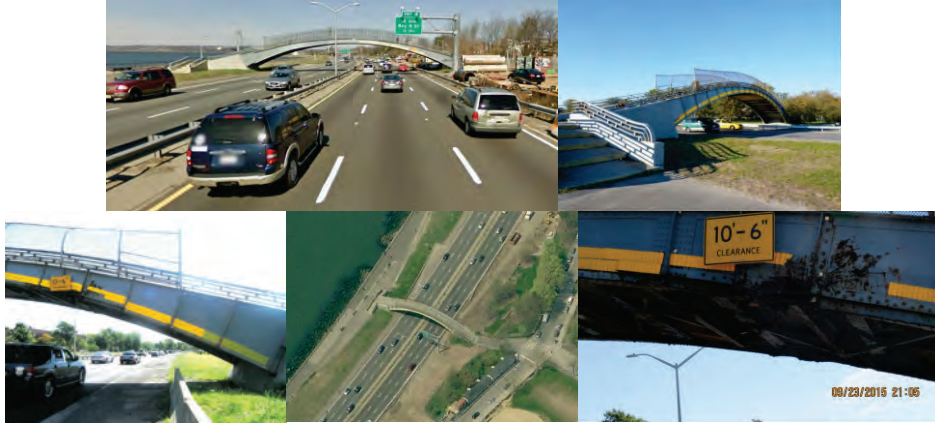
17 th Avenue Bridge – Existing Conditions. Deteriorated Left Girder. Span 1 Left Girder over Belt Pkwy Eastbound Left Lane was Hit in September 2015.
