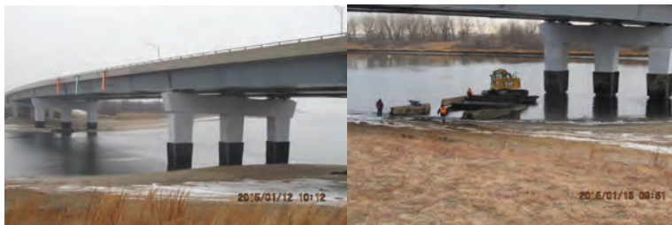
January 2015: Paerdegat Basin Bridges. Eastbound Belt Parkway Bridge over Paerdegat Basin. Newly installed Pier Bumpers at Low tide Facing East. Navigation Lights Over Center of Channel. Barge-Mounted Back Hoe used to Complete Installation of Pier Bumpers.
