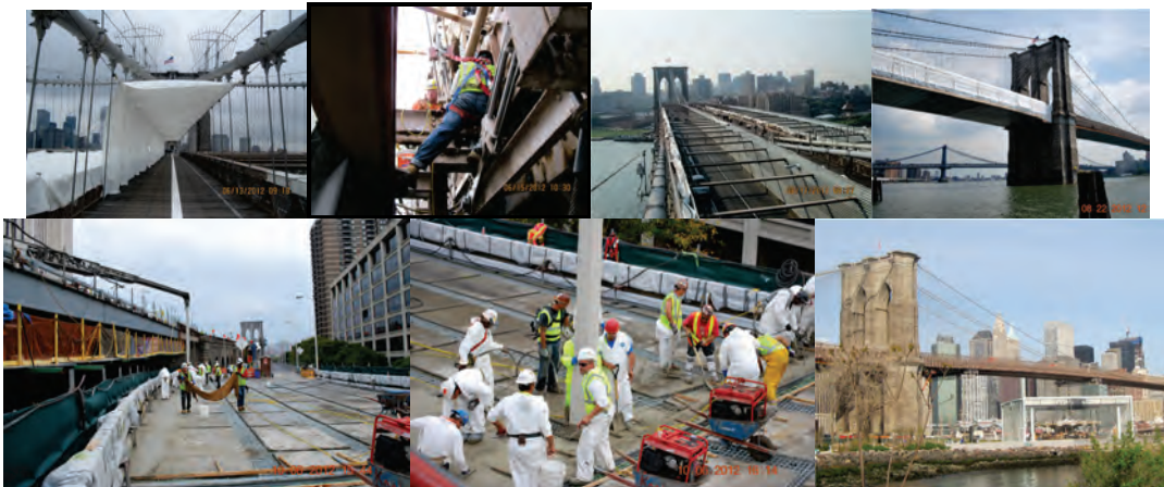
June 2012: Brooklyn Side Span Netting Protection for Main Cable and Suspender Rope Painting. June 2012: Structural Steel Repairs. 2012: Manhattan Main Span Vertical Wall. August 2012: Manhattan Side Span Containment at Manhattan Tower. First Full Roadway Closure: Ramp A Concrete Placement. Second Full Roadway Closure: Brooklyn Approach. December 2012: Brooklyn Main Span in Finish Coat.
