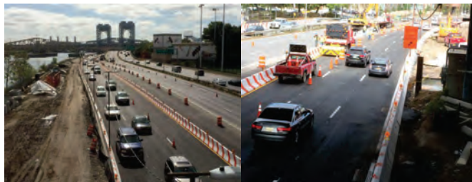
On October 5, the Temporary Roadway was Opened on the Northbound Harlem River Drive. This will enable the Start of Construction of the New 2 nd Avenue Exit Ramp.
