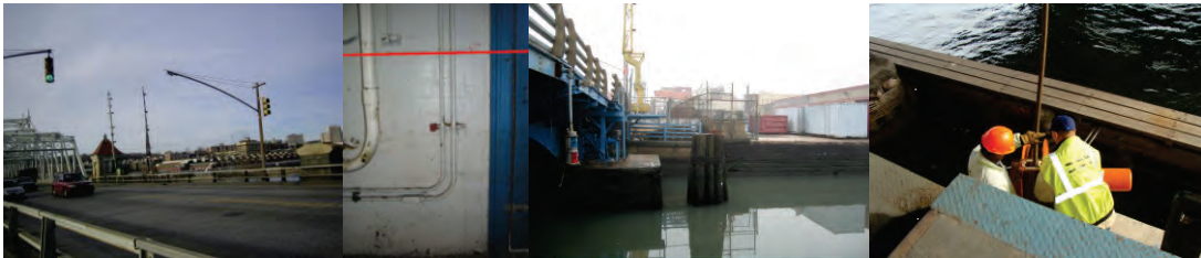
Inspection in Late 2012: East End of the West 207 th Street Bridge - Missing Traffic Signal was Knocked Down by the Hurricane Winds. Borden Avenue Bridge Operator's House Basement Level - Depicted Flood Line was Approximately 5 Feet Above the Floor. Third Street Bridge - Northwest Channel Light Missing. Ninth Street Bridge - Manually Pulling the Cable Reel Because the Motor Failed.
