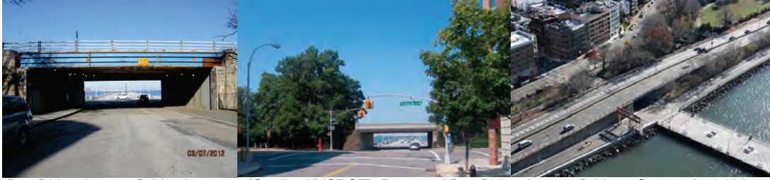
Bay Ridge Avenue Bridge in 2012. (Credit: NYSDOT) Proposed Bay Ridge Avenue Bridge. Current Aerial View.
