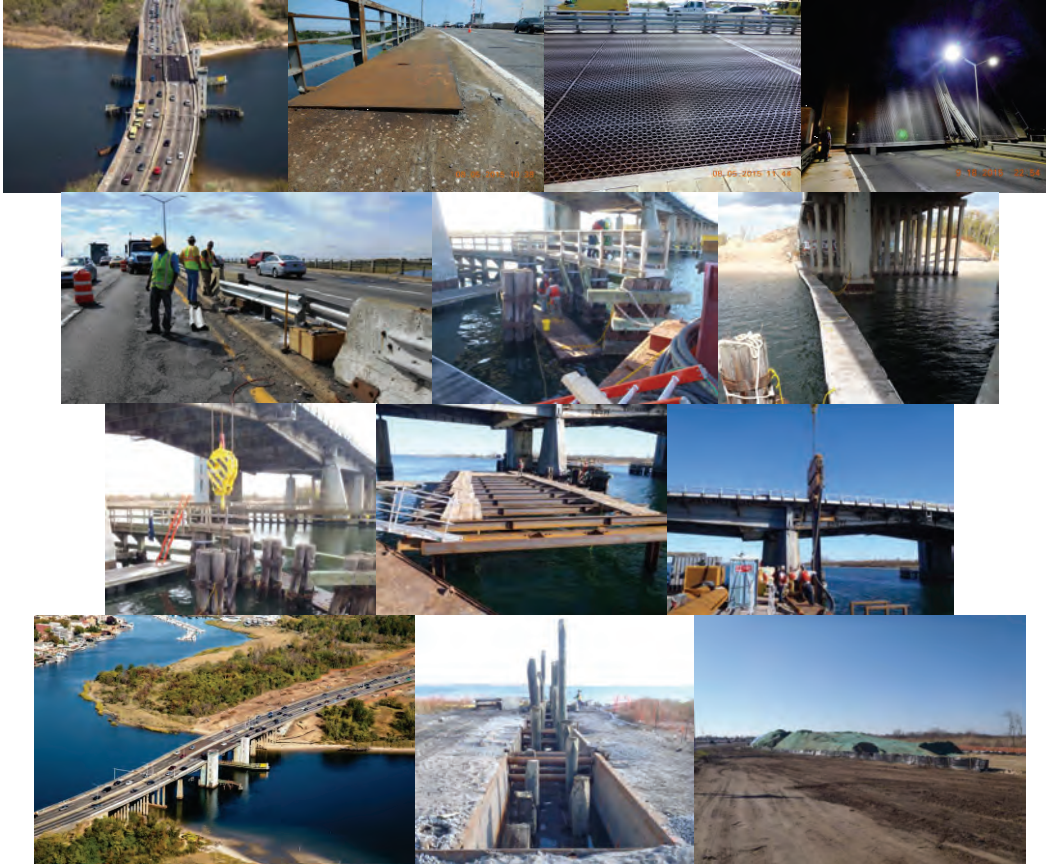
July 2015: Eastbound Traffic on Right. Westbound Traffic at Left. August 2015: Span 3, Top of Deck, Westbound (Left) Sidewalk. Span 8, Top of Deck, Steel Grating Side. September 2015: Bascule Span Fully Lifted. Median Guide Rail Repair Operations on East Side of Bridge. October 2015: Removal of Existing Fender at North Side of Pier #6. Temporary Walkway on North Side of Bridge for Access to Pier #9. November 2015: Extracting Wood Piles From the Existing Bridge Fender System at New Pier #9 Site. Pier #9 Steel Framing for the Cofferdam on the West Side of the Existing Bridge. Pier #9 – Driving “Pin Pile” for Support of the Cofferdam Steel Frame. Site After Completion of Tree Removal. December 2015: Outfall #2. Pressure Treated Wood Piles – Facing East. Hydroseeded Topsoil Stockpile to Prevent Erosion at Southwest Quadrant, Protected by a Silt Fence.
