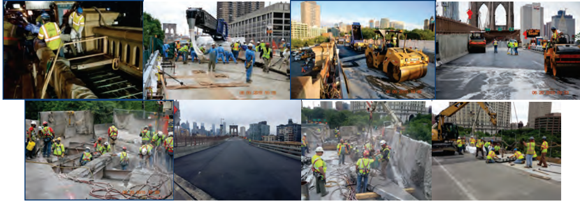
May 2015: Brooklyn Arch Blocks Steel-Faced Curb. June 2015: Division Quality Assurance Personnel Observe Closure Pour Concrete Placement at Westbound Park Row Structure. Asphalt Paving of Brooklyn Approach. Division Quality Assurance Personnel Observe Testing on the Newly-Applied Asphalt Overlay at the Westbound Brooklyn Approach. Manhattan-Bound Approach North Cantilever. Paving of the Manhattan-Bound Brooklyn Approach, Demolition at Ramp D in Manhattan, and Super Slab Installation During the Full Weekend Closure in June.
