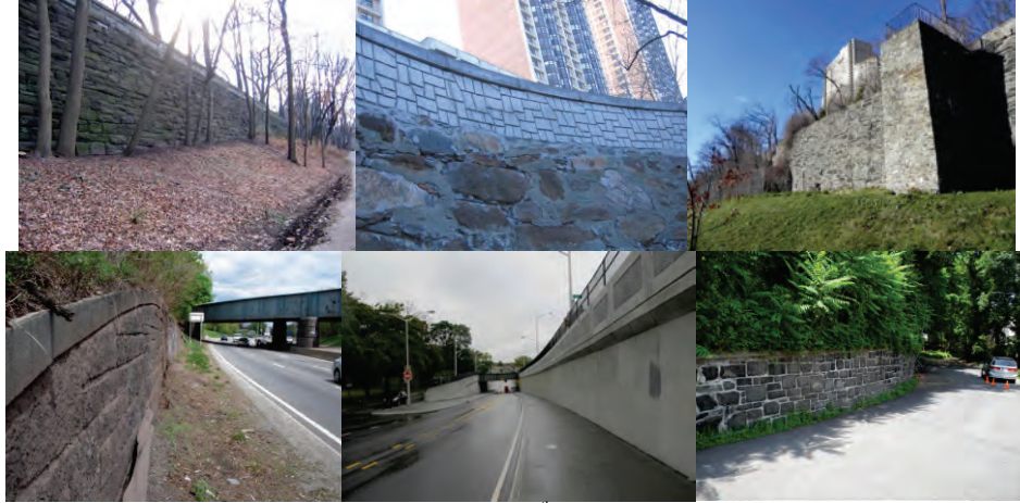
Retaining Walls: Southeast Corner of West 108 th Street and Riverside Drive. Left Side of Ramp From Riverside Drive to George Washington Bridge. Irwin Avenue. Cross Island Parkway Southbound Before 100 th Avenue. Cooper Avenue. Douglas Road.
