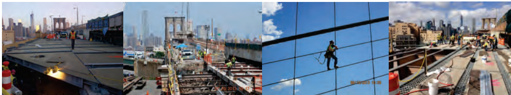
April 2013: Installation of Temporary Deck Units at the York Street Structure Over Brooklyn-Queens Expressway. July 2013: Removal of the Existing Concrete Slab on the Eastbound Main Street Structure. August 2013: Ironworker Replacing Cable Clamp Assemblies on the Suspended Span. October 2013: Grid Deck Panel Installation at the Eastbound Park Row Structure.
