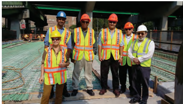
September 2015: Inspecting the Preparations for the Bridge Deck Concrete Pour at the Bryant Avenue Bridge over AMTRAK and CSXT. Assistant Civil Engineer Evgenia Campbell, Assistant Electrical Engineer Satpaul Jaswal, Director of In-House Design Ferdinand John, and Civil Engineers Kirolos Dimian, Kamran Sikandar, and Lev Gold. (Credit: Ludner Charles)
