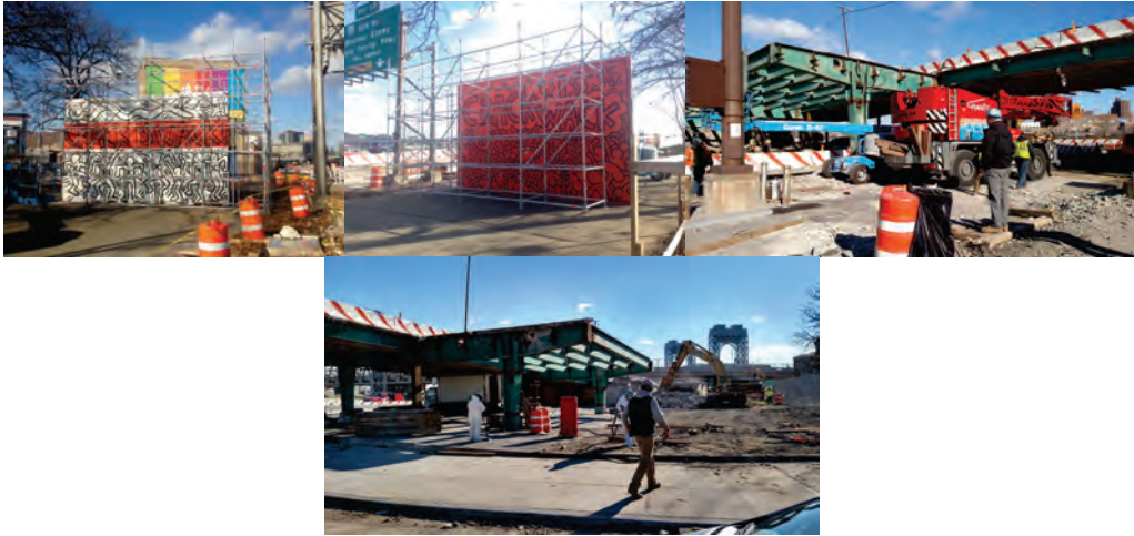
Starting the “Crack is Wack” Protective Scaffolding. Stage 2: Demolition of the Existing Southbound Structure. (Demolition Credit: Richard Solomon)
