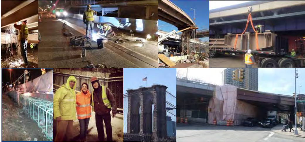
January 2015: Welding on the Bridge above Pearl Street (Franklin Square Structure). Replacing the First Column Supporting the Exit Ramp From the Northbound FDR Drive. Ramp C Steel Column Erection. Cast-in-Place Concrete Barrier Installation. Commissioner Polly Trottenberg Visited the Summit Street Pedestrian Overpass to Thank Division Staff for Clearing the Snow and De-icing the Walkway. March 2015: New Flag. April 2015: Containment System at Prospect Street.
