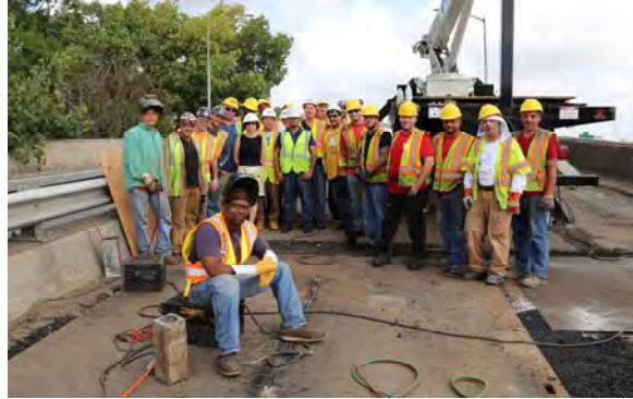
On September 29, 2015, Division Personnel Conducted Emergency Repairs on Two Punch-Through Locations on the Top of the Deck. Steel Plates Were Installed. The Repairs Were Then Added to the Contractor's Work Scope. From Left: Bridge Repairer and Riveters Charlie Zhao and Ignazio Trapani, Carpenter Gregory Nolan, Supervisor Bricklayer Edward Alfano, Cement Mason Luigi Mula, Commissioner Polly Trottenberg, Assistant Civil Engineer Andrew Hoang, Carpenter Edward Alfano Jr., Assistant Civil Engineer Fouad Althaibani, Area Supervisor Highway Maintenance Edward Pedersen, Supervisor Highway Repairer Andrew Bondi, Supervisor Carpenter Joseph Diblasi, Bridge Repairer and Riveter David Fontanez, Assistant City Highway Repairers James Cummings, Anthony Connelly, and James Kelleher, Bricklayer Stephen Daniel, and Cement Masons Victor Porowski and Frank Finzio. Foreground: Bridge Repairer and Riveter Chris Mauldin.
