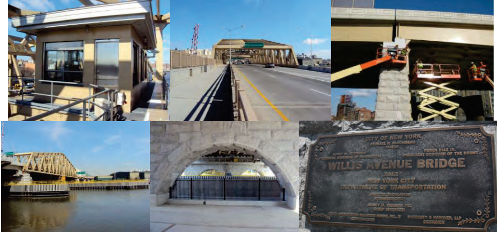
February 2013: Bridge Operator House. General View Taken From the West Side – Looking East. Pier 11- Continued installation of granite stone retrofit anchors. March 2013: Fenders of the River Piers. Pier 4 Picket Fence. Willis Avenue Bridge Plaque.
