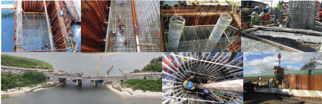
March 2014: Setting Footing Rebars Prior to Placing Pier Rebars and Concrete at Pier No. 2. April 2014: Setting Rebars for Footing and Pier Inside Cofferdam at Pier #1. May 2014: Plinth and Column Reinforcement Inside the Cofferdam for Pier 2. June 2014: Placing and Vibrating Concrete for Plinth at Pier #1. Rebars for Column in Place. West Abutment of Bridge. New Roadway Under Construction at top Next to Westbound Lanes. East Abutment of Bridge. Crane on Barge at Cofferdam for New Pier #2. August 2014: Workers Inside Rebar Cage During Operation of Pumping Concrete Into Pier #2 Column. November 2014: Steel Sheeting in Place for the East Approach Temporary Access Roadway.
