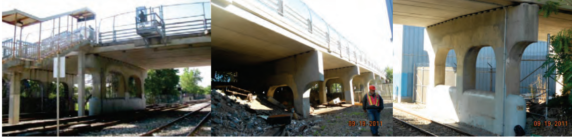
Hannah Street Bridge Over SIRT South Shore. Spans 1-4 - Right Elevation. Pier 3. (Span and Pier Credit: NYSDOT)
