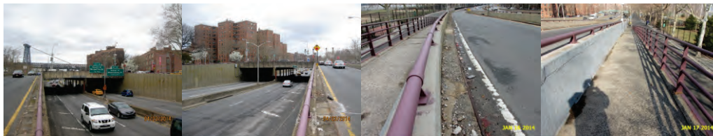
The Three Structures of the FDR Drive at Houston Street Overpass. 2014: Main Bridge – Left and Right Elevations. South Approach Ramp - Span 2, Left Side Safety Walk and Curb. North Approach Ramp - Span 2, Top of Cantilevered Pedestrian Walkway. (Credit: NYSDOT)
