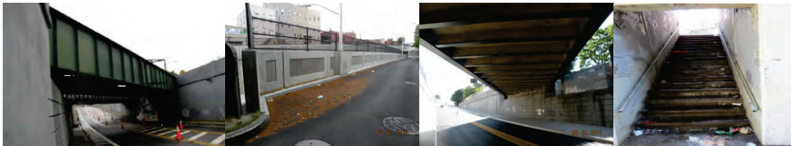
71 st Avenue Bridge over Cooper Avenue. Left Concrete Parapet/Guide Rail. Span 1 Bridge Framing. (Parapet and Span Credit: NYSDOT) Stairway at Right Side of Beginning Abutment.
