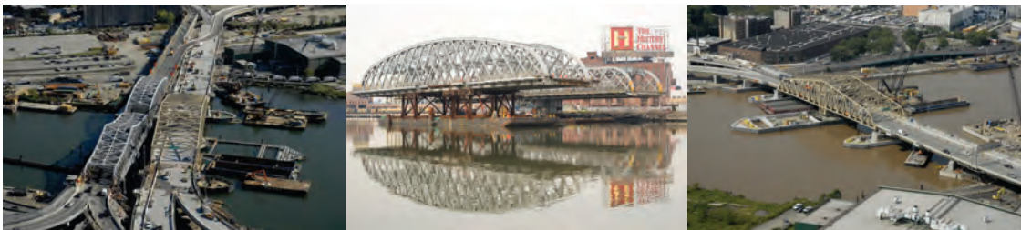
New and Old Willis Avenue Bridges on October 2, 2010. Old Willis Avenue Spans in December 2010. (Credit: Duane Bailey-Castro) Aerial View in September 2011. (Credit: Hardesty and Hanover)
