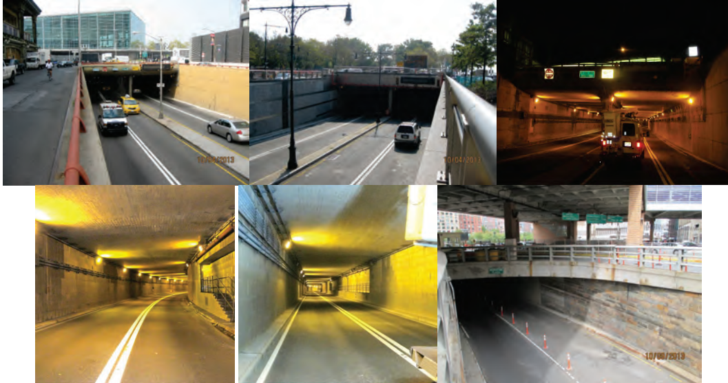
October 2013 – Battery Park Underpass – Elevation Right Span 1 and Left Span 1. (Credit: NYSDOT) September 2013 - Span 2 Looking Westbound (FDR Drive to West Street). June 2014 – The Underside of the Tunnel is Completely Covered With Tiles. October 2013 - West Street Underpass - Elevation Right Span. (Credit: NYSDOT)
