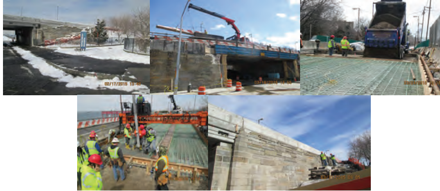
February 2015: Northwest Abutment and Wingwall Prior to Stonework Restoration. March 2015: Installation of Temporary Concrete Barrier on Eastbound Bridge in Response to a Red Structural Flag. Dumping Sub Base Soil for East Approach Deck. Placing and Finishing the Deck Wearing Surface for the Stage III Concrete Deck. Workers Resetting the Stone Facing on the Northwest Abutment and Retaining Wall.
