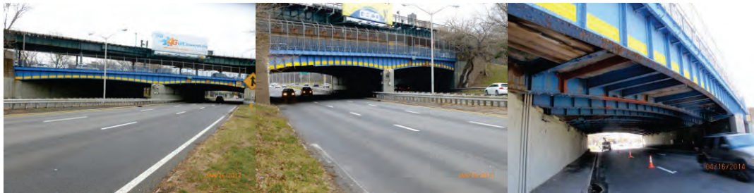
Westchester Avenue Bridge Elevation Left and Right in 2012. (Credit: NYSDOT) April 2014: Span 2 – Deteriorated Areas Shielded With Planks.
