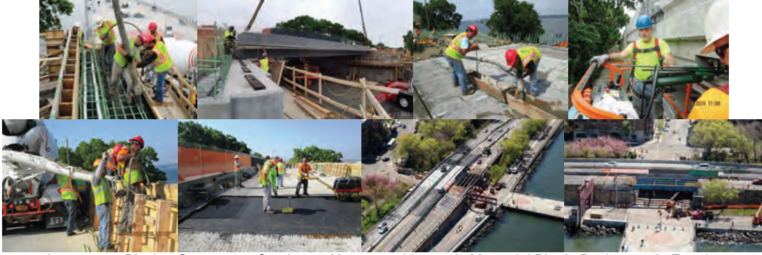
June 2015: Placing Concrete at Southeast Abutment - Veteran's Memorial Pier in Background. Erecting Precast Prestressed Concrete Beams at South Side of the Bridge Onto Elastomeric Bearing Pads. Placing Grout Between Recently Placed Precast Prestressed Beams - Facing Southeast. July 2015: Final Post-Tensioning of Precast Concrete Deck Beams From the North Fascia of the Bridge. Placing and Vibrating Concrete for the Parapet on the Eastbound Bridge. Compaction Testing of the Asphalt Pressure Relief Joint at the West Side of the Eastbound Roadway. Stage IV Existing Eastbound Bridge Deck Removed. Eastbound and Westbound Traffic on New Pre-Cast Pre-Stressed Beams. Westbound Traffic at Left. Veterans Pier at Right. Shore Road at Left. Stage IV - Preparing to Remove the Structural Steel From the South Side of the Existing Bridge.
