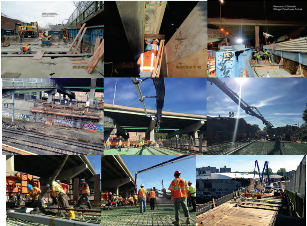
March 2015: Chipping Out Roadway Deck Concrete and Removing Shielding Concrete. May 2015: Installing Overhang Brackets on South Side of Pedestrian Walkway. Removal of Sidewalk Stringer Panel. Summer 2015: Existing Structure Removed. September 2015: Placing the Concrete for the Bridge Deck. The Concrete Pump Placed 110 Cubic Yards of Concrete Into the Deck. Covering and Protecting the Fresh Concrete with Wet Burlap.
