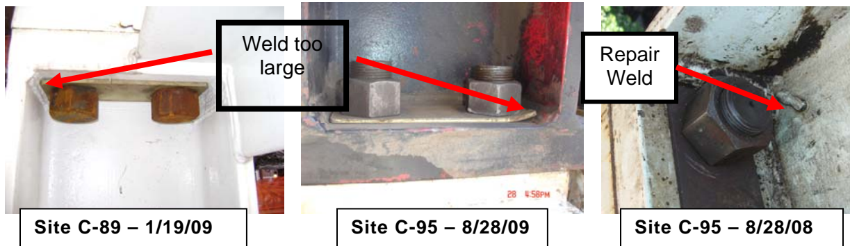
Figure C.10.5: Poor repair welds
