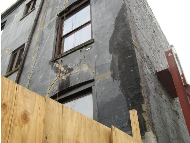
Figure D.10.3: Extensive structural cracking of upper stories with superficial repair
