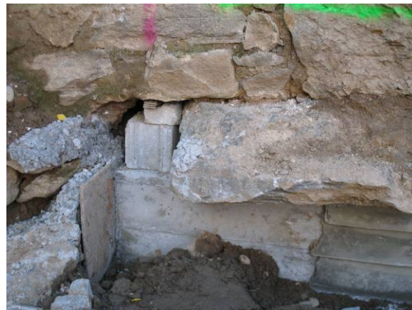
Figure D.14.7: Inadequate repair and shimming
