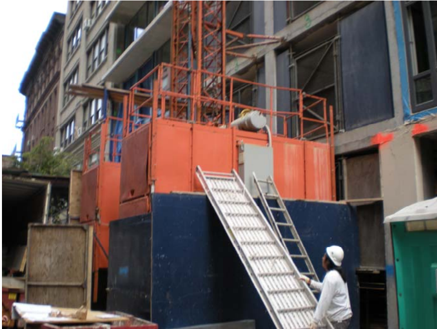
Figure C.8.17: Improper use of hoist car to transport material.
