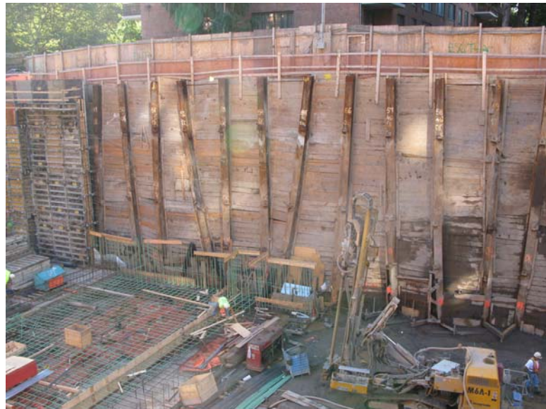
Figure D.16.2: Soldier pile and lagging with 2 layers of tiebacks supporting a 40-ft excavation
