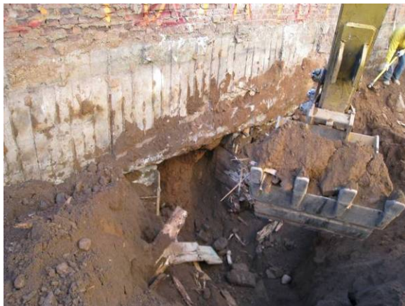
Figure D.14.6: Improper pit excavation
