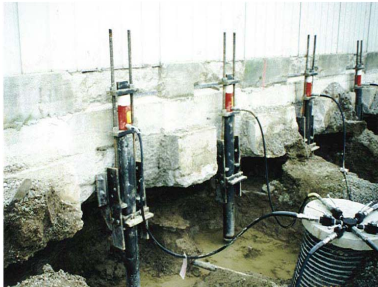
Figure D.16.8: Manifold jacking of push piles to underpin a bearing wall (Reproduced from Atlas Systems Technical Guide for Underpinning Settled Structures, 2003)
