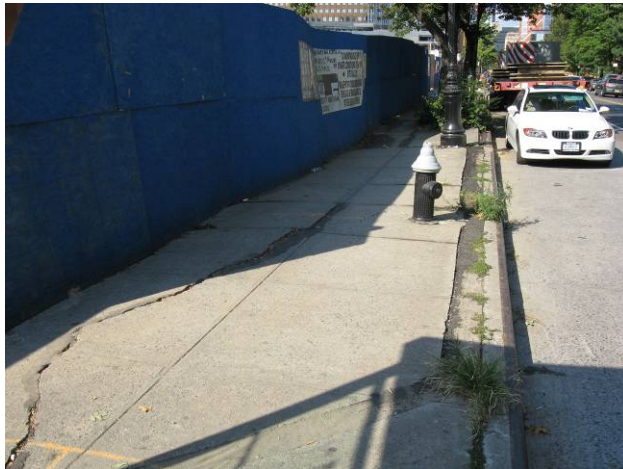
Figure D.10.5: Sidewalk cracking and subsidence extending to the curbline
