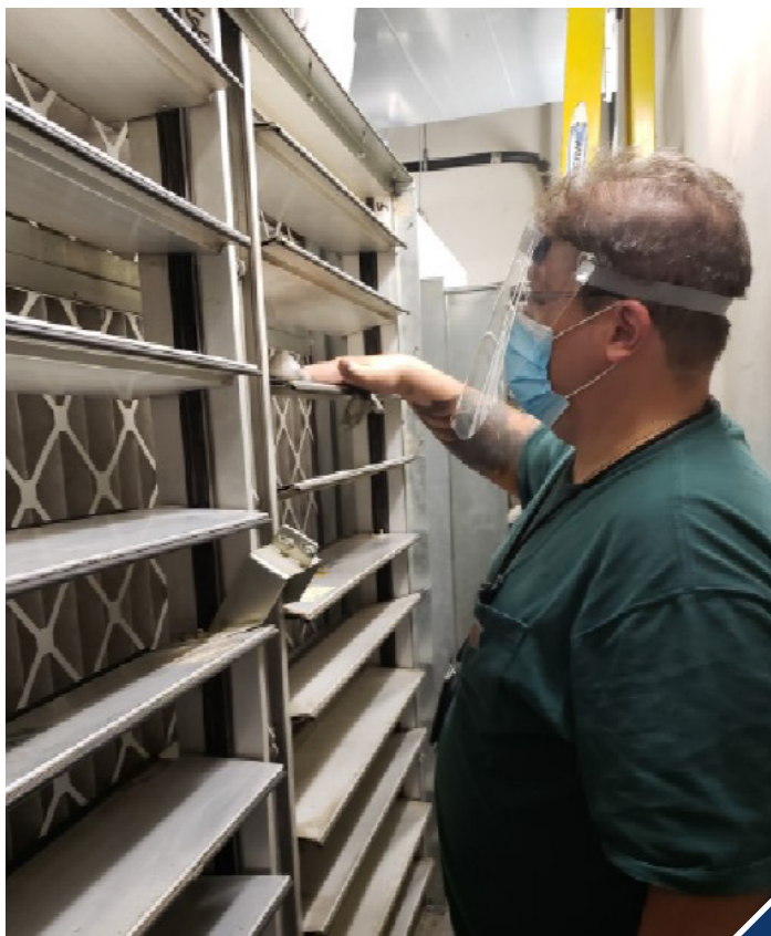
DCAS staff member Robert Valdes working on our air handling systems.
