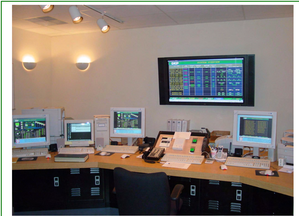
Figure 2.6 SCADA System control room depicting water supply status for water quantity and quality.
