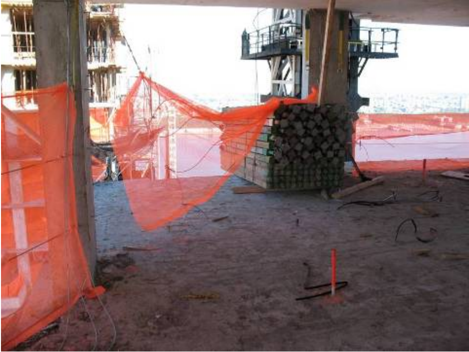
Figure B.7.19: Current Code-Compliant Material Storage Practice (Piled Material is Banded and Braced) and Accompanying Fall Hazard at Unprotected Edge (Left)
