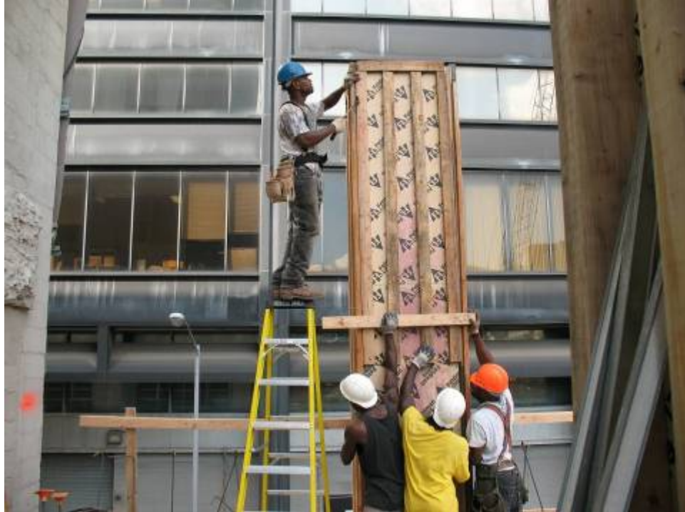
Figure B.8.7: Initial Failure to Tie-off at Site No. 86, 3-Sept. 2008 (OSHA Violation)
