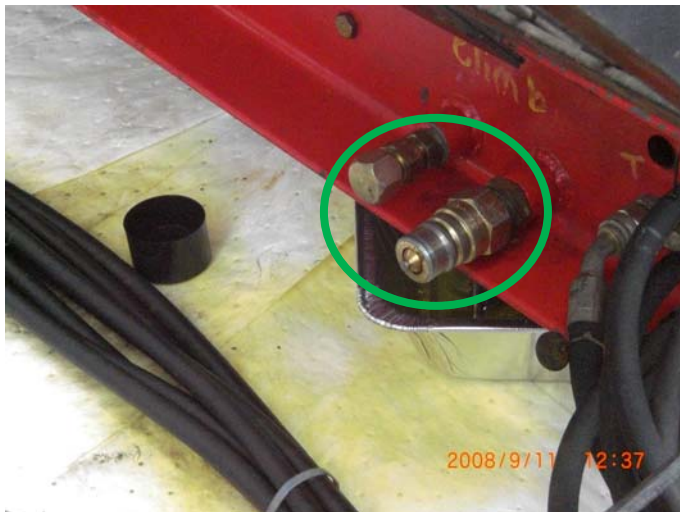
Figure C.6.9: Leaking Hydraulic Fitting
