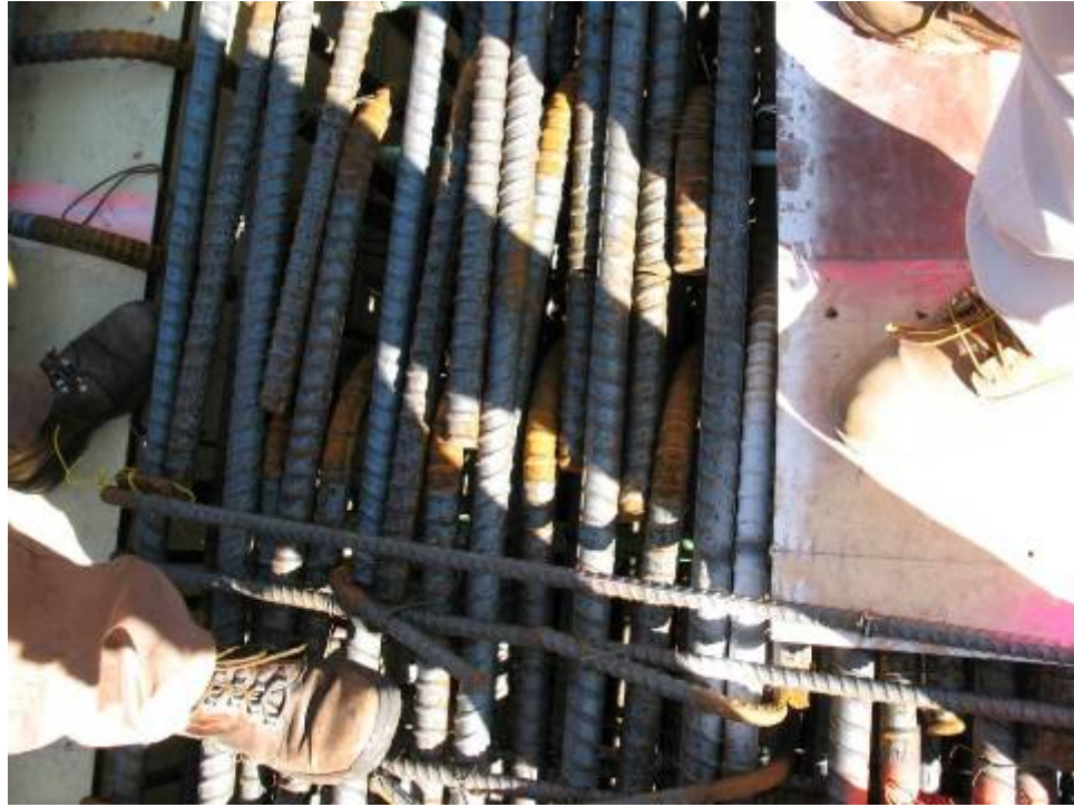
Figure B.10.2: Constructability Issues at Beam-Column Connection
