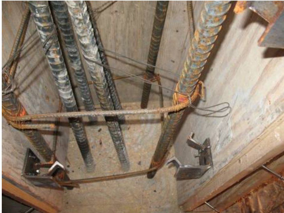
Figure B.10.1: Splice Condition Requiring Additional Information from the Engineer of Record.
