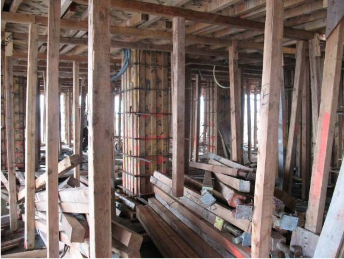
Figure B.7.2: Unacceptable Debris Accumulation and Material Storage during Formwork Operations. Lack of Storage Space Concentrates Material within Work Areas, Impeding Egress Pathways. Note Shoring Post (Center) Stopped Short of Floor over Stacked Material.
