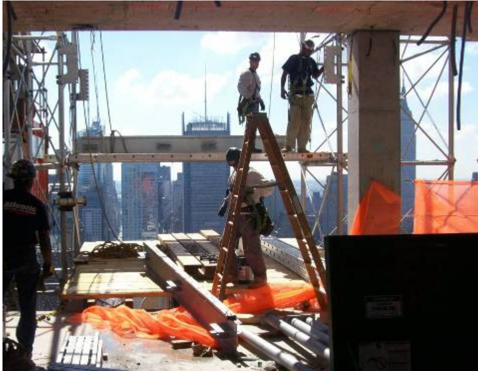
Figure B.7.12: Failure to Tie-off within 10 feet of Unprotected Edge
