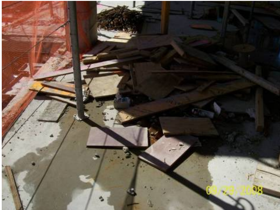
Figure B.7.9: Unacceptable Level of Debris Accumulation. Enforcement Level: Violation
