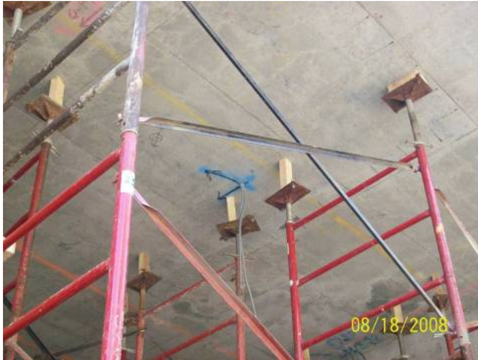
Figure B.6.2: Formwork Construction Not in Conformance with Design, Unstable Timber Posts used as Filler between Steel Shoring Tower and Concrete Soffit
