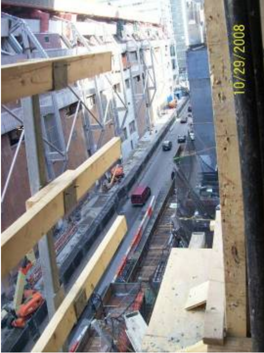
Figure B.7.4: Localized Gap Condition at Guardrail. Lack of Specificity Regarding Allowable Gap Distance (if any) Forces Inspector to Make a Potentially Inconsistent Judgment Call
