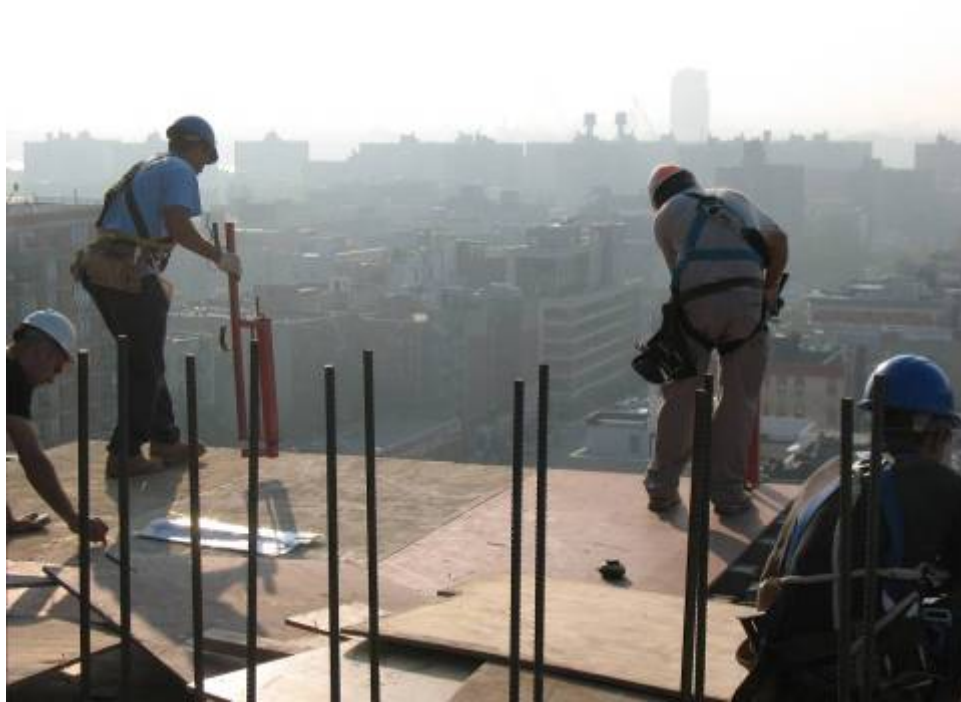
Figure B.8.1: Failure to Tie-off During Decking Operations. Retractable Lanyards Could Have Been Utilized, Anchoring to Formwork Subassembly
