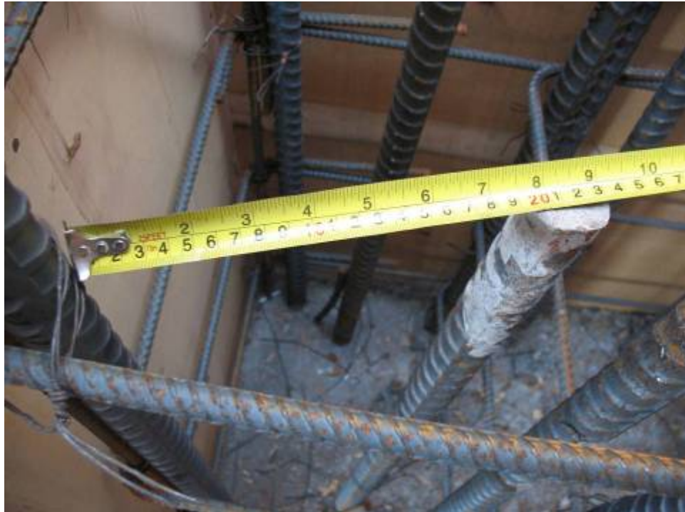
Figure B.9.1: Typical Critical Quality Defect: Column Splices Noncompliant with ACI. Conditions Subsequently Remedied to the Satisfaction of the Engineer of Record
