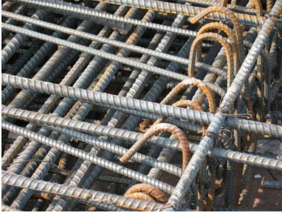
Figure B.9.6: Improperly Fabricated Shear Stirrups, Resulting in Improper Stirrup Engagement. Conditions Subsequently Remedied to the Satisfaction of the Engineer of Record
