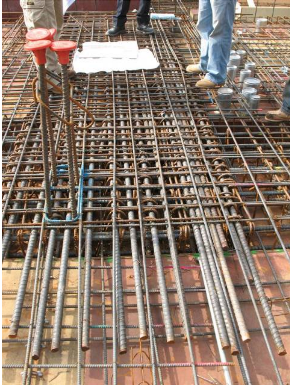
Figure B.9.13: First Floor Transfer Girder Bar Congestion. Site No. 47
