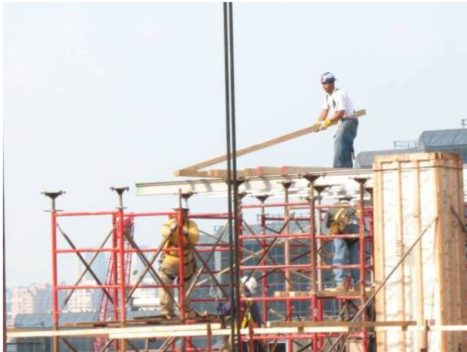
Figure B.8.6: Commonly Observed Failure to Tie-off During Formwork Erection Operations
