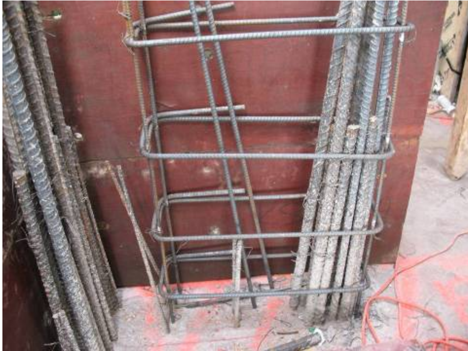
Figure B.9.9: Column Bar Congestion. Conditions Brought to the Attention of the Engineer of Record
