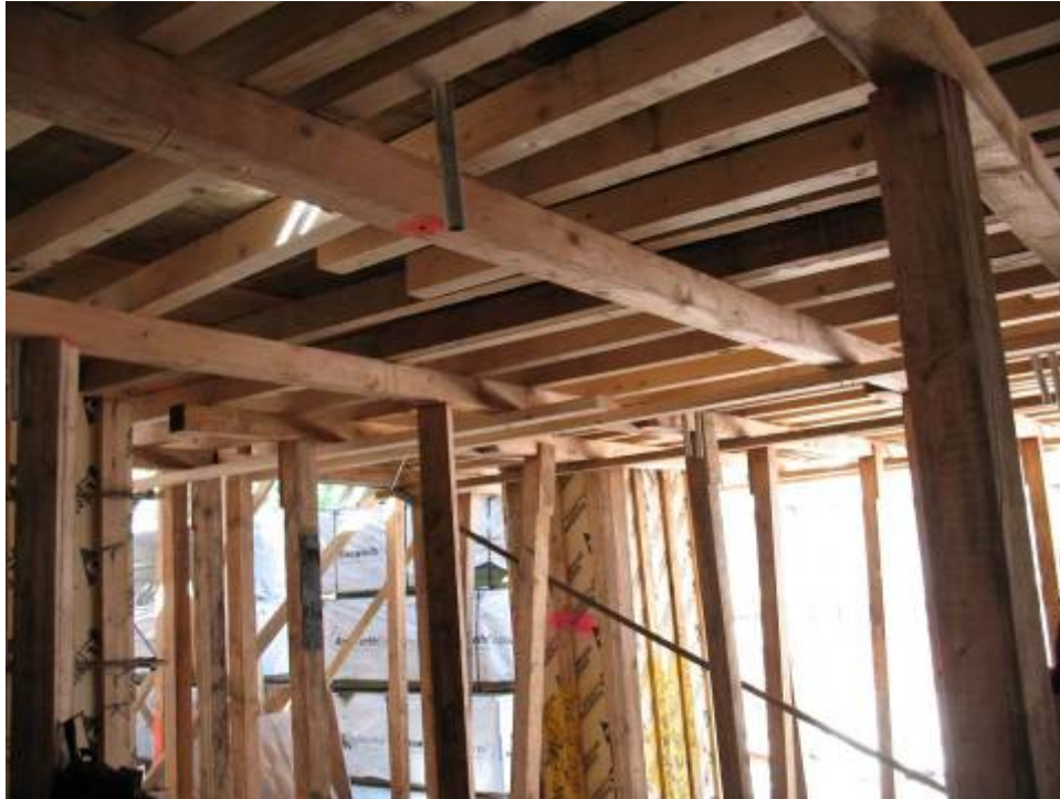
Figure B.6.5: Insufficient Post Spacing, Missing Posts at Stringer Element (Top Center)
