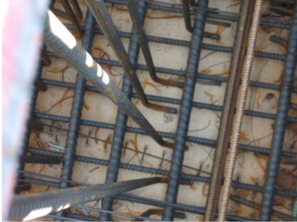
Figure B.9.3: Typical Critical Quality Defect: Improper Shear Stirrup Engagement. Conditions Subsequently Remedied to the Satisfaction of the Engineer of Record
