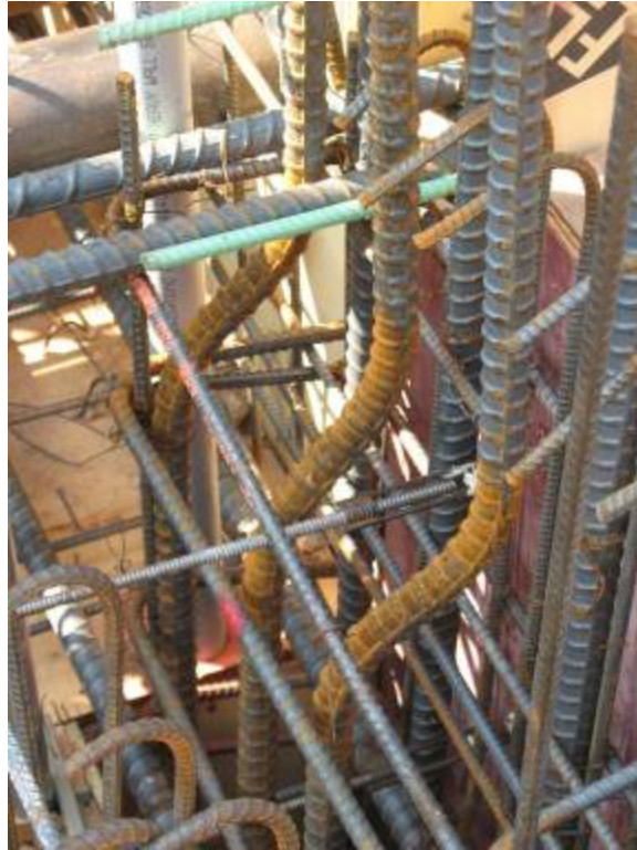
Figure B.9.7: Bar Fabrication Noncompliant with ACI 28 . Conditions Brought to the Attention of the Engineer of Record
