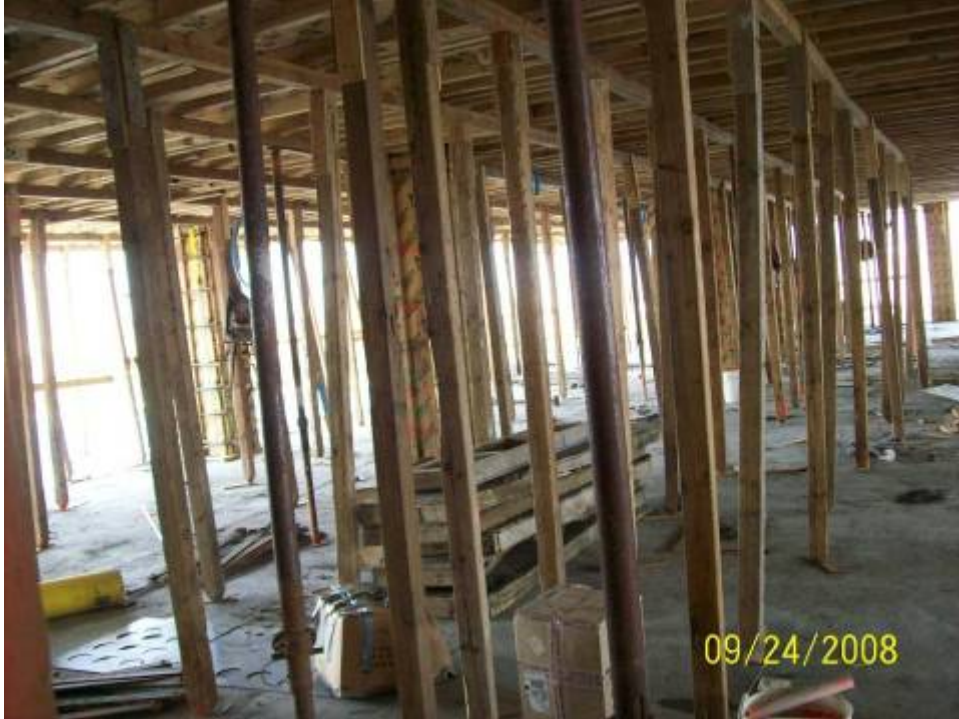
Figure B.6.1: Typical Stick Formwork Assembly consisting of Timber Posts and Lumber Framing Elements
