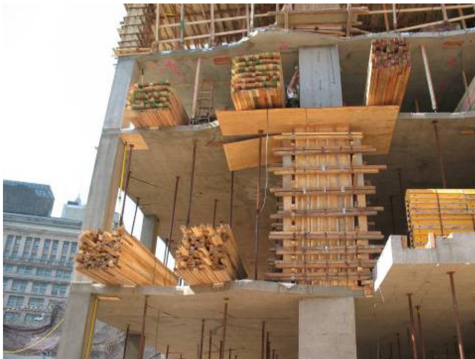
Figure B.7.18: Typical Unacceptable Lack of Edge Protection at Building Edge Coincident with Material Storage. Guardrails Removed over a Large Portion of This Building's Exposure to Accommodate Material Piles
