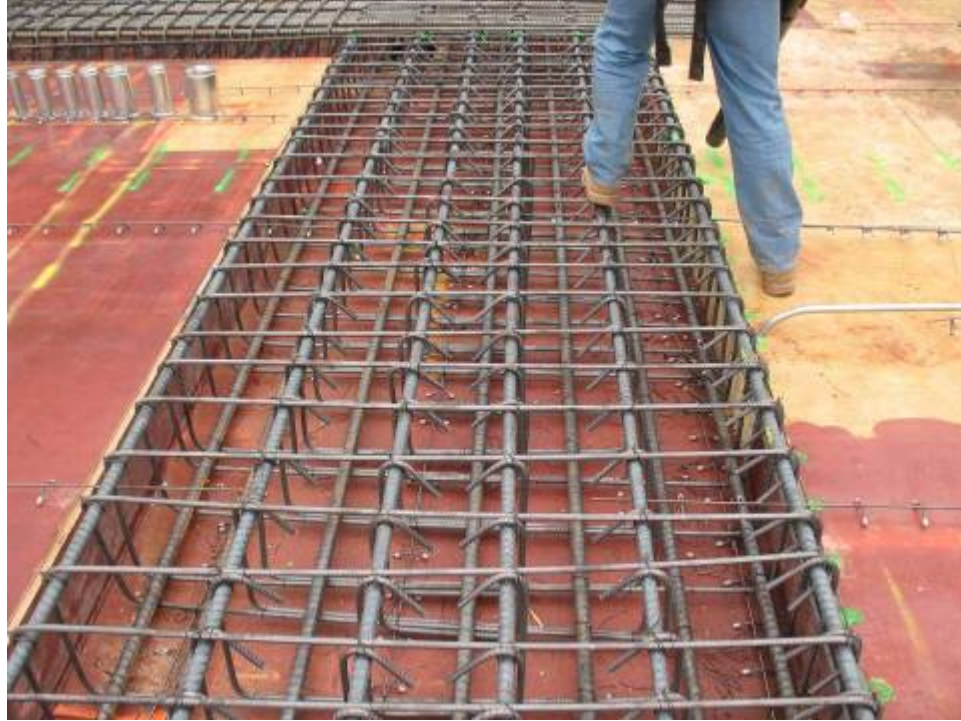
Figure B.9.12: First Floor Transfer Girder with Insufficient Numbers of Installed Shear Reinforcing Sets. Site No. 47
