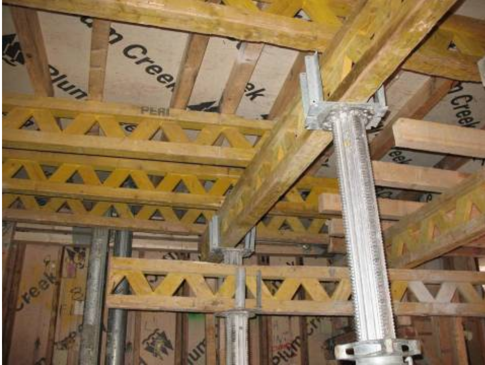
Figure B.6.8: Unstable 8 Stacked Truss-Type Stringer Assembly, Not in Conformance with Design
