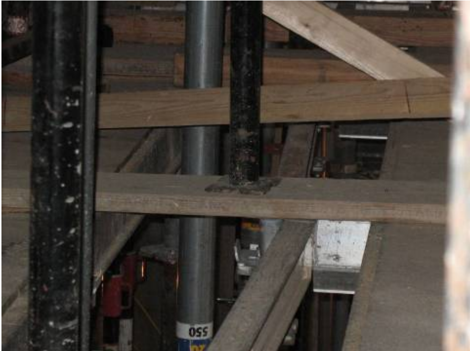
Figure B.6.10: Lack of Adequate Support under Post Base (Center), Not in Conformance with Design.
