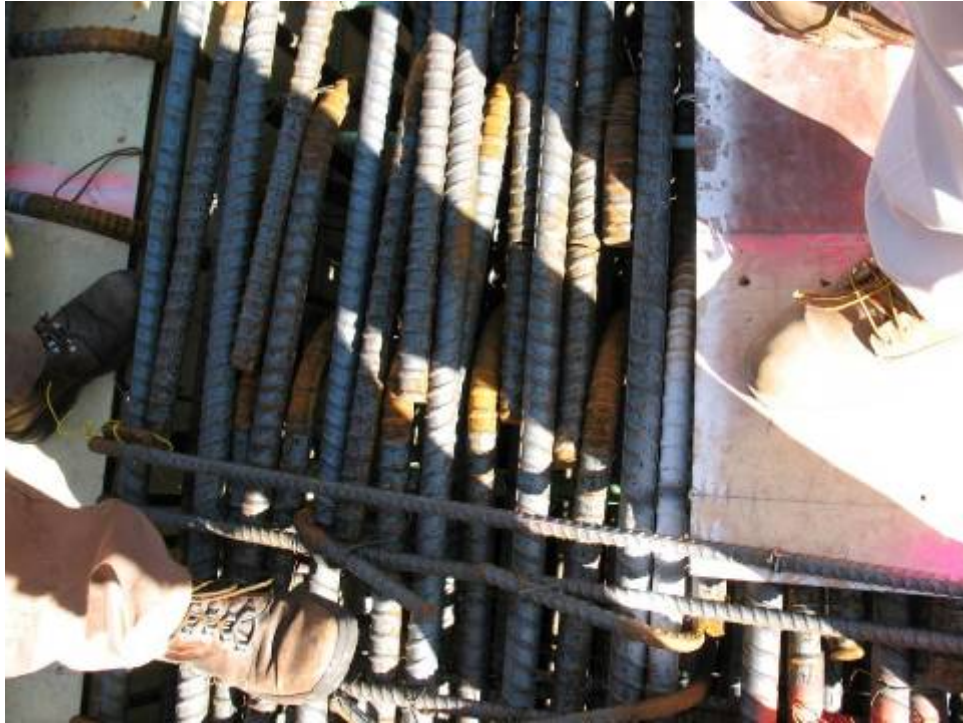
Figure B.9.10: Severe Bar Congestion 29 . Conditions Brought to the Attention of the Engineer of Record
