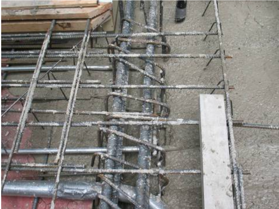
Figure B.9.8: Lack of Proper Shear Stirrup Engagement. Condition Soon to be Hidden by Concrete Encasement. Conditions Brought to the Attention of the Engineer of Record
