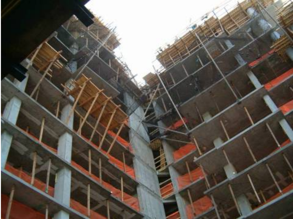
Figure B.7.6: Building Exposure with Incomplete Edge Protection. Code Provisions Do Not Address Violation Thresholds Relating to Percentage of Exposure without Protection
