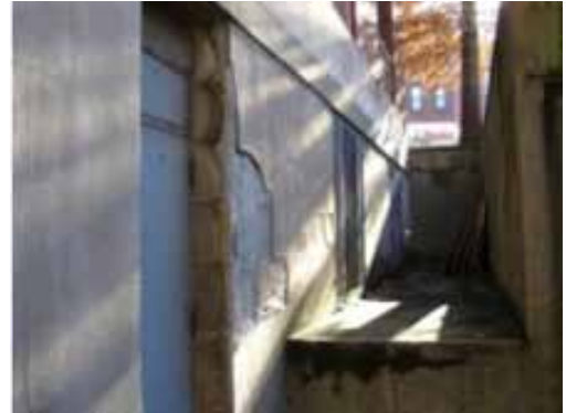
Figure 9. Basement wall of bluestone, now with deteriorated stucco covering.
