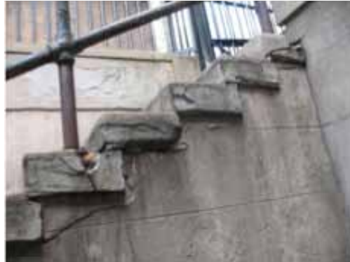
Figure 8. Example of an original parged wall, scored and pointed to resemble stone blocks. Also visible are the deteriorated bluestone steps and original pipe handrail.
