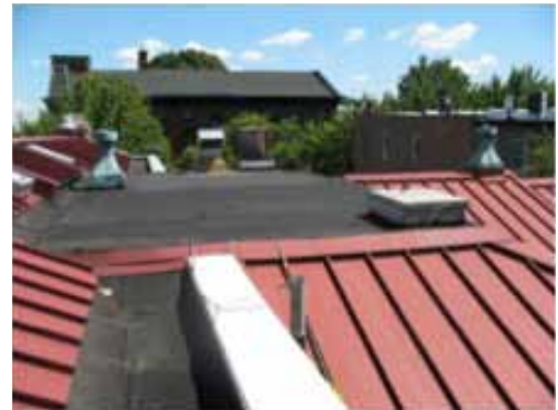
Figure 24. Typical roof conditions. The sky light over the book stacks was partly in the flat area of roll roofing and extended into the pitched roof, creating what must have been a complex sky light.
