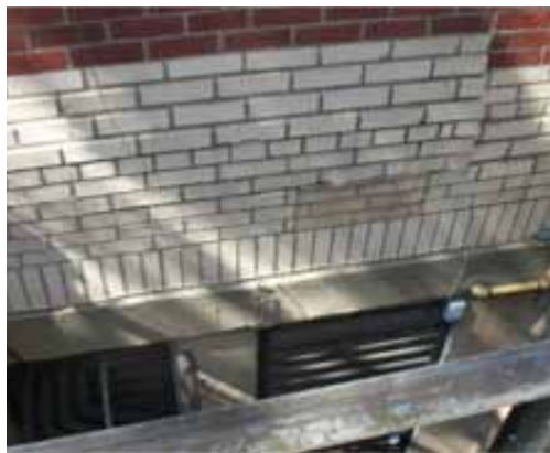
Figure 10. Originally substituted for limestone at the rear of the building to save money, the white brick is in deteriorated condition.
