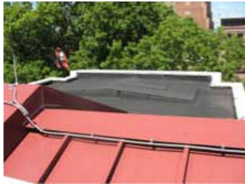
Figure 23. Looking towards the front of the building with the vestibule sky light location evident from the raised curb.
