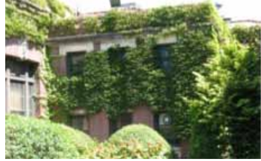
Figure 19. Rear facades from the south ca. 2012. The vines, while picturesque, are not good for the masonry and can obscure maintenance needs.
