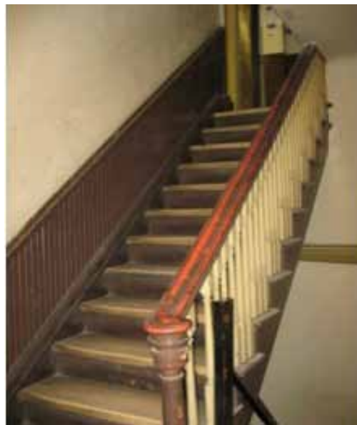
Figure 43. South staircase prior to stripping. The mirror-image stair on the opposite side of the stack area was removed in phase 1 for an elevator.
