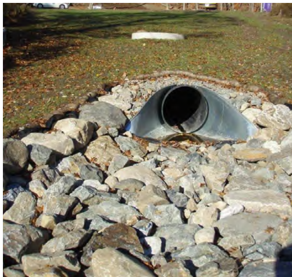
Figure 4.31. A) N7 before construction, B) installation of N7 pipeline, and C) N7 after construction.
