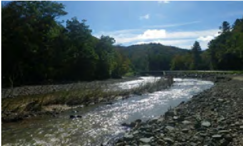
Figure 4.24. Neversink Demonstration Project, damaged by September 18, 2012 flood.
