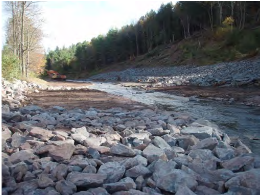
Figure 4.23. West Kill bank stabilization at NYS Route 42 following construction of the project to slow this fine sediment-laden landslide of approximately 40 acres.
