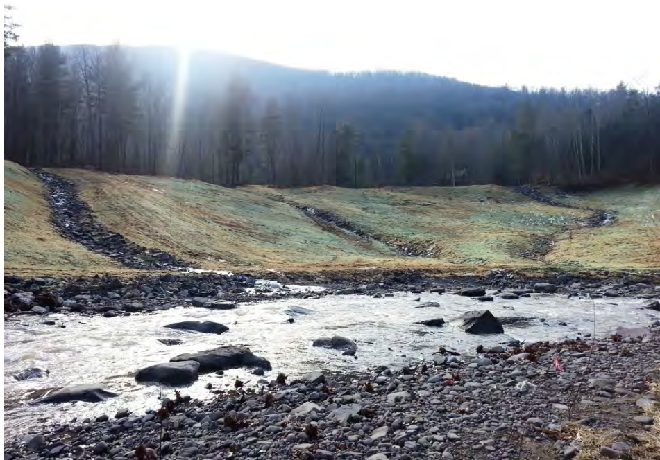
Figure 4.17. The Stony Clove Creek at Chichester reach Site 2, showing the hill slope and reconstructed stream channel that elevated the bed, stabilized the mass failure, and modified the slope drainage.
