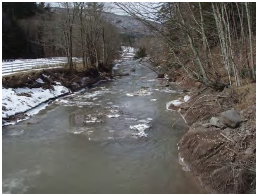
Figure 4.20. Incision into the bed causing slope failure at the West Kill bank stabilization at County Route 6 before the project was completed.
