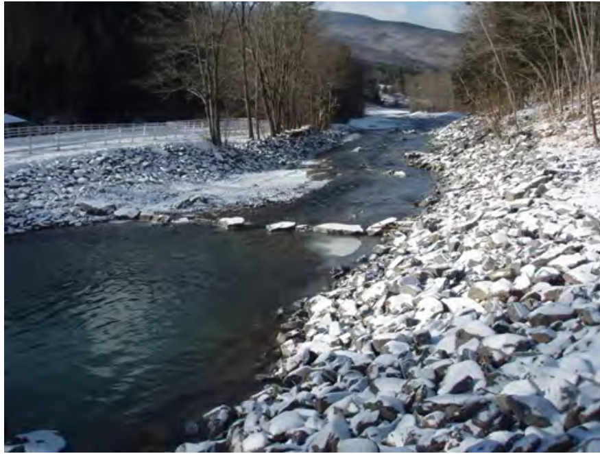
Figure 4.21. West Kill bank stabilization at County Route 6 following construction designed to stabilize the bed and banks.
