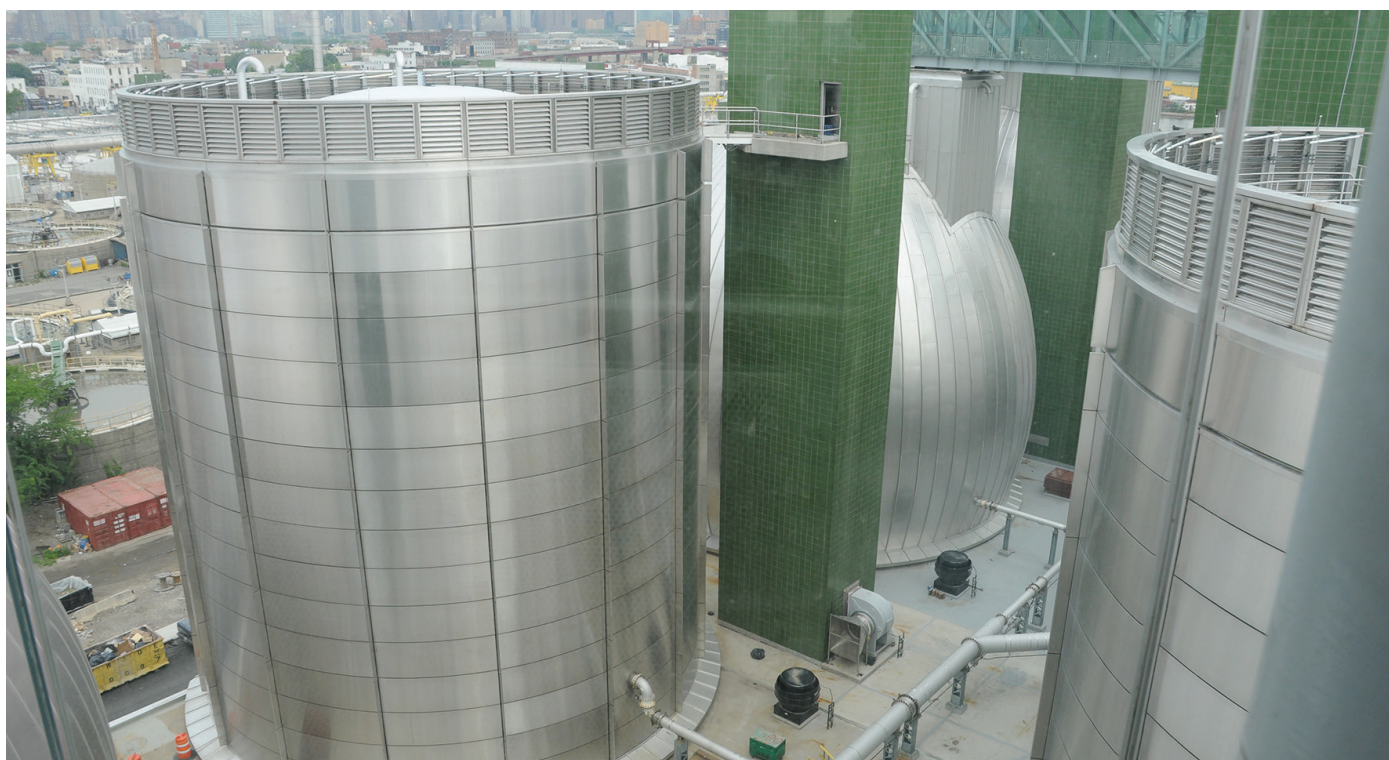
Newtown Creek Wastewater Treatment Plant
