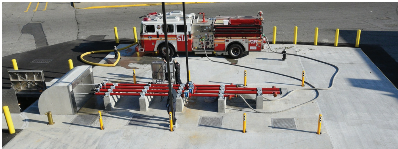
FDNY’s water recovery facility on Randall’s Island (Photo courtesy of FDNY)
