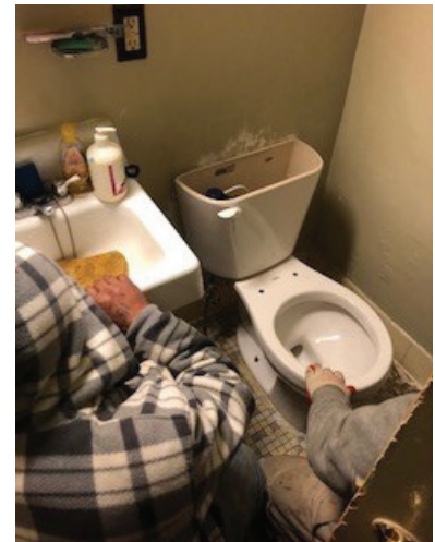
Installation of a new, high efficiency toilet in an apartment at NYCHA Latimer Gardens in Queens, one of the buildings participating in TRP.
