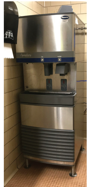
Water-cooled ice machines at NYC Health + Hospitals/Harlem will be replaced with more efficient models
