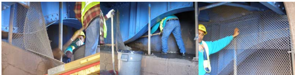
Highway Repairer Ruben Sanchez Cleaning the 174 th Street Bridge Seat. (Credit: Louis Garzia)
