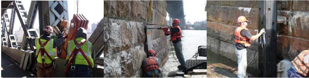
Contract #8 in 2009: Looking Southeast at the Installation of the Triangular Jacking Frame for the Intermediate Tower Bearing Replacement in January 2009. Main Tower Pier Fender System Installation in July 2009.
