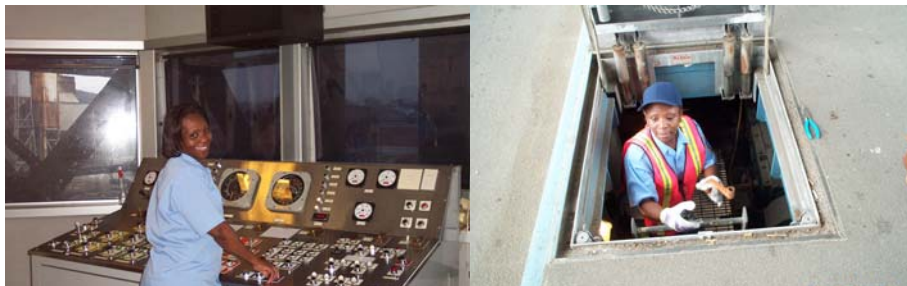
Bridge Operator-in-Charge Delonda Bates-Pinkney at the Controls of the 9th Street Bridge. She has worked for the Department since 1989. (Credit: Keith Burrowes) BOIC Bates-Pinkney Preparing to Check the Bridge's Mechanisms. (Credit: Vera Ovetskaya)
