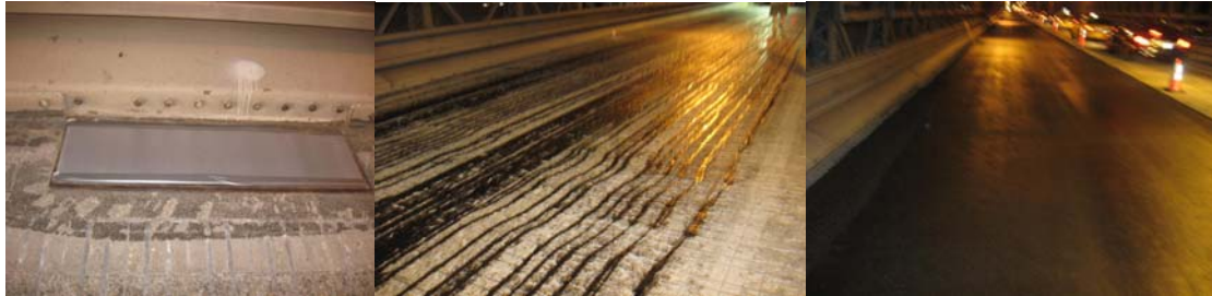
2008: Covering all the Drainage Systems Before Applying the Micro-Surfacing on the In-Bound Brooklyn Bridge. Applying the Tack Coat for the Micro-Surfacing. Applying the New Micro-Surfacing Materials. (Credit: Fouad Althaibani, Emad Shaker, and Sunil Desai)
