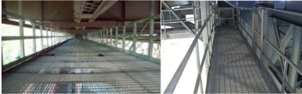
Queensboro Bridge Lower Level Flooring System Catwalk under Lower Level Queens Approach. Manhattan Bridge Brooklyn Tower Catwalk. (Credit: NYSDOT)
