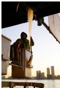
Icicle Removal From an FDR Drive Bridge.
