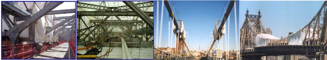
Containment Examples. Manhattan Bridge - Painting Containment Structures on the Cables of the Manhattan Approach Span. 2005: Queensboro Containment. (Queensboro Credit: Peter Basich)
