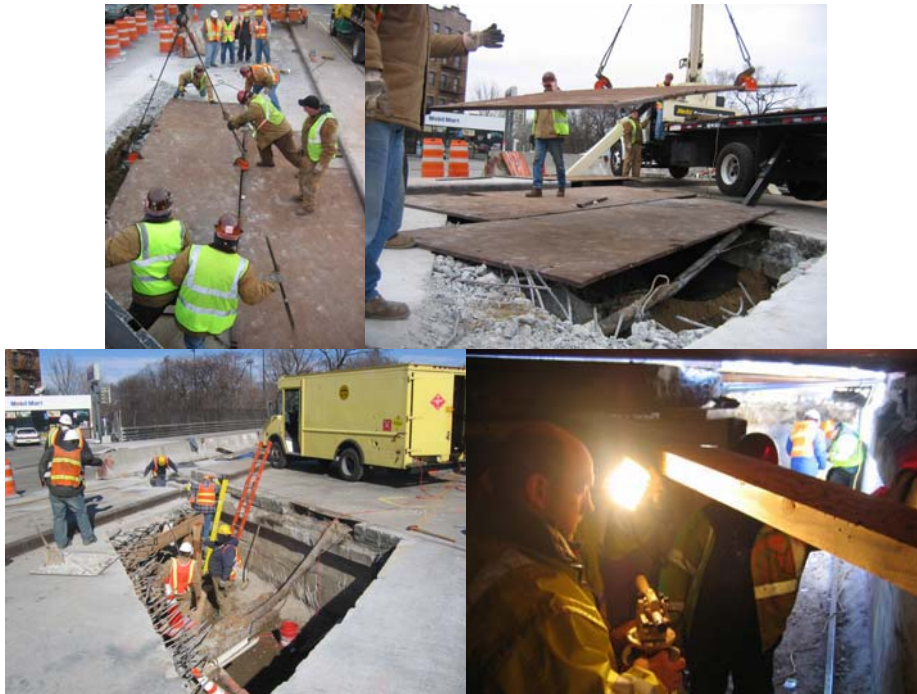
Red Flag Repairs in February 2006: Ironworkers Removed the Plates From the Holes and Replaced Them at the End of Each Day. They Also Placed Reinforcing Bars for the New Concrete Slab. Supervisor Bridge Repairer and Riveter Gean Pilipiak Monitoring Red Flag Repairs in 2006. (Credit: Peter Basich)
