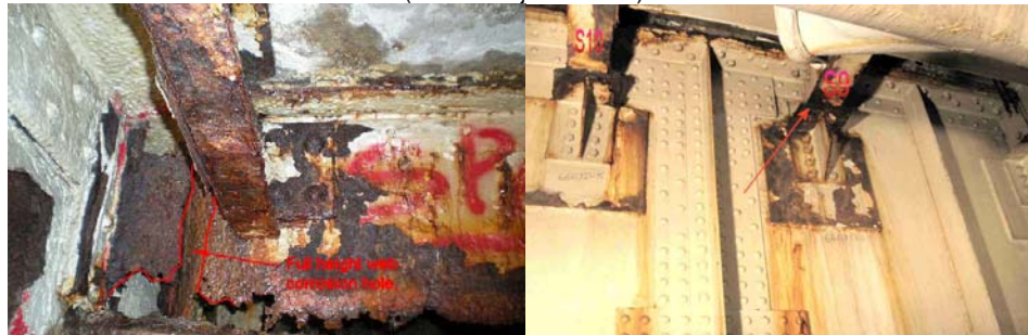
September 2008: Advanced Corrosion of Steel Stringer and Girder.
