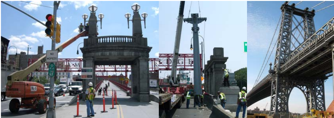
2008: Installation of Luminaires at the Manhattan Plaza Bridge Entrance. Erection of the Manhattan Entry Electrolier. Brooklyn Tower in October 2008. (Tower Credit: Russell Holcomb)
