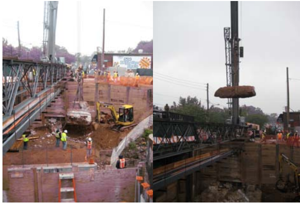
Annadale Road Bridge: Removing the North Abutment Footing and the Partly Embedded Abandoned Sewer Pipe Containing Asbestos in May 2009.
