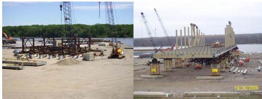
June and October 2009: Assembling the Willis Avenue Bridge Swing Span near Albany, New York.
