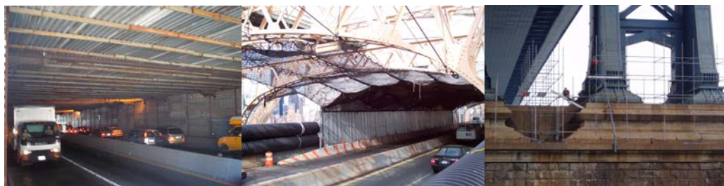
2007: Queensboro Bridge Lower Level and Upper Level Shielding. 2006: Erecting Scaffolding to Build Painting Containment at Base of Brooklyn Tower of the Manhattan Bridge.
