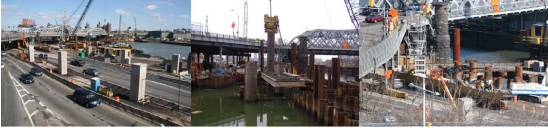
View From Harlem River Drive in February 2009. Manhattan Relieving Platform in July 2008 and February 2009.
