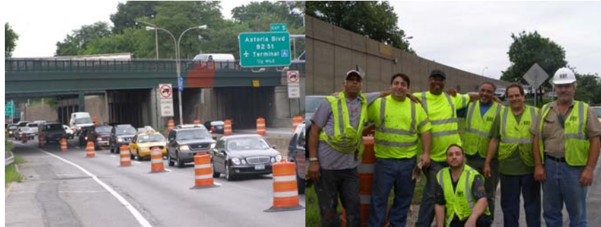
Painting Along the Grand Central Parkway in August 2009. Crew: Bridge Painters Joao Silva, Thomas Anzalone, Reynaldo Grant, Michael Scotti, Oswaldo Lima, Albert Pappas, and Supervisor Bridge Painter Georgeios Ploumis. (Credit: Earlene Powell)
