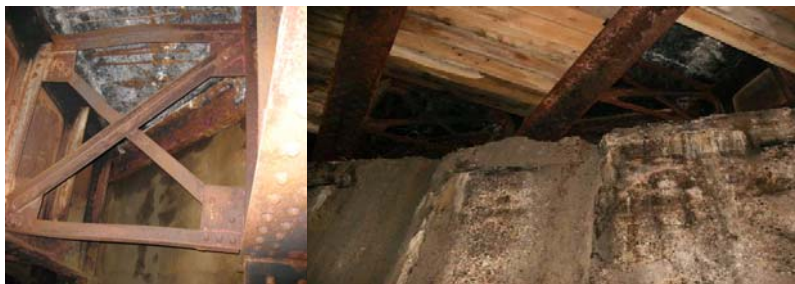
Deteriorated Bridge Deck With Exposed Rebar and Warped Steel Bracing Due to the Heat From the Fire. Timber Shielding on the Underside of the Bridge.
