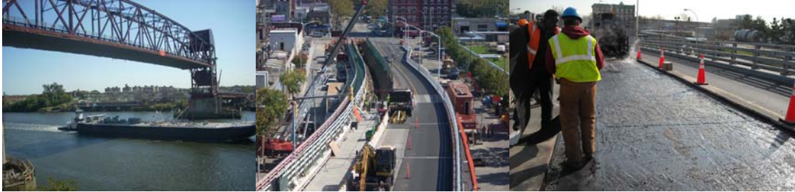
Open Lift Span During United Nations General Assembly Week in September 2008. Stage II Roadway Construction of the Queens Approach in October 2008. Asphalt Placement on the Queens Approach in November 2008.
