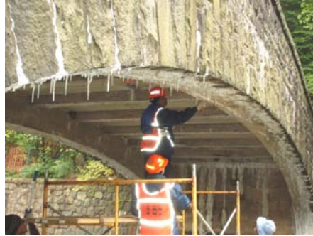
Inspecting the Bridge over the Dam at the North End of Clove Lake in Staten Island in October 2009. (Credit: Syed Mahmood)
