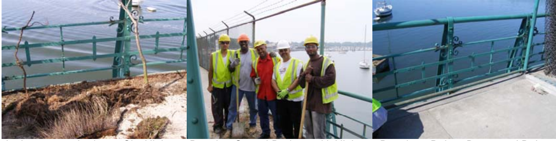
In June 2009, Assistant City Highway Repairer Seveul Redzeposki, Highway Repairers Robert Bynes and Ruben Sanchez, Supervisor Highway Repairer Dionisio Matos, and Assistant City Highway Repairer E'boni Brown Removed Vegetation From the Fascia Girder and Performed Chain Link Fence Repairs on the City Island Bridge. (Credit: Paul Schwartz)
