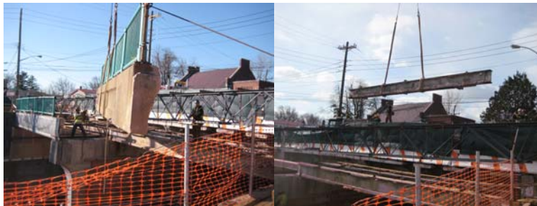
Annadale Road Bridge: Removing the Eastern Bridge Railing Fence and the Stringer in February 2009.
