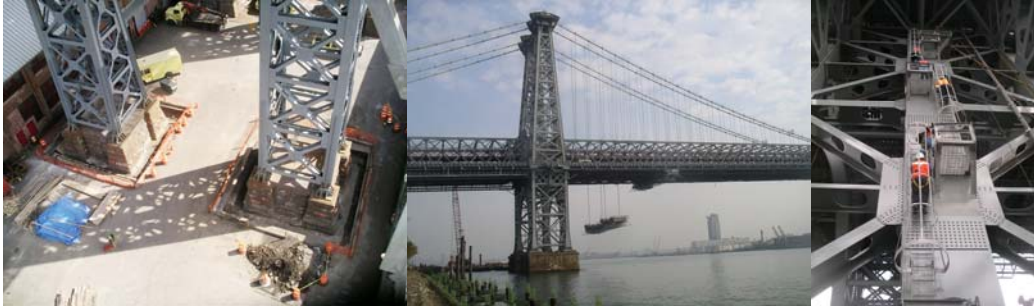
2007: Seismic Retrofit Concrete Work in Brooklyn. Raising the Manhattan Side Traveler at the Manhattan Tower. Manhattan Tower North.
