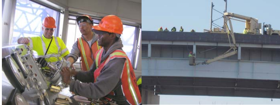
Construction Project Manager Gholamali Mozaffari, and Electricians Nelson Crooks and Gary Emmanuel Fixing Machinery in the Ninth Street Bridge Operator House in April 2008. (Credit: Vera Ovetskaya) Repairing the Navigation Lighting on the Hunterspoint Bridge. On the Bridge: Oilers Carl Wharton, Richard Morreale, and Paul Califano, Mozaffari Ali, Electrician Naum Golburt, and Highway Repairers Manny Nardiello and Kevin Donahue. In the Snooper Bucket: Harry Parmaman and Supervisor Electrician Jose Done. (Credit: Samuel Teaw)
