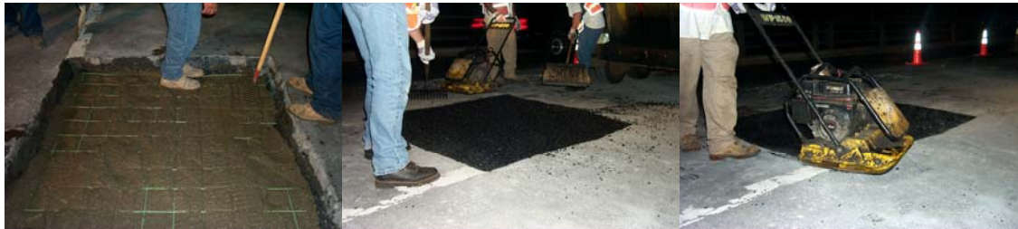
2005: Installing New Concrete With Rebar in the Cutout on the Eastbound BQE. Rolling and Tamping the Asphalt on the Eastbound BQE. (Credit: Anthony Napolitano)
