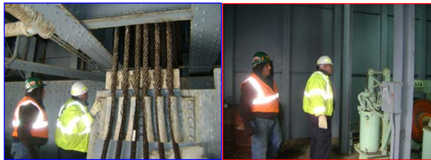
Executive Director of Bridge Preventive Maintenance and Repair Thomas Whitehouse (Wearing Yellow Jacket) Inspecting the Broadway Bridge Machinery Room and Instructing the Contractor. (Credit: Albert Hong)
