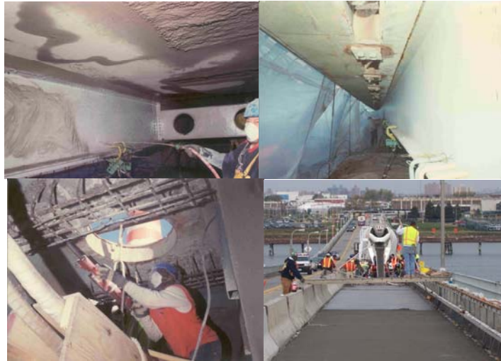
2006: Performing Underdeck Repairs. Working Inside the West Rebar Box Frame. Beam Repair. Concrete Placement.
