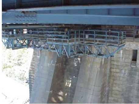
Manhattan Bridge Traveler. (Credit: NYSDOT)
