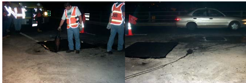
2005: Sealing the Edges of the Cutout With Asphalt Cement to Prevent Water From Seeping In. Closeup of Part of the Completed Concrete Deck Repair on the Eastbound BQE. (Credit: Anthony Napolitano)
