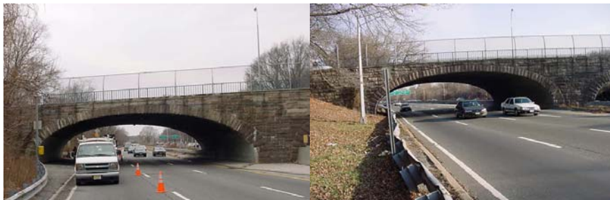
130 th Avenue Bridges over Laurelton Parkway (EB and WB) in 2002. (Credit: NYSDOT)
