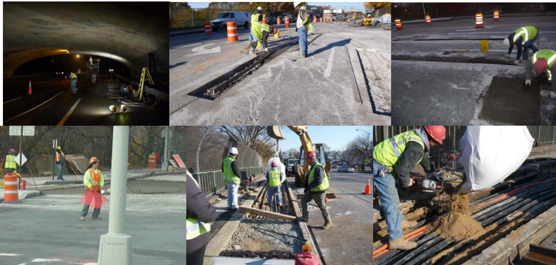
Merrick Boulevard Bridges: Repairing the Under Deck in September 2009. Deck and Sidewalk Repairs in November and December 2009.
