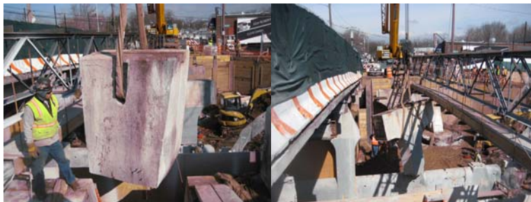
Annadale Road Bridge: Removing the South Abutment and Center Pier in March 2009.
