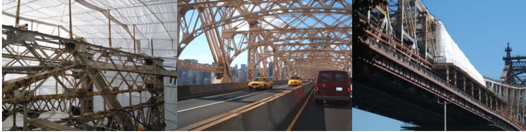
Protective Coating in 2006: Inside the Containment Rigging at Span #1. Finish Coat on the Trusses at Span #5 on the Upper Roadway. Class 1A Containment Installed on the Trusses at Span #2, And the Working Platform Above the South Outer Roadway.
