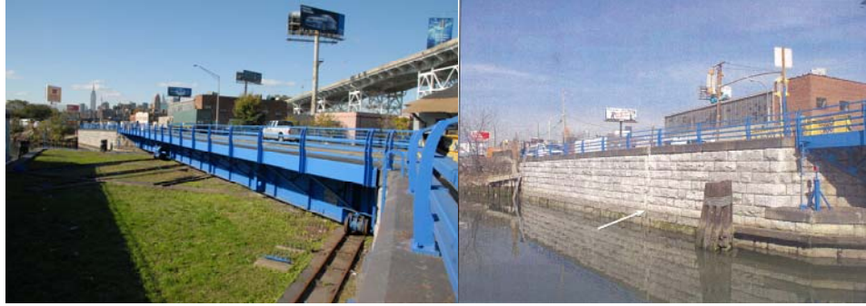
Borden Avenue Bridge. (Credit: Peter Basich) General View of the Crack in the Wingwall.
