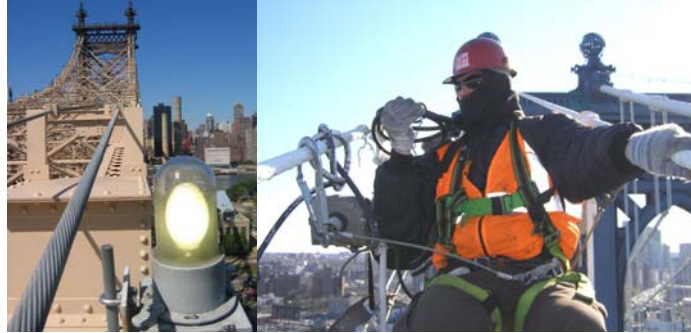
A Bulb of the Queensboro Bridge Necklace Lights. (Credit: Peter Basich) Repairing a Manhattan Bridge Necklace Light. (Credit: Hany Soliman)
