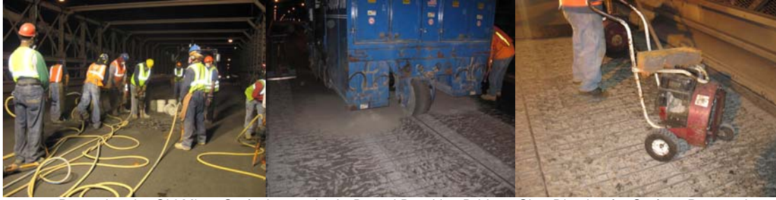
2008: Removing the Old Micro-Surfacing on the In-Bound Brooklyn Bridge. Shot Blasting for Surface Preparation. Cleaning the Roadway Surface. (Credit: Fouad Althaibani, Emad Shaker, and Sunil Desai)
