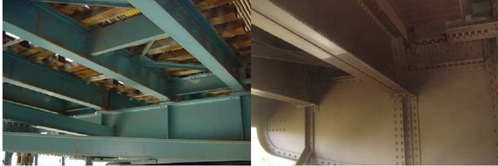
South Transit Floorbeams, Stringers, and Bracing Members on the Manhattan Bridge. Queensboro Bridge North Outer Roadway Floorbeam. (Credit: NYSDOT)
