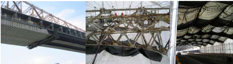
Platform Installed for Painting of the Queensboro Bridge. (Credit: Vadim Sokolovsky) Working Inside the Containment. Protected Roadway.
