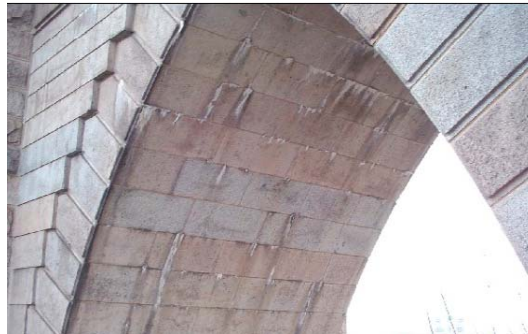
Moderate Efflorescence on the Brooklyn Bridge Brooklyn Tower North Gothic Arch in 2004. (Credit: NYSDOT)
