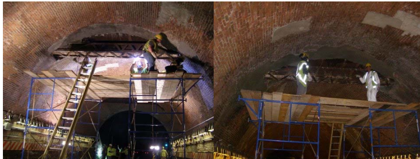
Cement Masons Frank Finizio and Paul Maguire. Bricklayer Vincent Sculla and Cement Mason Frank Finizio. (Credit: Mohammad Siddiqui)
