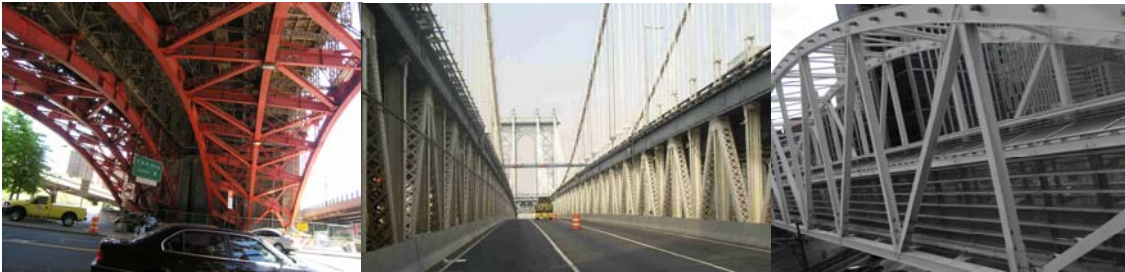
Brooklyn Bridge Franklin Square Truss. (Credit: Andy Hoang). General view of Manhattan Bridge Trusses B and C From the Lower Roadway on the Main Span. (Credit: NYSDOT) Chambers Street Pedestrian Bridge Truss.
