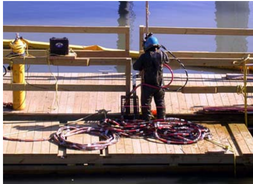
Diver Preparing to Inspect the Borden Avenue Bridge in April 2009. (Credit: Bernard Ente)
