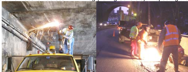
PIA Flag (Truck Wedged Under the FDR Drive at Span 41): Removing the Debris. (Credit: Victor Sandoval) PIA Flag Repair (Through Hole) on Harlem River Drive Ramp. (Credit: Bojidar Yanev)
