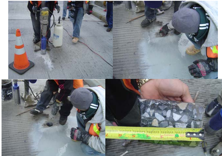
Removing a Core From 252 nd Street Bridge over Henry Hudson Parkway in January 2009. (Credit: Masroor Mahmood)
