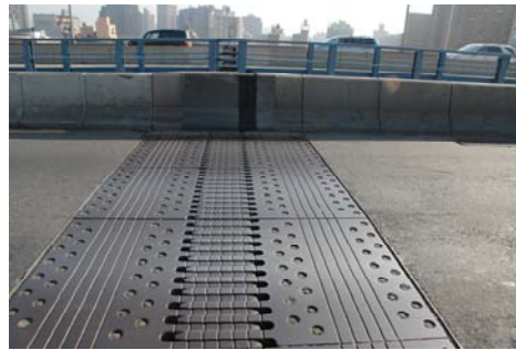
Manhattan Bridge Finger Dam. (Credit: Jagtar Khinda)
