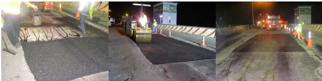
Belt Parkway Bridge over Mill Basin: Installation of New Asphalt. Compacting the Asphalt With the Assistance of a Gasoline Roller Engineer From the Roadway Repair and Maintenance Division. Completed Resurfacing Work. (Installation Credit: Yousef Demis, GRE Credit: Ali Mozaffari)
