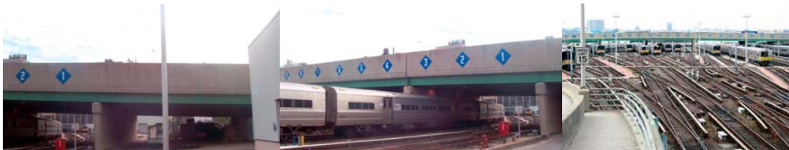
11 th Avenue Viaduct (West 30 th Street to West 33 rd Street) in 2006. (Credit: NYSDOT)
