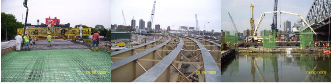
Willis Avenue Bridge August 2009: Placement of Deck Concrete on New Ramp to Bruckner Boulevard. Curved Girders on New Ramp. Placing Concrete in Pier 7 Box.
