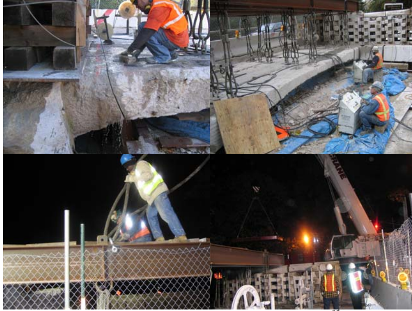
2006: Wire Sawing the Deck and Removing the Existing West 252 nd Street Bridge Sections Over the Parkway.
