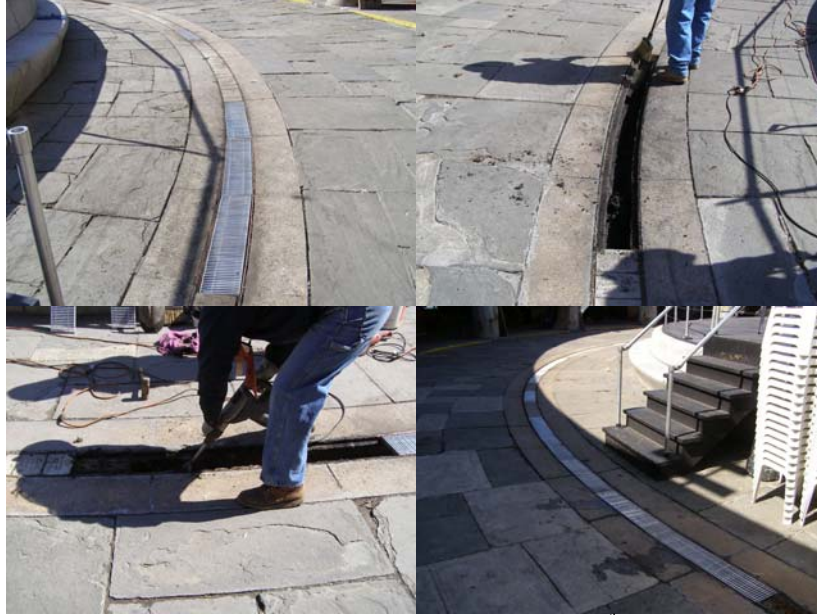
Installing Steel Grating for the Circular Gutter at the West 79 th Street Rotunda in March 2009.
