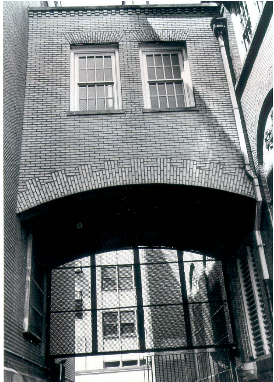
Newtown High School, Borough of Queens Bridge between auditorium and southeast wings
