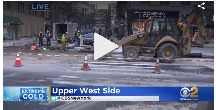
BWSO was quick to respond to a recent water main break in Manhattan.
