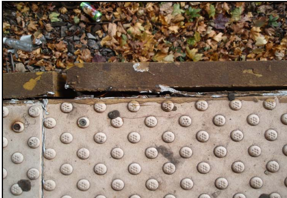
Loose Rubbing Board at Edge of Platform at the Cortelyou Road Station
