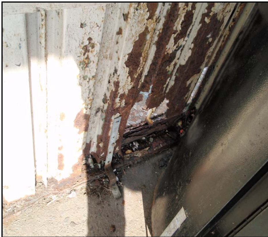
Eight-Inch Hole in Metal Wall Panel of Elevated Platform At the 111 th Street-Greenwood Ave. Station
