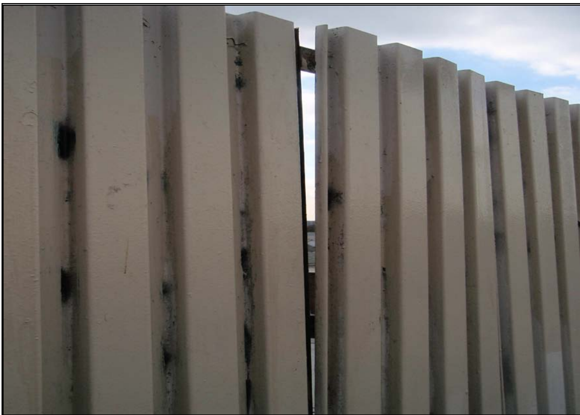
Loose Wall Panel on Elevated Platform at the 88 th Street-Boyd Street Station
