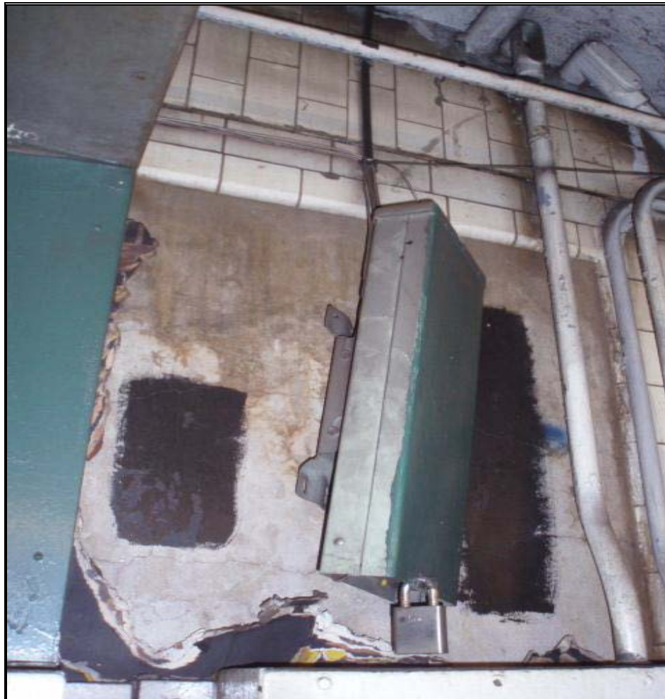
Loose Electrical Box Hanging from Wire at the 116 th Street Station
