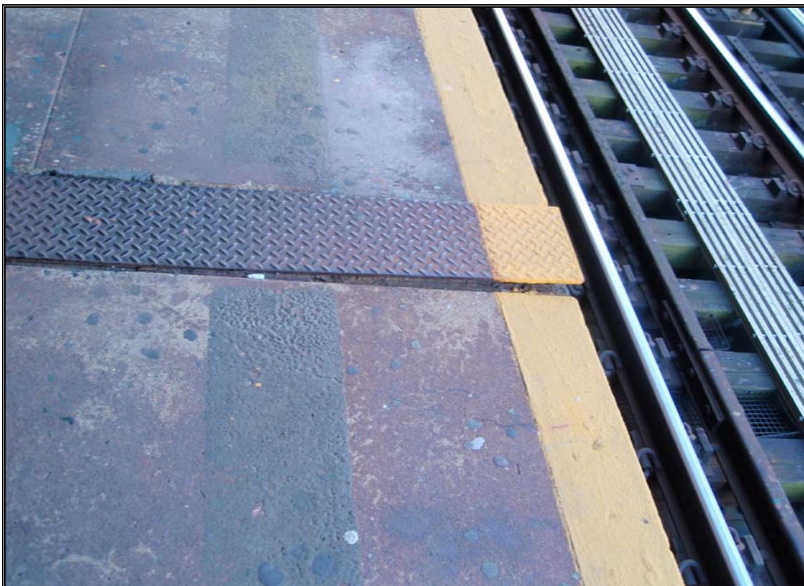
Raised Expansion Plate on Elevated Platform At the 111 th Street-Greenwood Avenue Station
