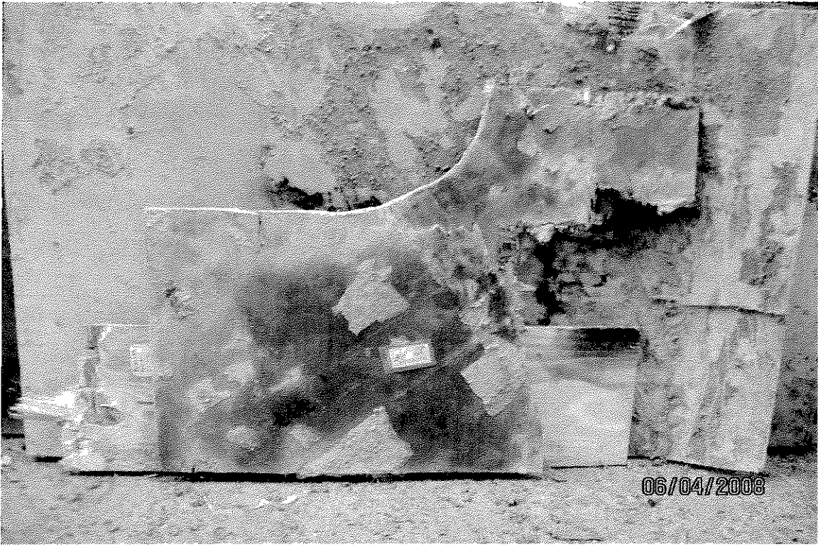
Photo 17 - Failure pattern consistent with a base plate punch through failure in panel DOB #PW41019.
