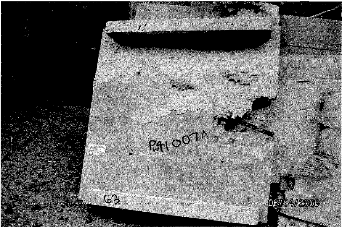
Photo 18 - Failure pattern consistent with a base plate punch through failure in panel DOB #PW41007A.
