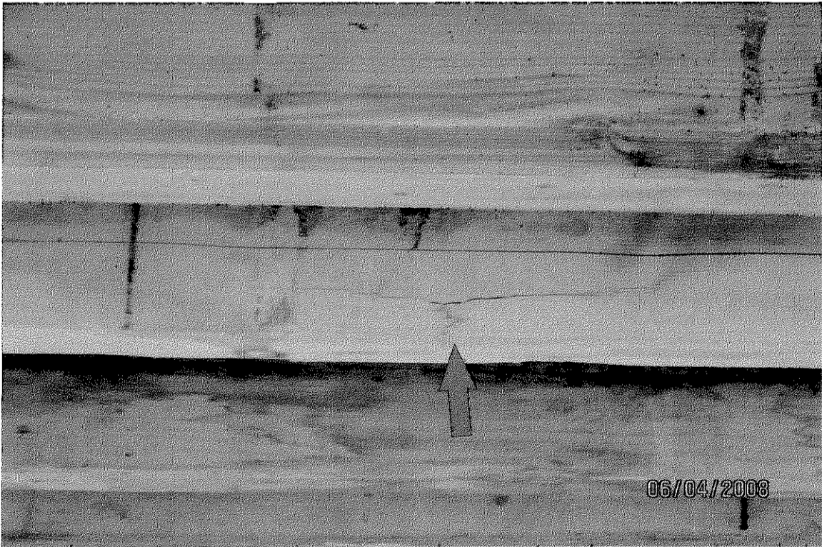
Photo 13 - A 3x4 lumber rib exhibiting a brash failure being used in formwork during our inspection.
