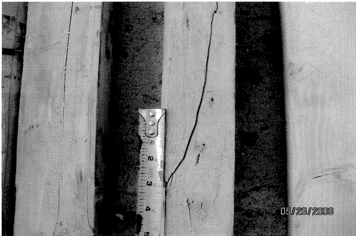
Photo 4 - Slope-of-grain of 1:3 in 3x4 stored on 40 th floor.
