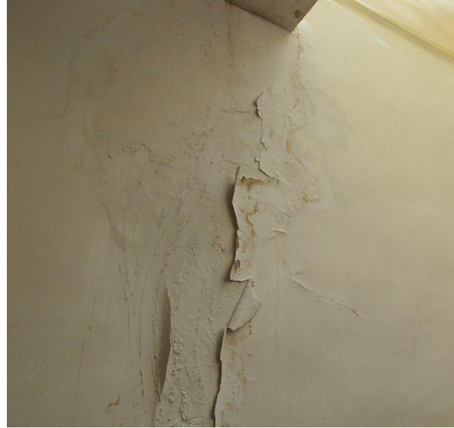
Figure 9: Mike's House (hotel). Severely chipped paint and water damage in the public hallway.
