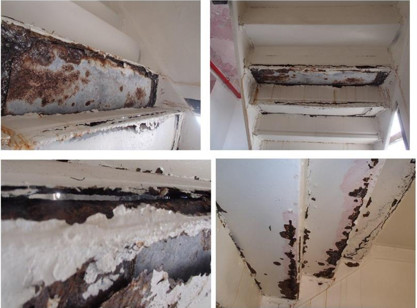
Figure 11: Regent Family Residence Stairway A: severely corroded and rusted stairs. Visible large holes (bottom left). The DOI inspection resulted in fire guards being placed at the stairs 24 hours a day.
