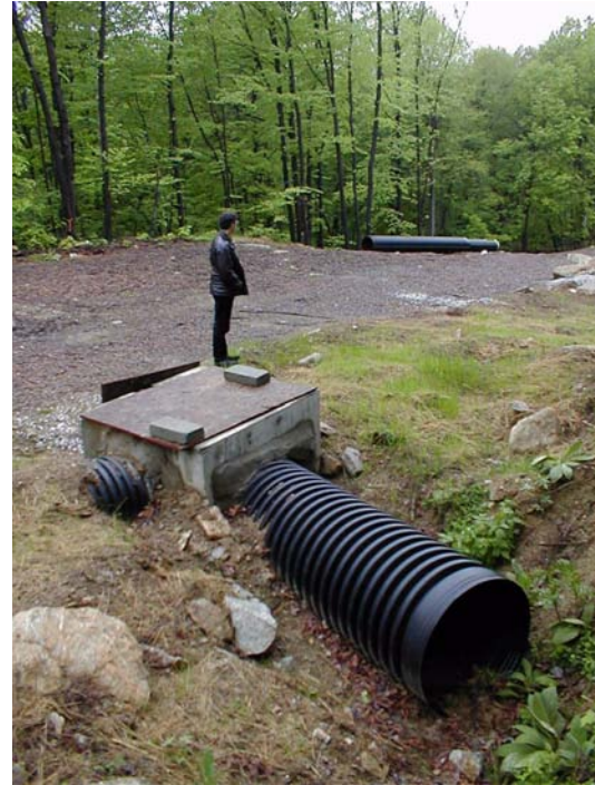
Figure 5.1 Watershed Protection Program's attempt to displace or control excessive runoff that can result from activities or land uses that disrupt vegetation or create impervious surfaces which prevent the natural infiltration of rainfall.
