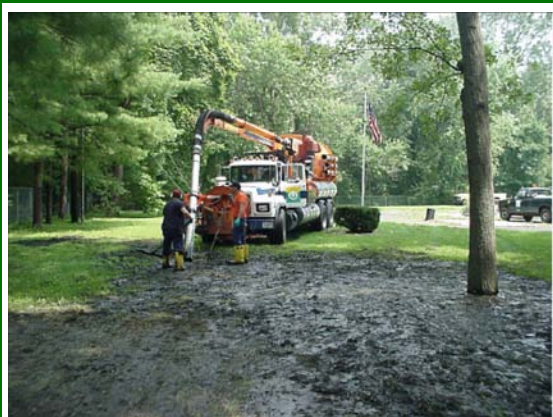
Figure 3.14 Vacuum truck removing spilled sludge at Yorktown Heights WWTP, Muscoot Reservoir watershed.
