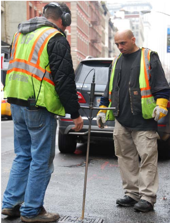
Figure 18: Sonar hearing detection for leaks
