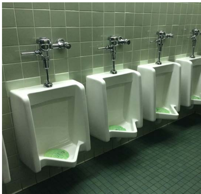
Figure 5: Retrofitted urinals at P.S. 1 in Staten Island
