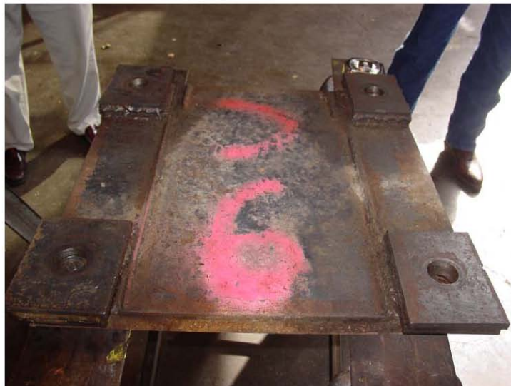
Figure 2 Ninth Floor Horizontal Tie Beam Base Plate 9C With Weld Fractures.
