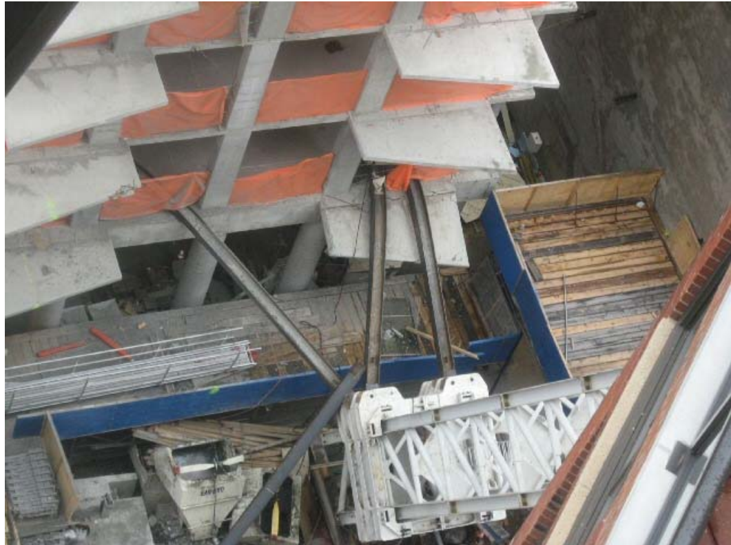
Photograph 1.14 - 3rd floor collar assembly following the collapse. The 9th floor collar and 18th floor collar rest atop the 3rd floor collar. Source: New York County District Attorney IMG_0355_085.jpg.
