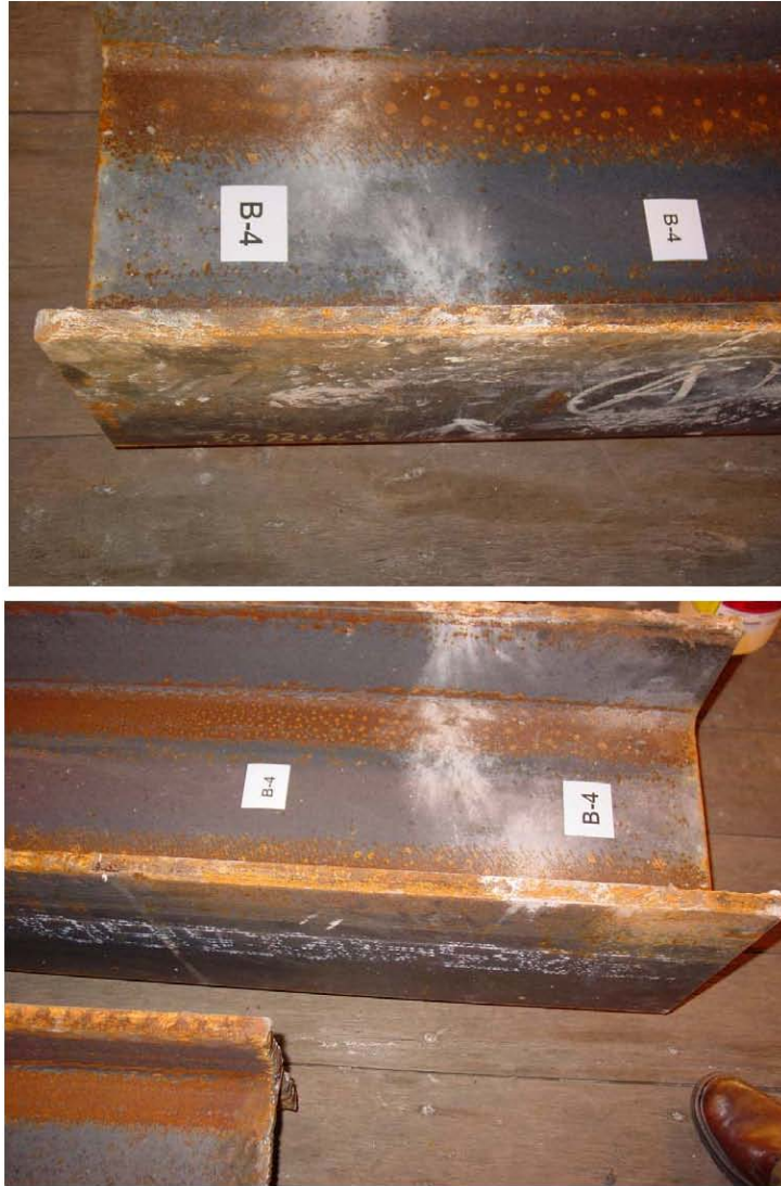
Figure 12 General Views of Weld Fracture on Tie Beam B4.
