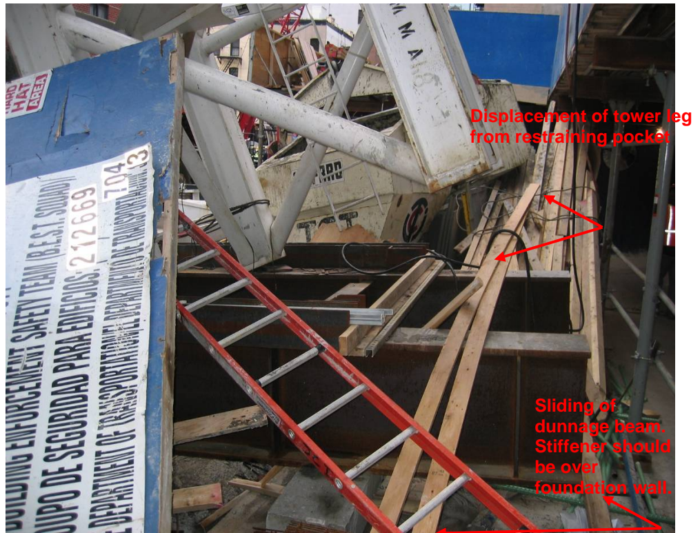
Photograph 11.3 - Base of tower crane after collapse. Note the movement of the dunnage beam and displacement of the tower legs from their restraining pockets. Photo from New York County District Attorney IMG_0379_109.jpg.
