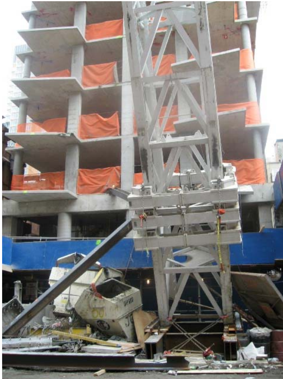
Photograph 1.4 – Photograph showing conditions at tower base following the collapse (source: New York County District Attorney’s Office, Photograph ID No. IMG-0332-062).
