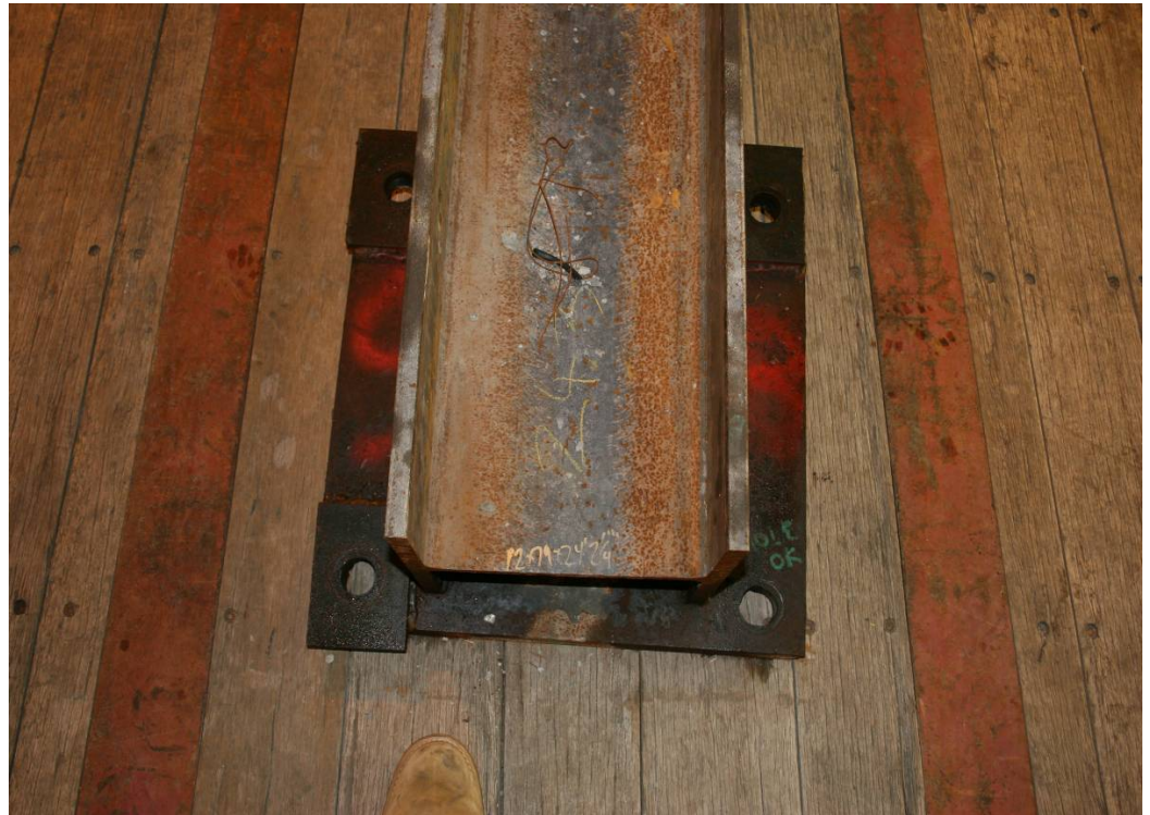
Photograph 9.3 – Base plate 9B from floor level 9. The tie-beam is still attached. Photo by Arup.
