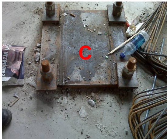
Photograph 1.10 – Conditions at 9 th Floor: Failed base plate 9C for Beam B5 prior to its removal from the site (the bent beam in the photograph is Beam 9B). Photos provided by the NYCDOB.
