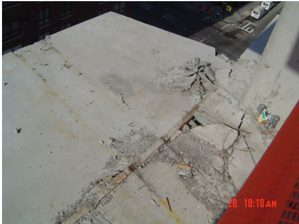
Photograph 1.18 - Damage to 9th floor balcony. The imprint in the slab is from Beam 9B. Photo by Arup.
