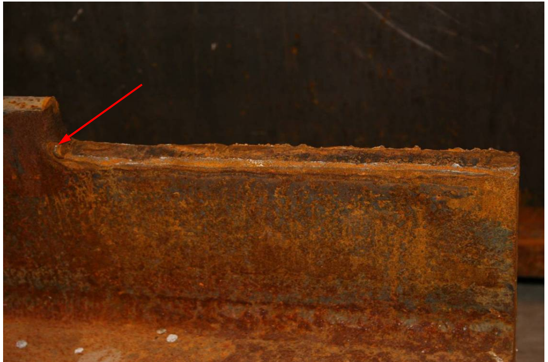
Photograph 3.20 - Tie-Beam 9A (9th floor level collar, formerly located at the east side of the collar). Collar end. Note the lack of clearance between the end of the failed fillet weld and the radiused cut in the beam flange (at arrow location). Photo by Arup.
