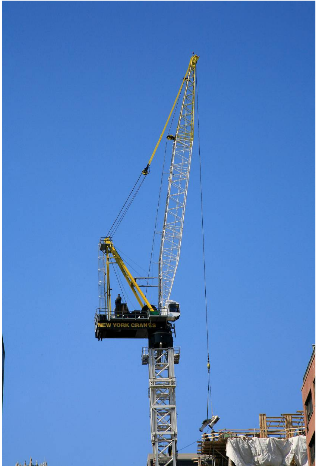
Photograph 1.7 - Photograph showing the position of the crane boom during tie-in assembly, approximately 1 hour before the crane collapse (source: photograph by Gary Halby).
