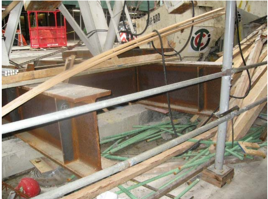
Photograph 1.5 – Photograph showing conditions at tower base following the collapse (source: New York County District Attorney’s Office, Photograph ID No. IMG-0372-102).
