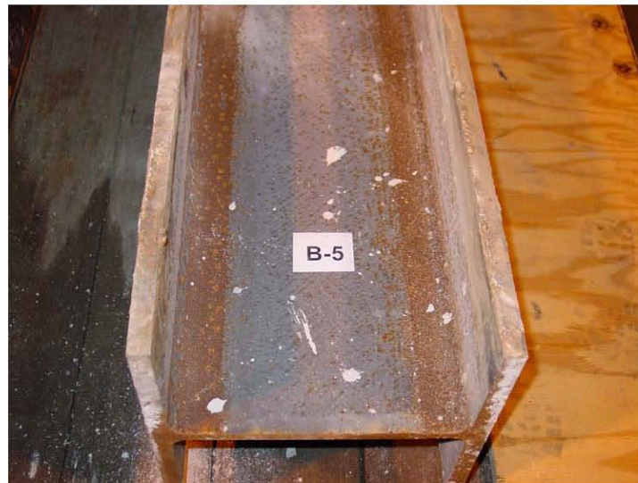
Figure 4 Ninth Floor Horizontal Tie Beam (B5) End With Weld Fractures. (Welded to Base Plate 9C).
