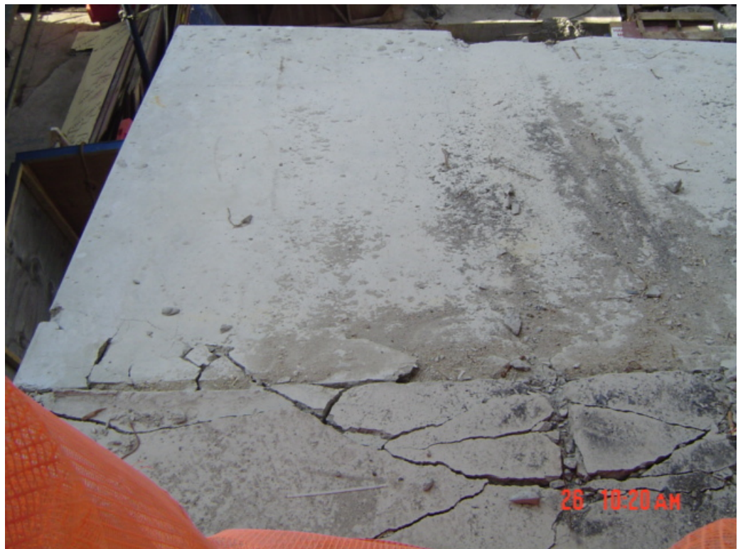
Photograph 1.19 - Damage to 3rd floor balcony. Photo by Arup.
