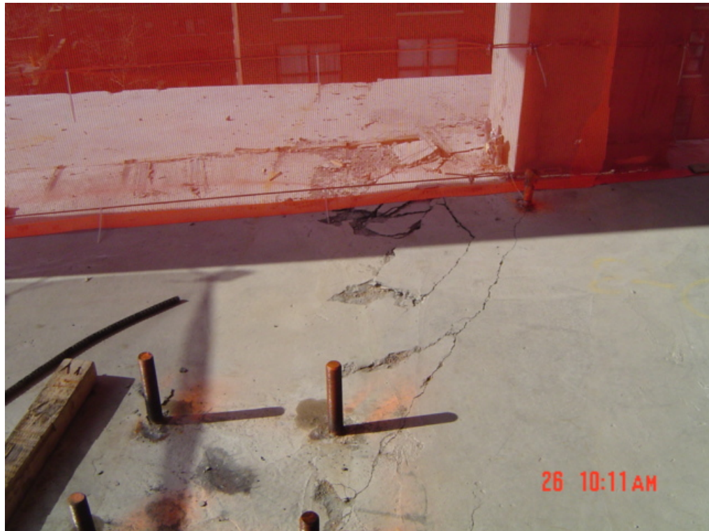
Photograph 1.20 - Minor spalling of concrete in the vicinity of the bolted connections to the 9th floor slab. Photo by Arup.
