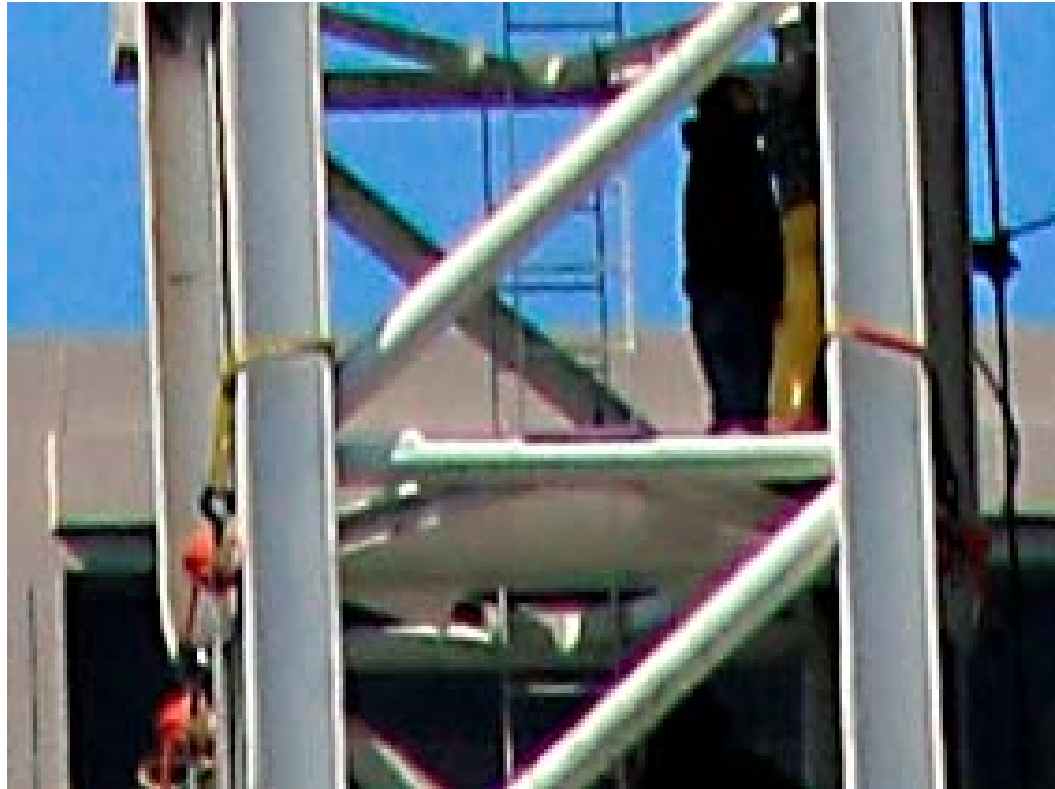
Photograph 3.1 - Close-up of crane tower shortly before collapse. Two polyester web slings are seen in a choker hitch around the legs of the tower. (Source: photograph by Gary Halby.
