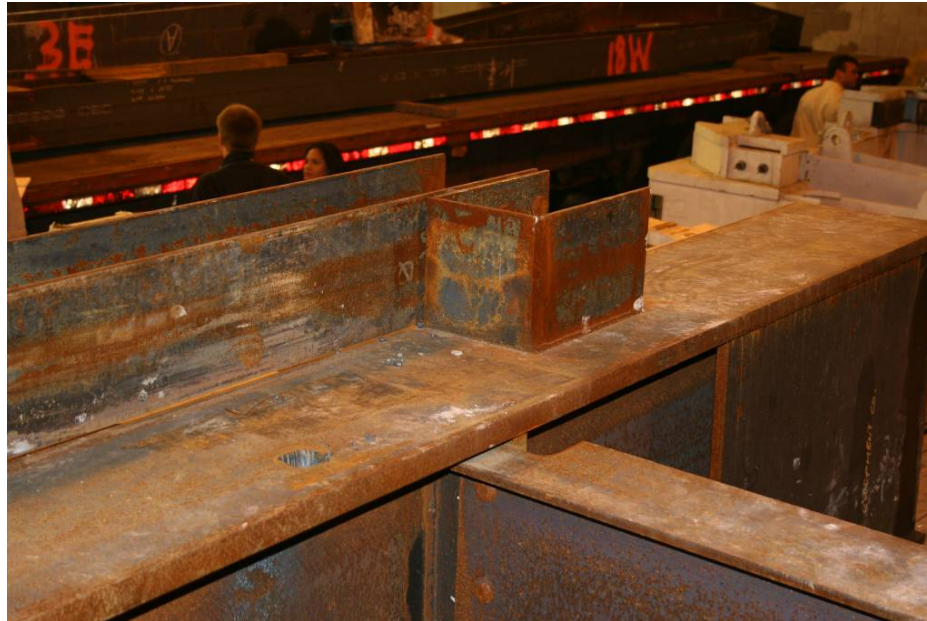
Photograph 1.1 - Dunnage steel at the base of the tower crane (source: lmg_0282 from April 18, 2008 visit to OEM warehouse by Arup). Visible in the photo are a W24x194 dunnage beam with a W24x55 cross-brace and W8x31 sections to create lateral restraint for the tower legs. Note the absence of anchorage for tower legs, which rested in the nooks created by the W8x31's.
