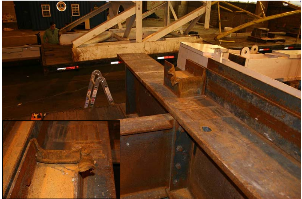
Photograph 7.1 - Dunnage foundation. The inward deformation visible in the closeup of the deformed pocket indicates that the steel plate at the end of the pocket was squashed due to a downward force from the tower legs. Had failure occurred due to a horizontal sliding load the plate would have been deformed in the opposing direction. Photo by Arup.
