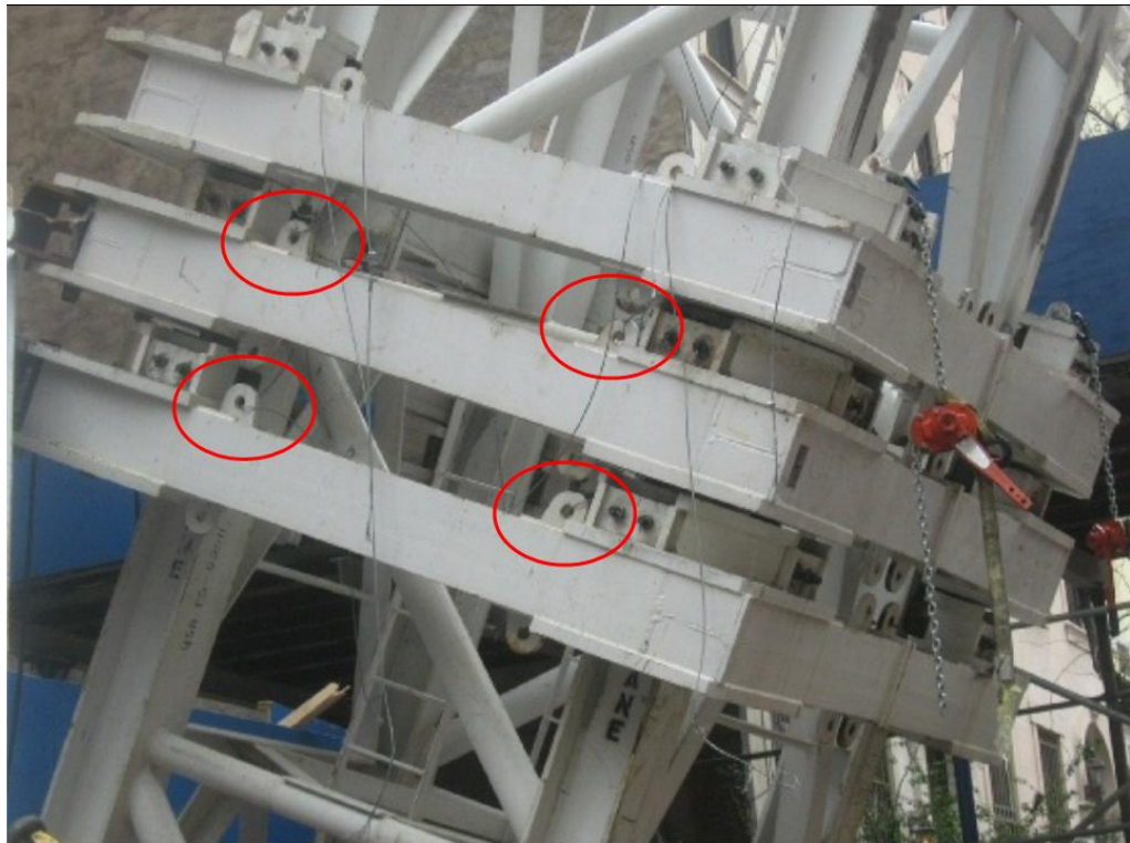
Photograph 3.5 - View of the west elevation of the collapsed tower collars. The location of visible wire rope attachments to the collars are circled. Note the lack of thimbles in the formed sling. Photo from New York County District Attorney 328_58.jpg.
