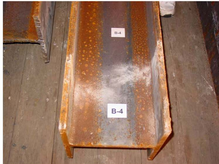
Figure 3 Ninth Floor Horizontal Tie Beam B4 End With Weld Fractures. (Welded to Base Plate 9A).
