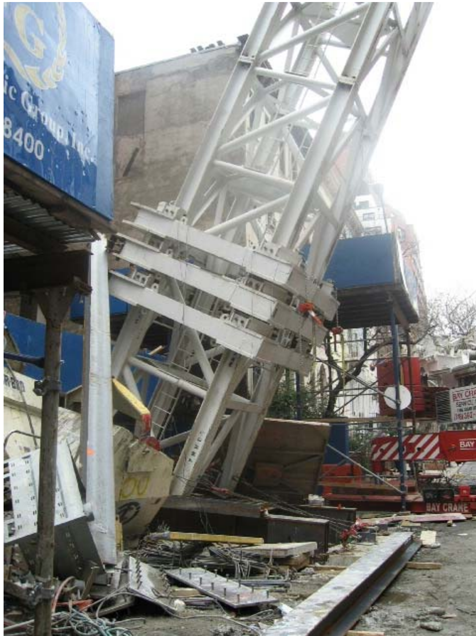
Photograph 1.3 - Photograph showing conditions at tower base following the collapse (source: New York County District Attorney's Office, Photograph ID No. IMG-0326-056).
