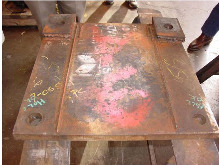
Figure 1 Ninth Floor Horizontal Tie Beam Base Plate 9A With Weld Fractures.
