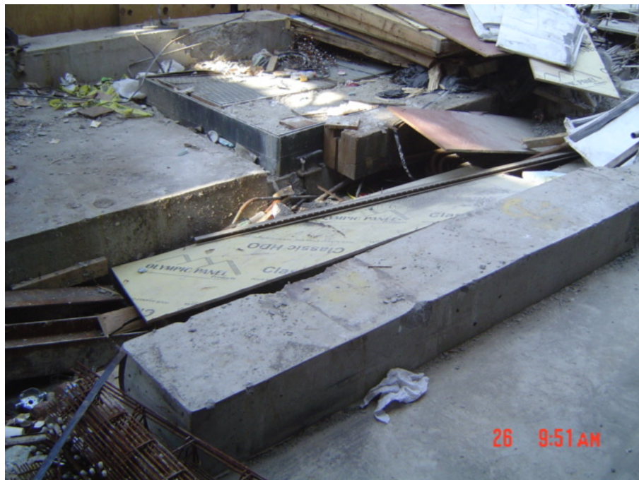
Photograph 1.2 - Tower foundations (source: photograph entitled "Manhattan Crane Collapse (03-26-08) 005" from March 26, 2008 visit to the collapse site by Arup). The foundation wall for the building is in the foreground. The foundation support wall, which was constructed specifically for the dunnage beams, is in the background. The Con-Ed vault can be seen between the foundations (in the center of the photo). Note the absence of anchorage for the dunnage steel, as per the design. Also note the absence of significant damage to the foundations (limited spalling evident only).
