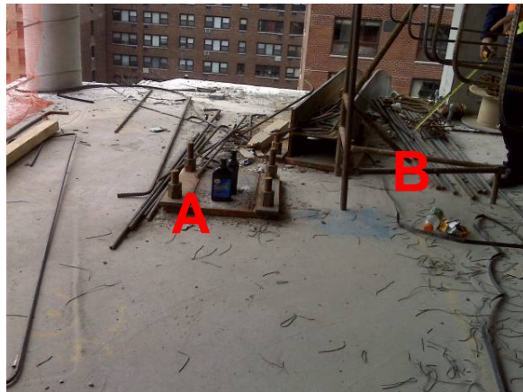
Photograph 1.9- Failed base plate 9A. Photo provided by the NYCDOB.
