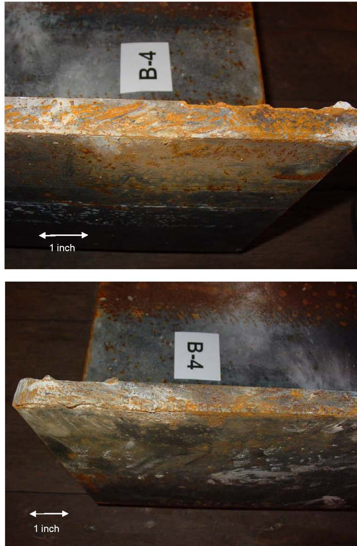
Figure 14 Enlarged Views of Ductile Weld Fracture on Tie Beam B4. Note Small Size of Deposited Weld.
