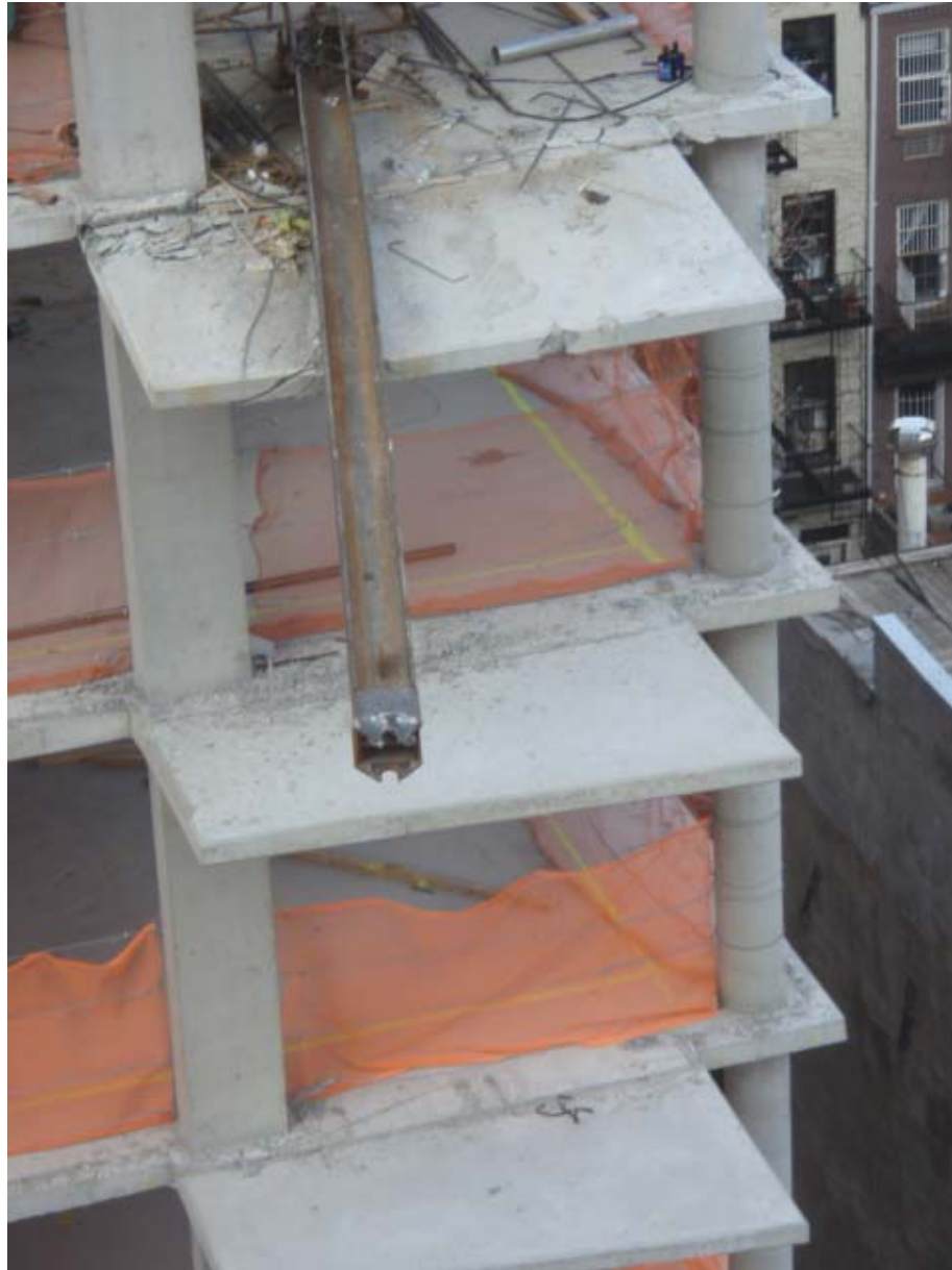
Photograph 1.13 - Failed pin end of Beam B5 at the 9 th floor level as seen immediately following the collapse. Photo provided by the NYCDOB.
