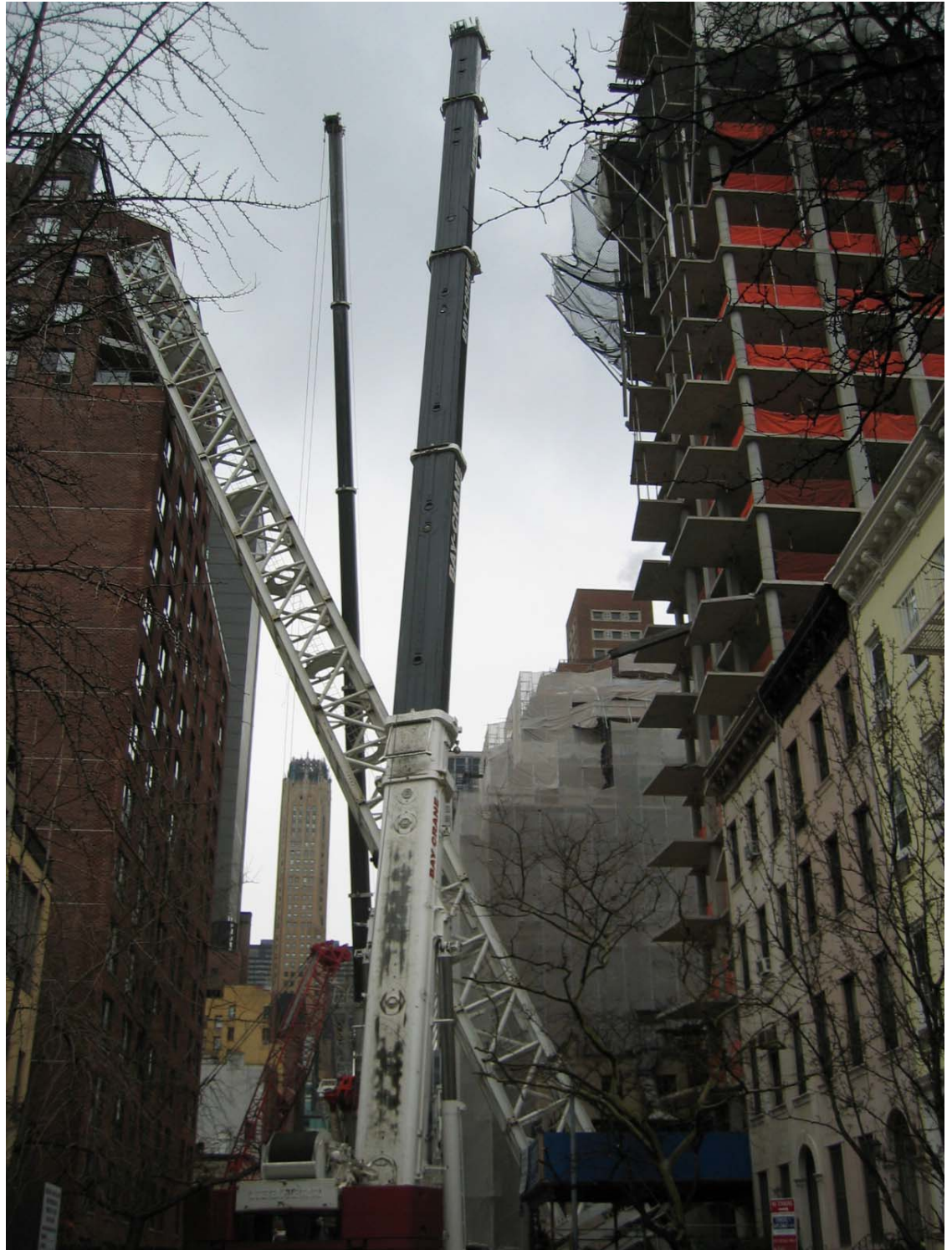
Photograph 1.22 – View of the intact tower crane after collapse. Photograph, from the crane engineer Peter Stroh, “After” photographs IMG_077.jpg.
