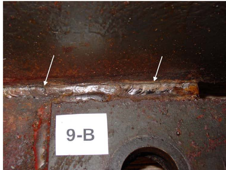
Figure 21 Enlarged View of Weld Toe Crack Observed in Base Plate 9B Weld. (see Arrows)
