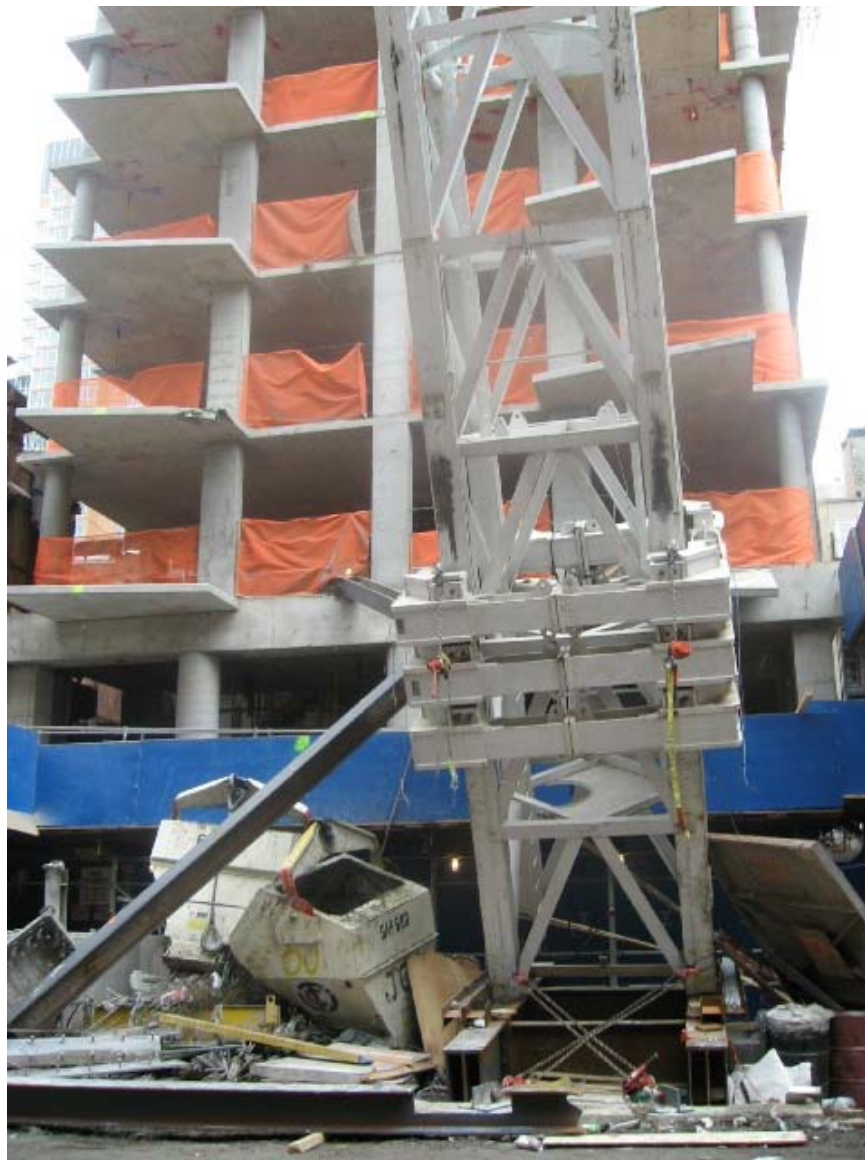
Photograph 3.4 - Base of tower crane after collapse. Note the lack of knee bracing at the base, the dunnage beam on which the tower stands and the slippage of the dunnage beam off of the submerged concrete wall foundation. Photo from New York County District Attorney IMG_332_062.jpg.
