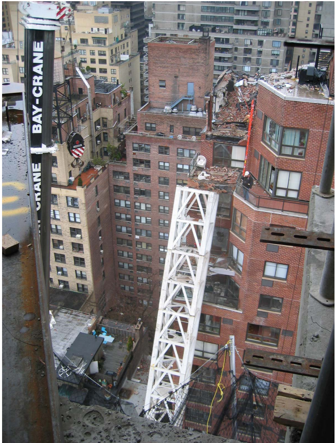
Photograph 1. 21 – View of the intact tower crane after collapse. Photograph by the crane engineer Peter Stroh, “After” photographs, IMG_066.jpg.
