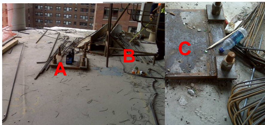
Photograph 11.1 - 9 th Floor: Failed base plate 9A for Beam B4 (labelled “A” in the photograph) and failed base plate 9C for Beam B5 (labelled “C” in the photograph) prior to its removal from the site (the bent beam in the photograph is Beam 9B). Photos provided by NYCD0B.
