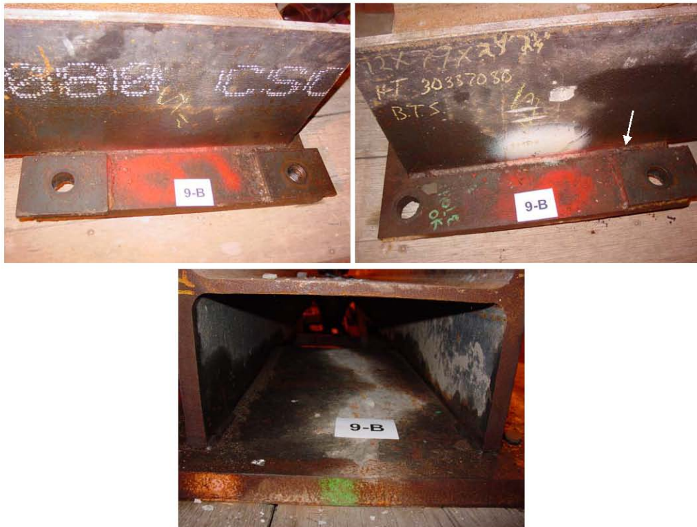
Figure 20 General Views of the Base Plate/Tie Beam Welds From Base Plate 9B.(Arrow Shows Location of Weld Toe Crack)
