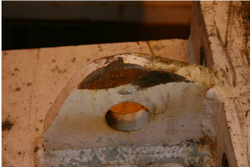
Photograph 3.12 - Collar C2-A chain block attachment point. Note the unprotected edges on which the wire rope sling would have been bearing (typical for all chain block and lifting attachments for all collars).. Photo by Arup.
