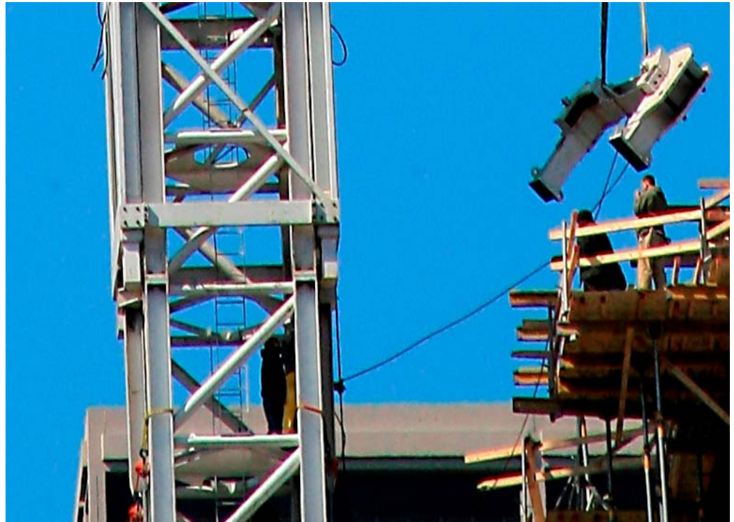
Photograph 8.1 - View of tower crane with collar half being lifted into place via polyester web slings attached to improper lifting lugs resulting in a non-horizontal position of the collar half during lift (right of photo) and chain falls incorporating polyester web slings choke hitched around the tower legs. (Source: photograph by Gary Halby).
