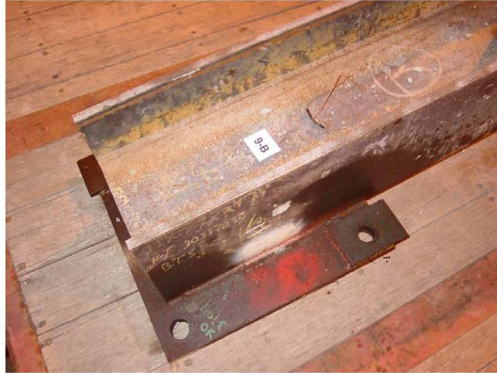
Figure 5 Intact Ninth Floor Horizontal Tie Beam and Base Plate 9B.
