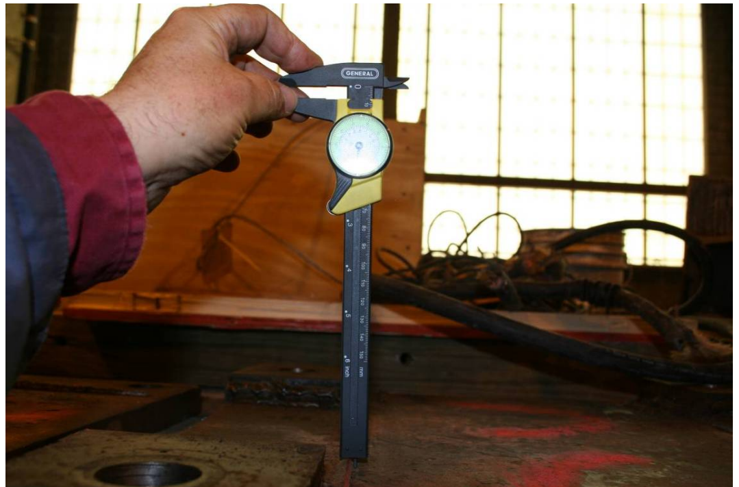
Photograph 3.22 - Fillet weld measurement of base plate 9C. Measurement is shown to be 7 mm, just under 9/32 inch which is 11.8% under the specified 5/16 inch. Photo by Arup.
