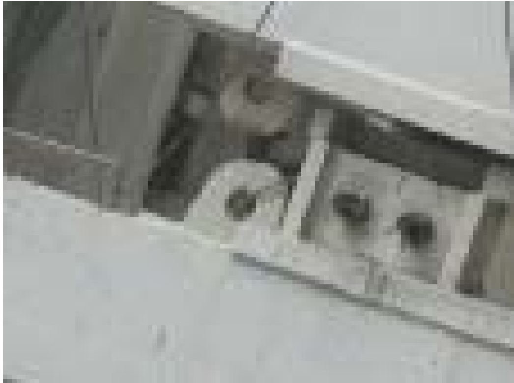
Photograph 3.16 - Close-up of 3rd floor level collar, west elevation, south corner, after collapse, showing the lack of evident protection or thimbles in the formation of the wire rope sling. Photo from New York County District Attorney 328_58.jpg.
