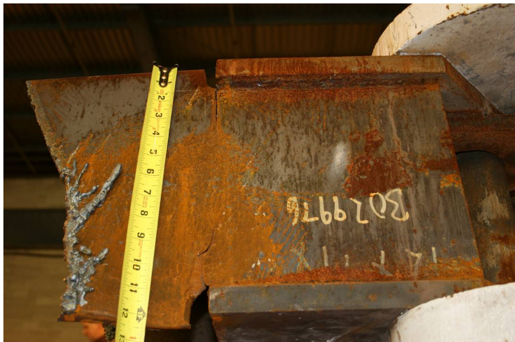
Photograph 1.15 - Fracture of a tie-beam which did not fully fail on the 3rd floor collar. (The fracture of interest is to the right of the tape measure. The damage to the left of the tape measure is a flame-cut (post failure) to assist in the removal of the debris. Photo by Arup.
