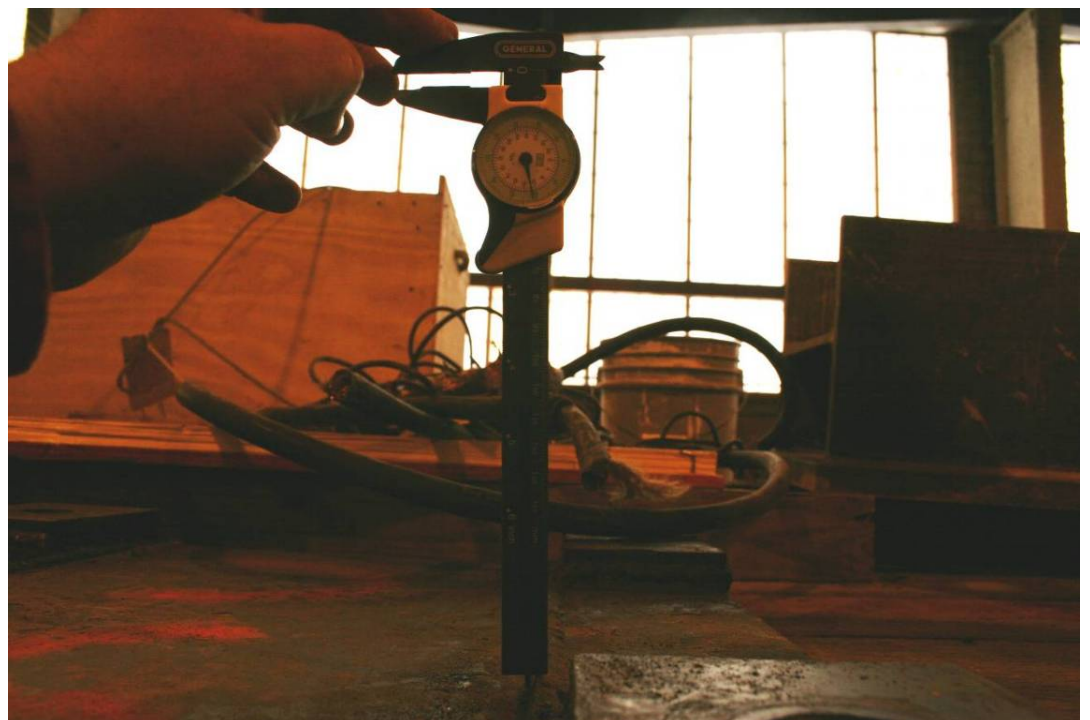
Photograph 3.23 - Fillet weld measurement of base plate 9C. Measurement is shown to be 5 mm, just over 3/16 inch, which is 37.0% under the specified 5/16 inch. Photo by Arup.
