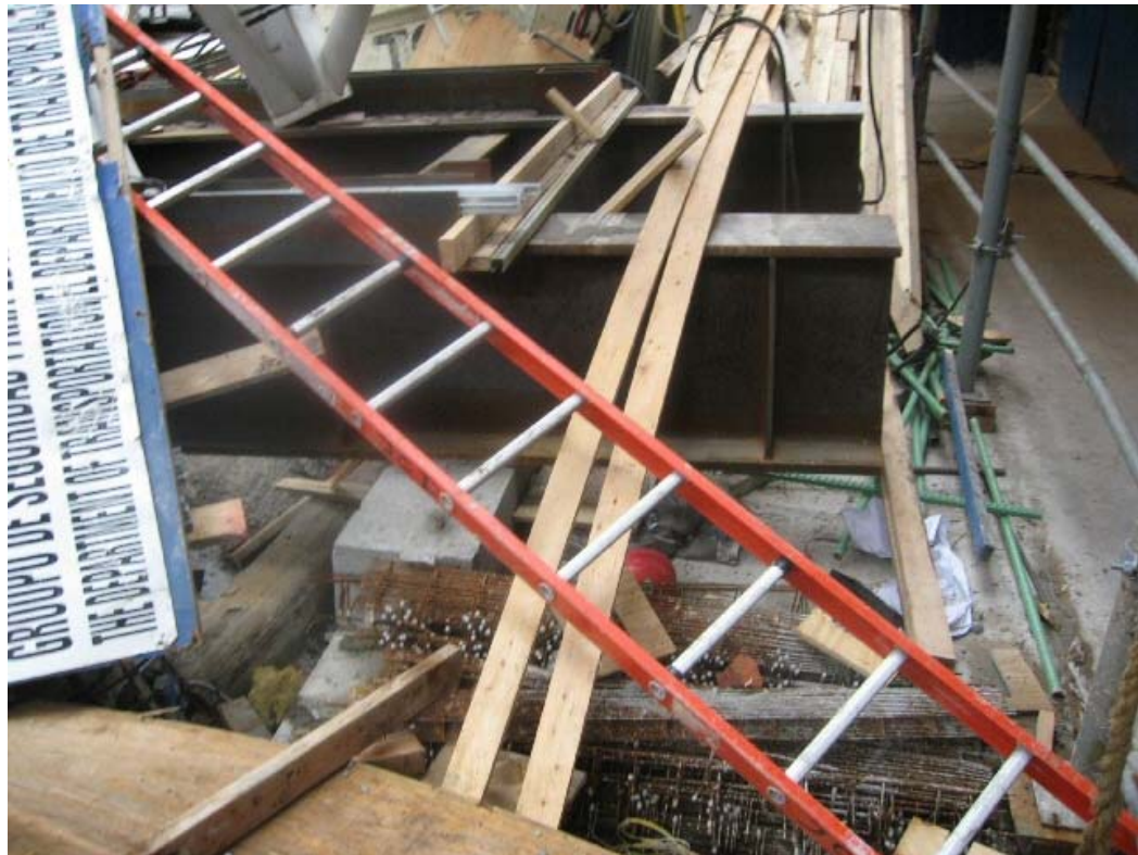
Photograph 1.17 - View of building side (north) of tower base after collapse. The dunnage beam has been displaced towards the building and the plywood bearing pads are off of the foundation wall. Lifting of the back tower legs and slippage of the front tower legs is also visible. Photo by New York County District Attorney IMG_379_109.jpg.
