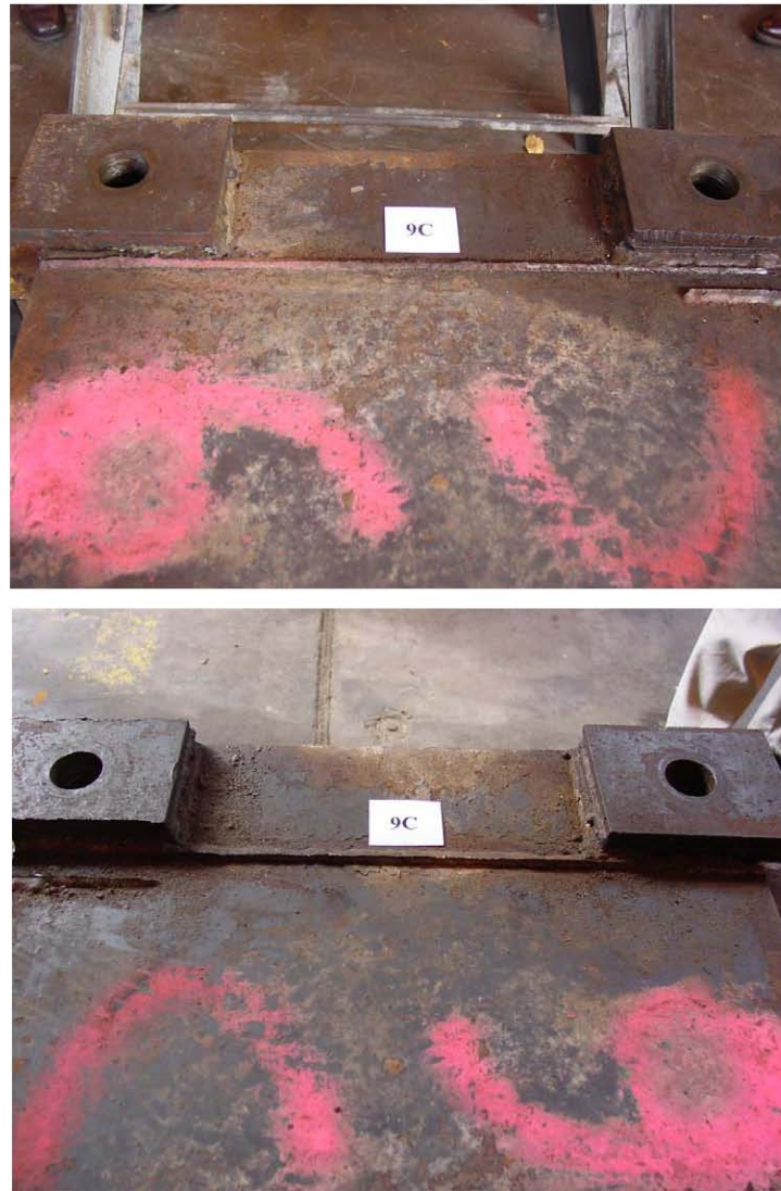
Figure 16 General Views of the Weld Fracture on Base Plate 9C.
