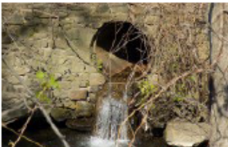
An outfall belonging to Yonkers near sentinel station S61 discharging during dry weather.
