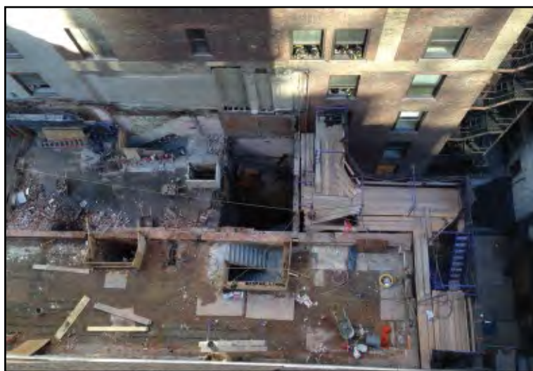
Aerial view of both buildings under demolition showing collapse in the rear section of the building.
