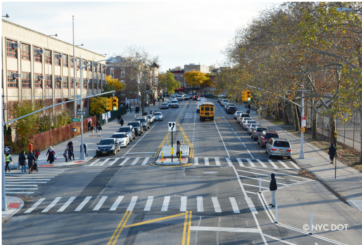
Ralph Avenue at Marion Street, Brooklyn: New traffic signal, crosswalks, pedestrian island, and painted curb extension adjacent to P.S. 40 George W. Carver.
