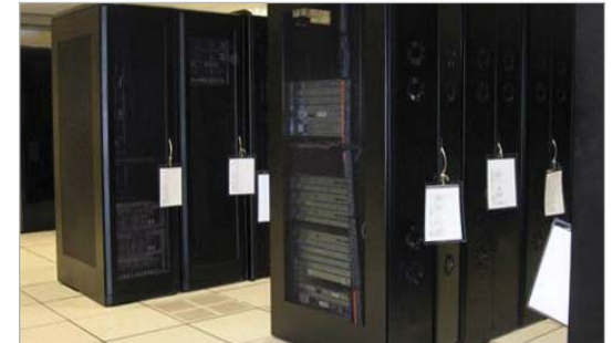
Providing space, storage and power.
