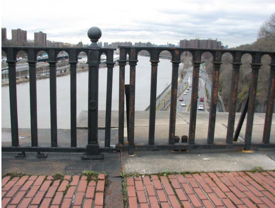
FIGURE 23. Elevation view of the transition between the 1928 railing (left) and the 1864 railing (right). Note the change between metal copings and granite copings and the metal expansion joint.
