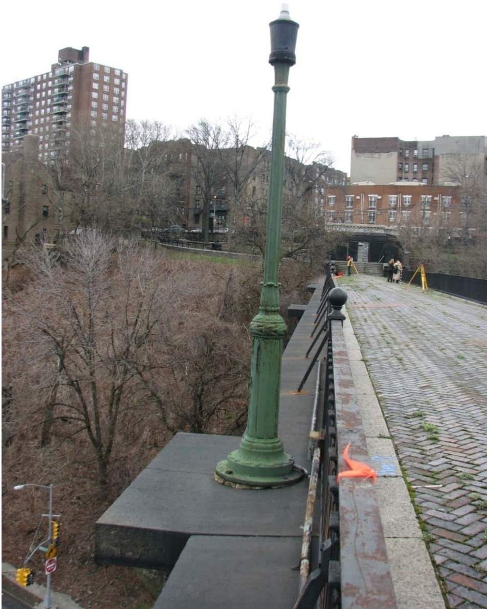
FIGURE 29. View an historic light pole mounted to a pier of a masonry arch on the Bronx side of the walkway
