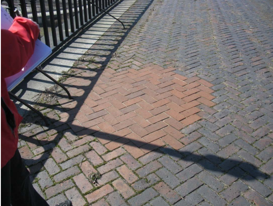
FIGURE34. Detail view of an existing bridge deck opening covered with a with a non-historic patch
