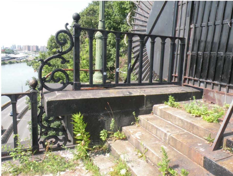
FIGURE 31. View of the 1864 railing and decorative metal scroll work with 1935 light pole at beyond at Manhattan steps.
