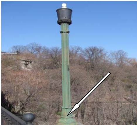
Photo LCM #5: Light green paint over orange primer present on seventeen (17) old abandoned light poles along the sides of the walkway.
