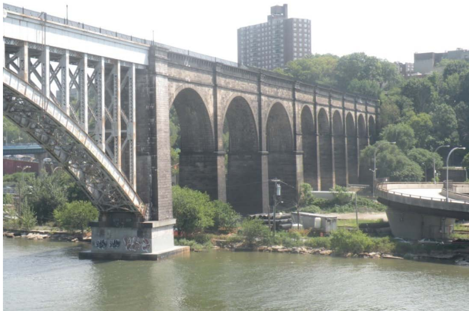
FIGURE 3. View of the south elevation of the metal arch and masonry arches looking toward The Bronx
