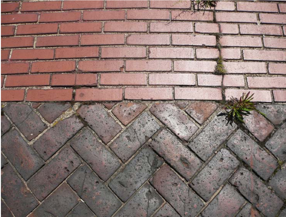
FIGURE 312. Detail view of the transition between the 1864 brick paving and the 1928 Brick paving.
