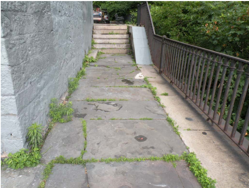
FIGURE 28. View of bluestone pavers and granite steps at north side of gatehouse
