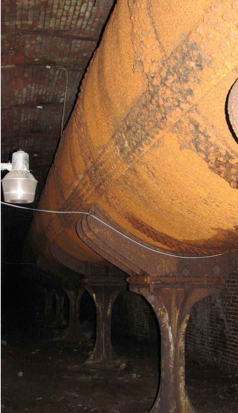
FIGURE 36. Interior view of the aqueduct supported on pedestals at the masonry attic.
