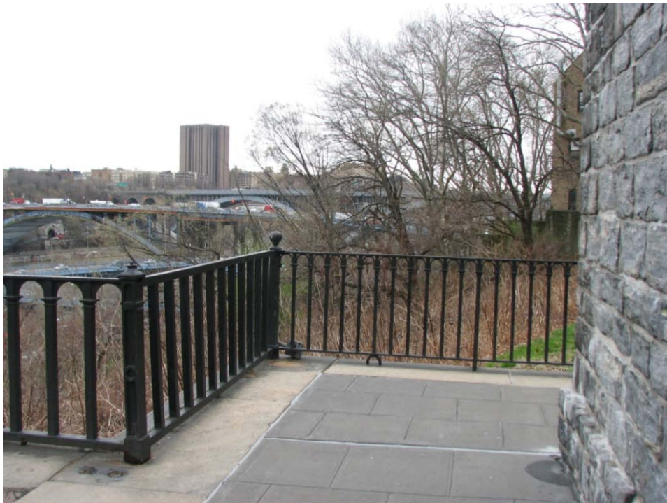
FIGURE 20. Detail view of the 1864railing (left), the non-historic in-fill railing (center), and the 1850(right) and 1864 railing (right) at the Bronx gatehouse plaza. Note the variance in picket spacing and formation of the arches.
