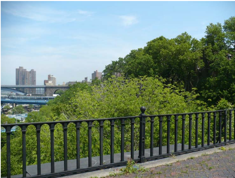
FIGURE 22. Elevation view of the 1868 railing and granite copings at masonry arches on the Bronx end of the walkway.
