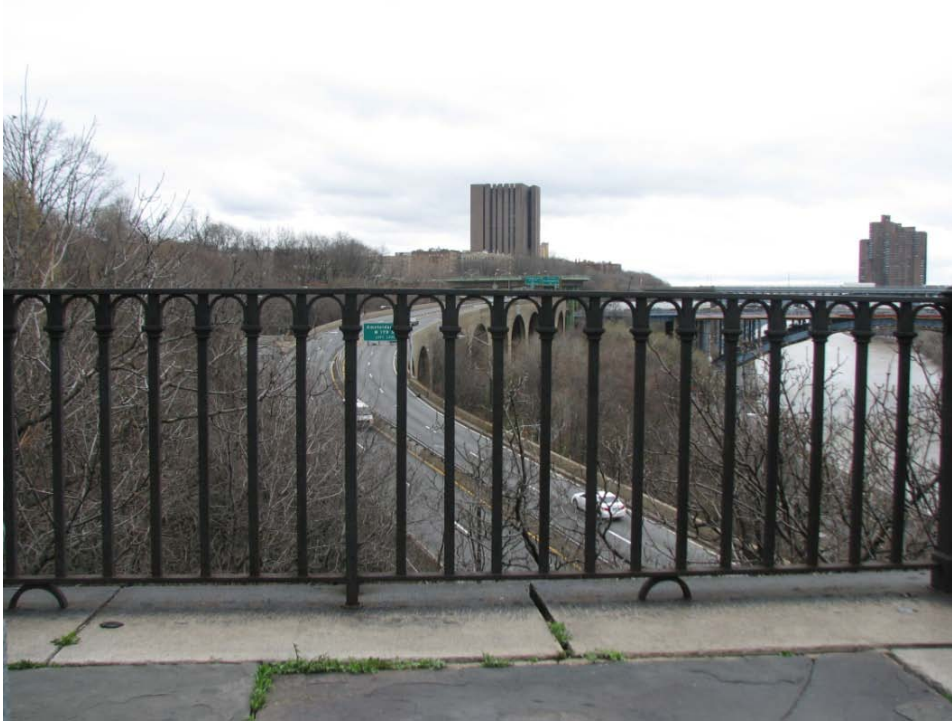
FIGURE 21. Elevation view of the 1850 railing and granite copings at the Manhattan gatehouse plaza.
