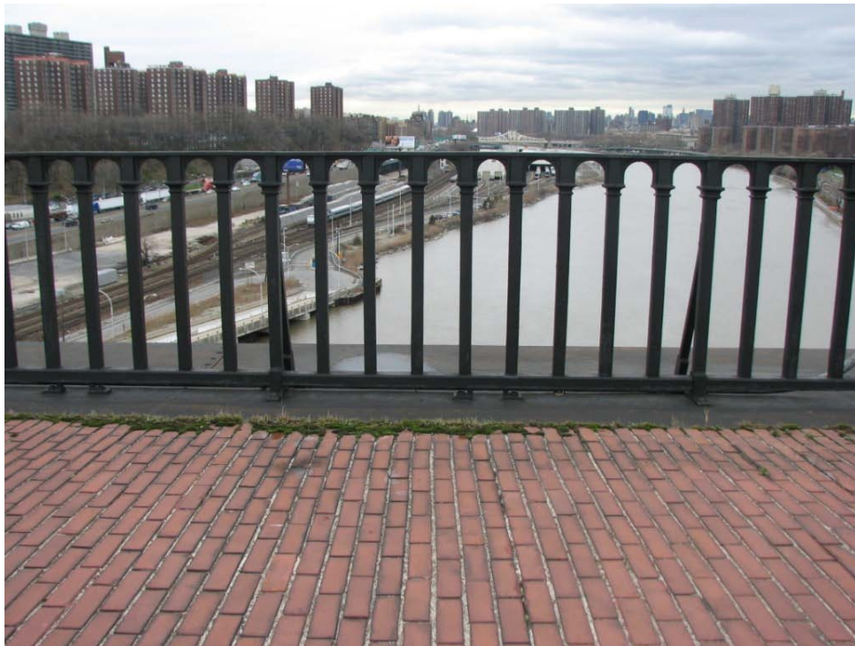
FIGURE 24. Elevation view of the 1928 railing and metal copings at the metal arch section of the walkway .
