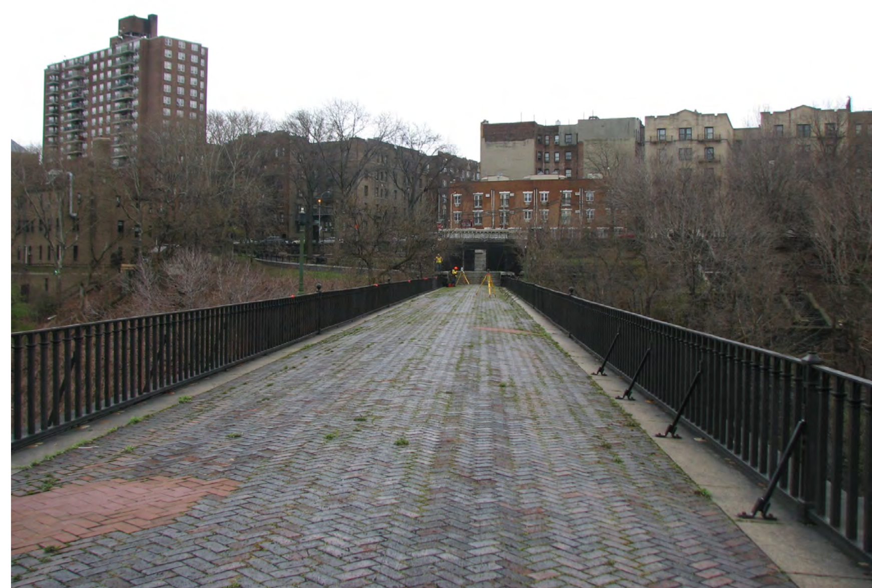
BRIDGE DECK- FACING THE BRONX Existing conduit hidden by rail
