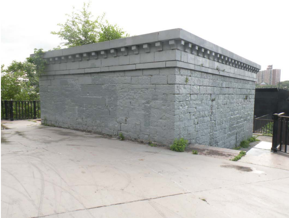
FIGURE 9. View of the west and south elevations of the Manhattan gatehouse and surrounding plaza
