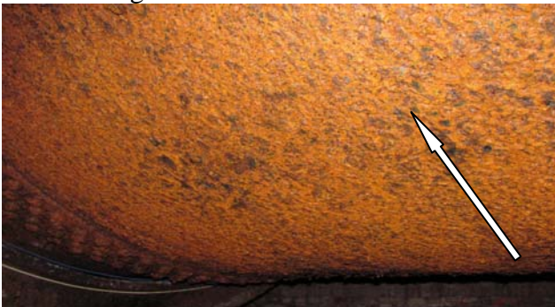
Photo LCM #3: Black coating present on 90 inch water main located in the east attic, east of pier 2.
