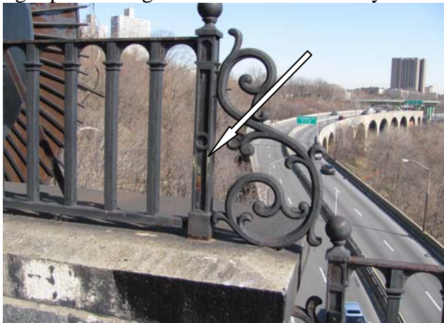
Photo LCM #6: Black over yellow over orange primer paint present on railings throughout the walkway.
