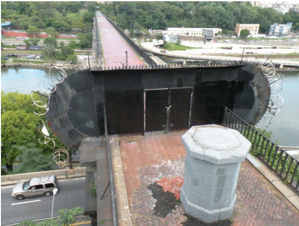
FIGURE 10. Aerial view of the Manhattan vent, vent plaza and security gate (taken from the roof of the Manhattan Gatehouse)
