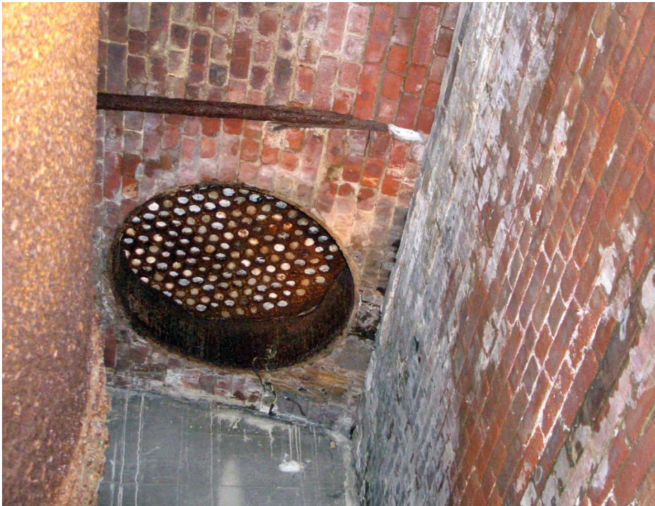
FIGURE35. Detail view of a historic vault light as seen from below in the attic.
