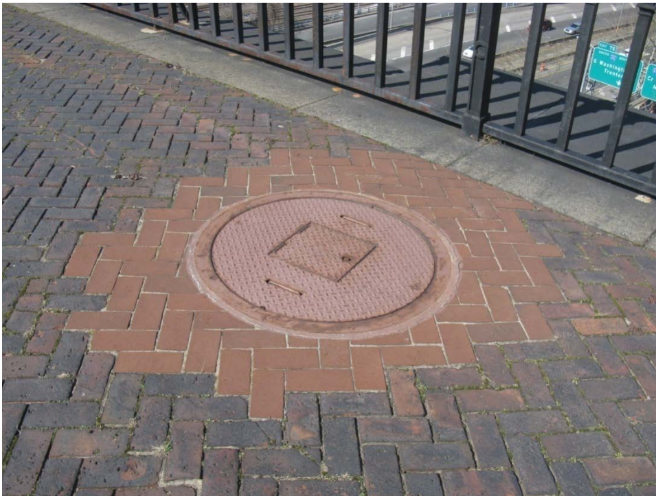
FIGURE 323. Detail view of a non-historic manhole cover has been installed at a location that previously had a vault lights. Note the surrounding non-matching brick at the area of repair.
