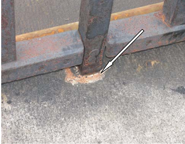
Photo LCM #10: Silver metal (lead solder) material present at railing post insets located in the vicinity of the west gate house fence (47 posts), west abutment/pier1 fence(13 posts), over pier 2 fence (10 posts) , and in the vicinity of the east gate house fence (22 posts). This includes remnant lead solder at old post holes.
