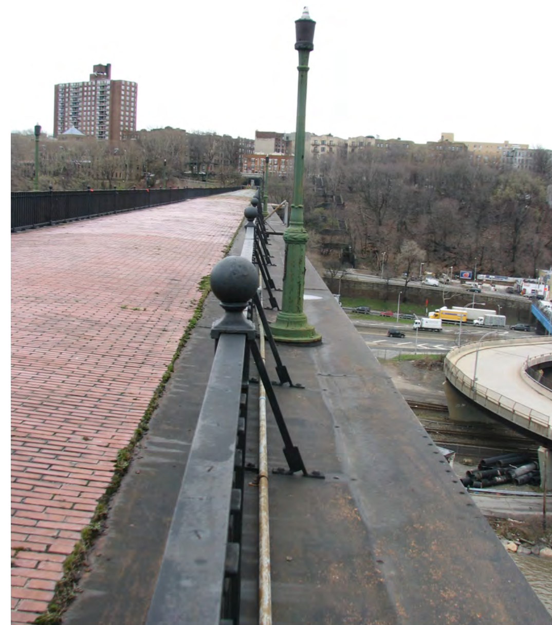
EXISTING CONDUIT AT STEEL COPING
