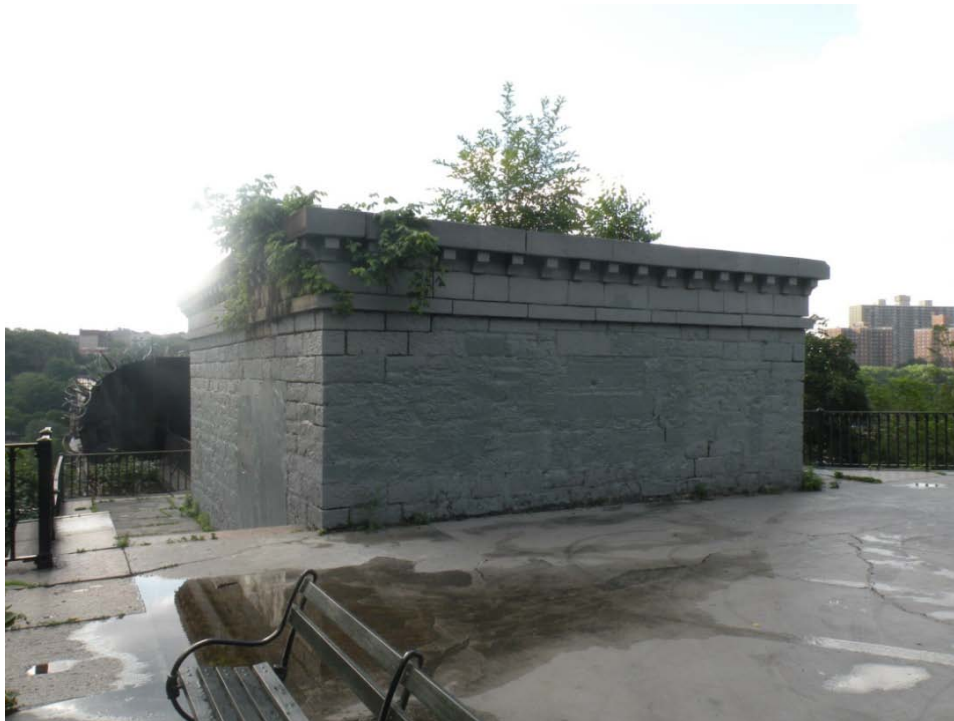
FIGURE 8. View of the north and west elevations of the Manhattan gatehouse and surrounding plaza
