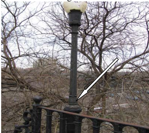
Photo LCM #9: Black over dark green paint present on one old light pole near the east security gate.
