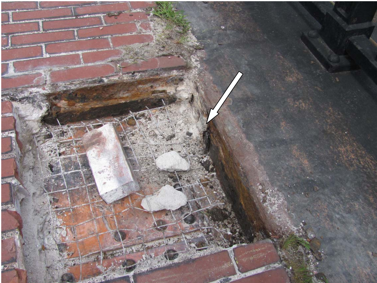
Photo ACM #1: Location of Asbestos-containing bituminous joint filler material present at joint between steel deck of bridge and the brick walkway. This material is present at the entire joint between piers 1 and 2. Note: the transverse expansion joints in the brick work contain similar joint filler materials. The transverse joint filler material was tested separately and did not test positive for asbestos.
