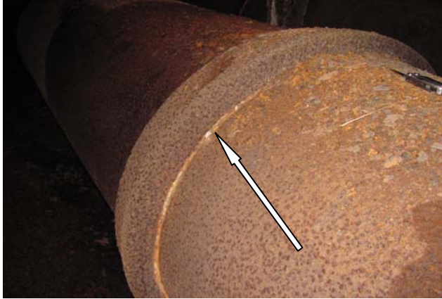
Photo LCM #4: Silver metal (lead solder) material present at bell fitting of abandoned 36 inch water mains located beneath the west abutment in the west attic. This material is also present at small diameter pipes and valves in the attic beneath the west and east gate houses.
