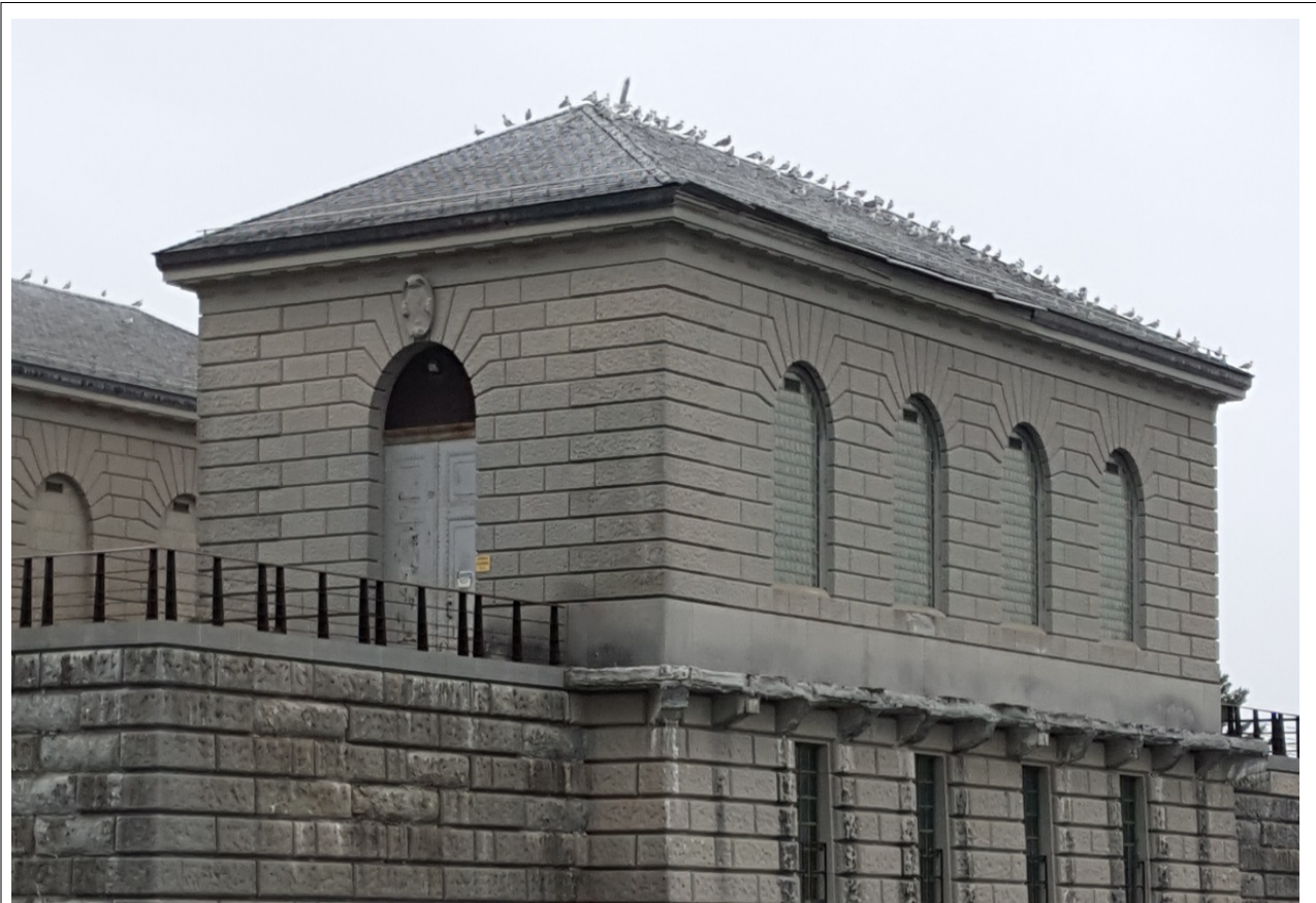
Figure 3.27. Monitoring shaft building rooftop waterbird roosting at the Ashokan Reservoir east basin.
