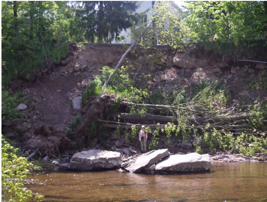
Figure 4.14 Schoharie Avenue streambank stabilization was constructed to address this laterally expanding bank failure in the Village of Hunter.
