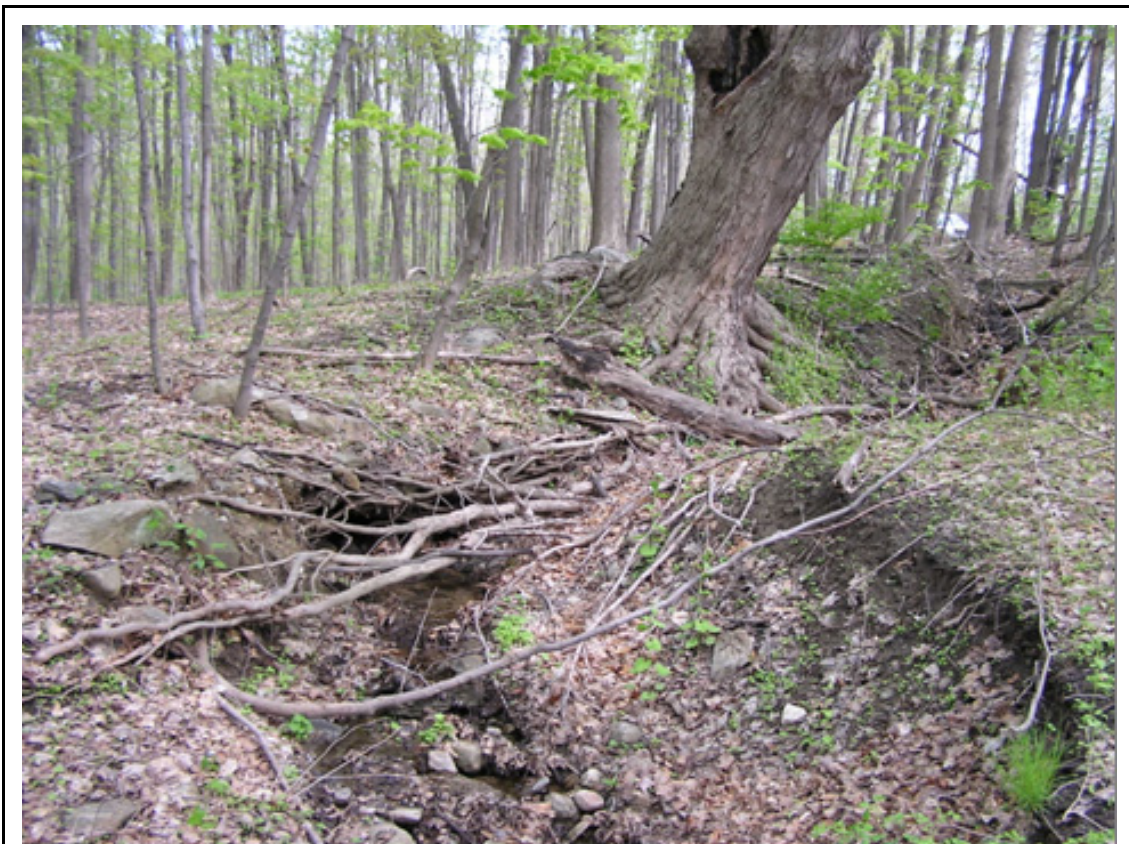
Figure 4.19 Eroded drainage ditch at Hemlock Road.
