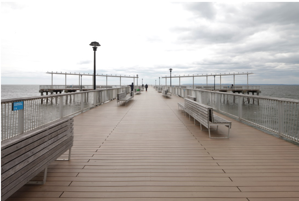
Coney Island (Riegelmann) Boardwalk , south end of Steeplechase Pier Sarah Moses (LPC), 2018
