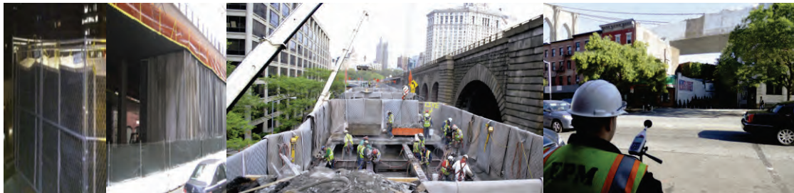
Noise Reduction Along the Sound Pathway – Acoustical Barriers on the Bridge During Night Construction Activities. Acoustical Curtains Along Frankfort Street. Two Crews Work Along Frankfort Street in April 2012. Cranes (On Left) Lift Material In And Out of Walled Enclosures of Sound Blankets. Inspector Taking Noise Measurements.
