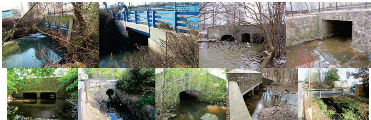
R00013 Naughton Avenue over Patterson Avenue. R00032 Seguine Avenue over Purdy Place. R00115 Victory Boulevard over Cloves Lake Park. R00114 Sweet Brook Road over Ridgewood Road. R00103 Aultman Avenue over St. George Road. R00139 De Pew Place over Maguire Avenue. R00105 Arthur Kill Road over Clarke Avenue. R00101 St. Andrews Road over Lighthouse Avenue. R00040 113 Maguire Avenue over Depew Place.
