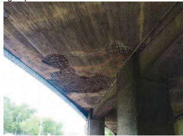
Hollow Sounding And Delaminated Concrete Areas With Exposed Rebars on the Sunrise Highway Bridge Westbound over Laurelton Parkway in 2014.
