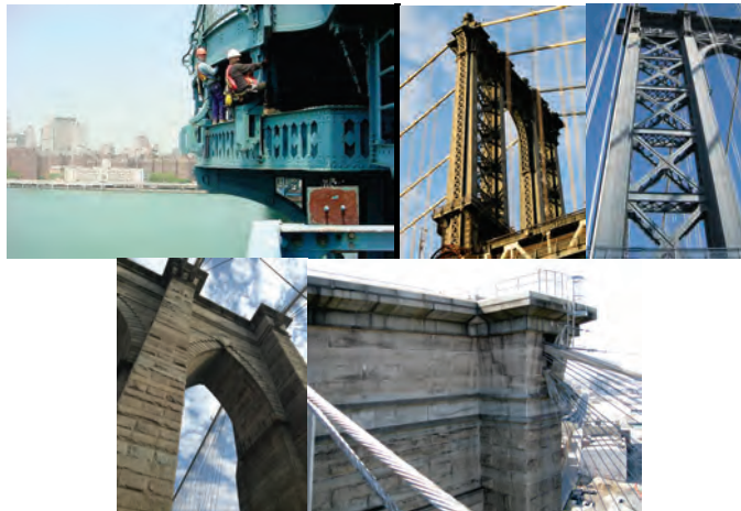
Inspectors on Manhattan Bridge Tower. (Inspector Credit: NYSDOT) Manhattan Bridge Tower. (Credit: Michele N. Vulcan) Manhattan Bridge Tower Detail. (Credit: Russell Holcomb) Brooklyn Bridge Tower. (Credit: Earlene Powell) Brooklyn Bridge Brooklyn Side Tower Detail. (Credit: Jagtar Khinda)
