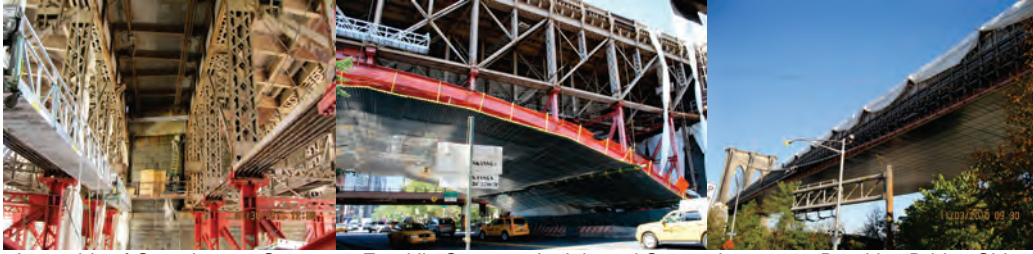
Assembly of Containment System at Franklin Square – in July and September 2010. Brooklyn Bridge Side Span Containment System – in November 2010.
