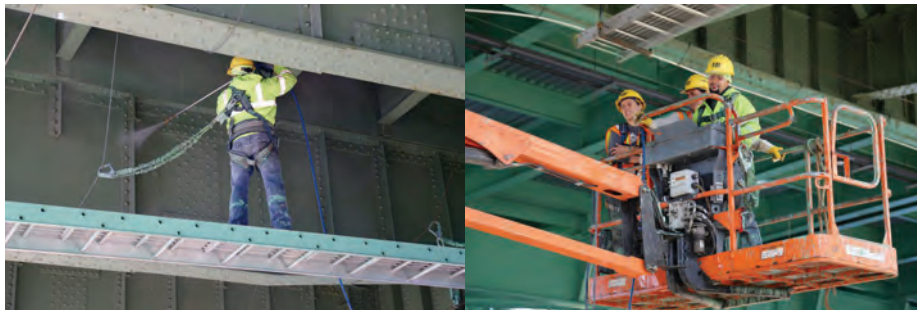
Joe DiMaggio Highway: On Scaffold - Bridge Painters Herbert Rodriguez and Reinaldo Leal. Bridge Painter Herbert Rodriguez. Bridge Painters Elisangela Oliveira, Reinaldo Leal and Herbert Rodriguez. (Credit: Jaclyn Jablkowski)
