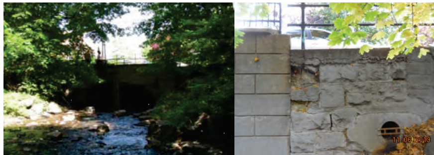
Forest Avenue Bridge Over Clove Lakes Park Stream. End Right Wingwall. (Wingwall Credit: NYSDOT)
