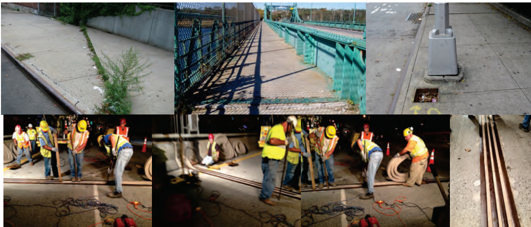
August, October, and November 2008: Examples of Tripping Hazards. July 2013 Safety Flag: Ironworker and Mason Crews Repairing Missing Joint Seal Materials on the Brooklyn-Bound Williamsburg Bridge. The Joint Sealer Spaces Were Widened on Each Part of the Joint Utilizing the Shop-Made Jack Expansion Blocks, and Then Completely Cleaned With a Needle Gun to Prepare the Surface to be Rough Contacted With Epoxy Glue. After the Glue was Spread on the Sealer Space Surfaces, the Seal Strip was Installed and Tightened. (Credit: Hany Soliman)
