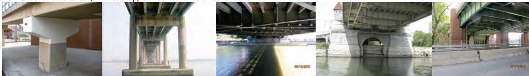
Pier 1 (Looking Southeast) of Minthorne Street Pedestrian Bridge. Pier 17 of Rikers Island Bridge. Pier 2 of Broadway Bridge. Pier 35 of Macombs Dam Bridge. (Credit: NYS DOT) Pier 1 (Looking East) of Hutchinson River Parkway Bridge over Hutchinson River.
