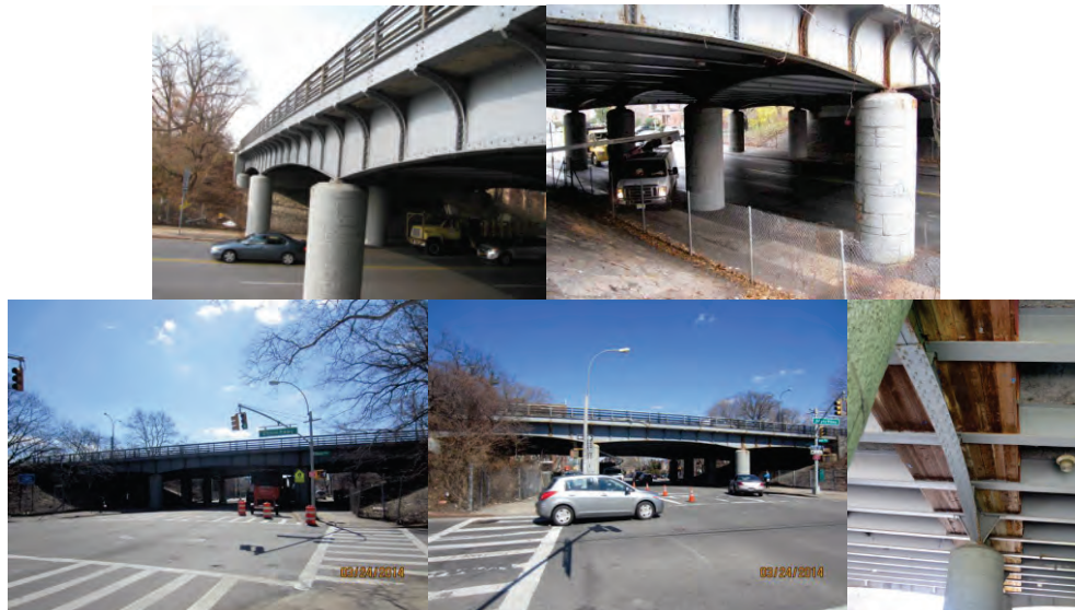
Nostrand Avenue Bridge Right Girder in November 2012. Pier 1 and 2 Columns in December 2014. Left and Right Elevations in 2014. Span 1 Deck – Hollow Sounding Concrete Areas are Covered by Timber Planks That are in Good Condition. (2014 and 2015 Credit: NYSDOT)
