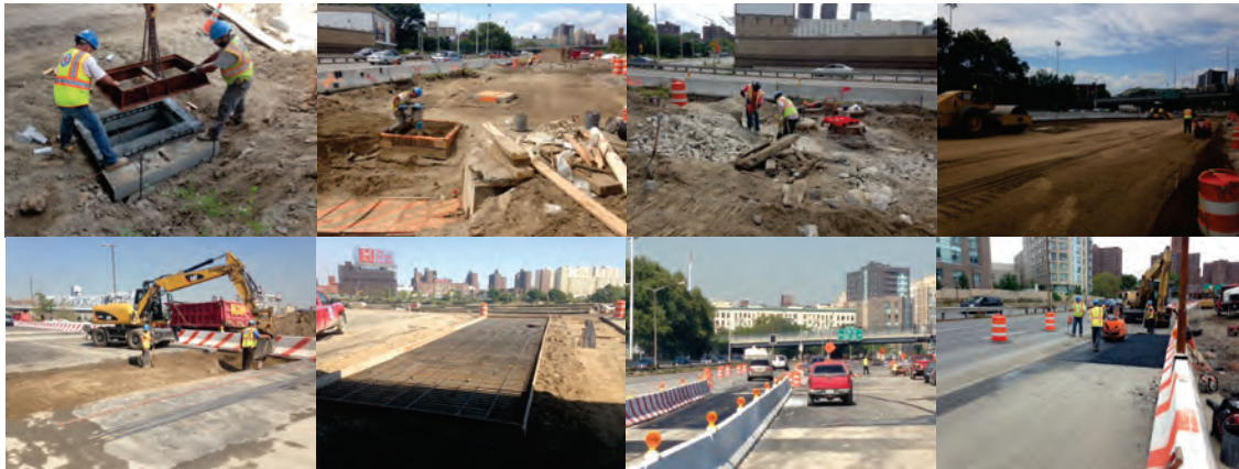
August 2015: Backfilling Utilities at Second Avenue. Contractor Working on the Temporary Roadway Placing the Sub-Base Second Layer. September 2015: Preparing New Concrete Crane Pads With Reinforcement. Painted Concrete Barriers Near Ramp C and Temporary Roadway. October 2015: Adjusting the Grading on the New Temporary Roadway. (Credit: Artemio Angeles)
