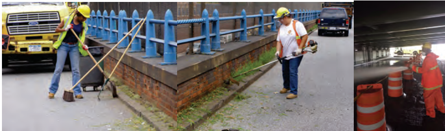
Assistant City Highway Repairer Lashawn Elam and Highway Repairer Anita Ramos Removing Vegetation and Other Debris. Assistant City Highway Repairer E'boni Brown Removing Debris under the Henry Hudson Parkway at 58 th Street. (HHP Credit: Edward Pedersen)
