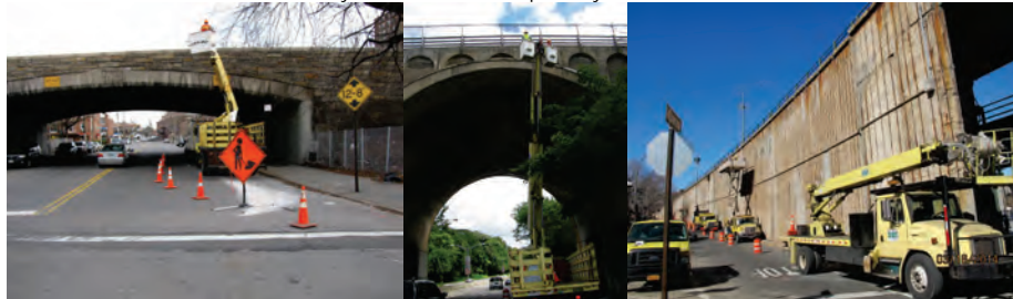
Inspecting the Belt Parkway Bridge over 26 th Avenue in December 2012. (Credit: Artemio Angeles) Inspecting the Nereid Avenue Bridge over Bronx River Parkway in June 2012, Using a 60 Foot Boom With Outriggers. (Credit: Bojidar Yanev) Inspecting the Brooklyn-Queens Expressway (Eastbound) over Cadman Plaza/Brooklyn-Queens Expressway (Westbound).
