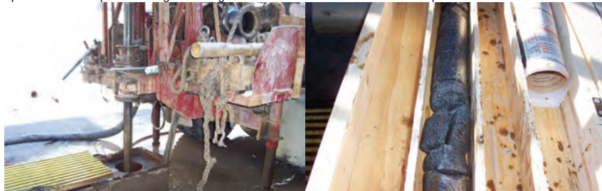
Conducting Soil Borings in 2008 as Part of the Seismic Retrofit Design of the Manhattan Bridge. Drilling to a Depth of Approximately 210 Feet to Obtain an 8-foot Long Hard Rock Sample. A 2 1/2 – Foot Long Hard Rock Sample Taken From a Depth of Between 202 and 204 1/2 Feet.
