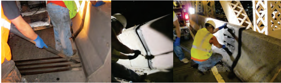
Expansion Joint Cleaning on the Williamsburg and Ed Koch - Queensboro Bridges in September 2011. (Credit: Shaikh Islam)
