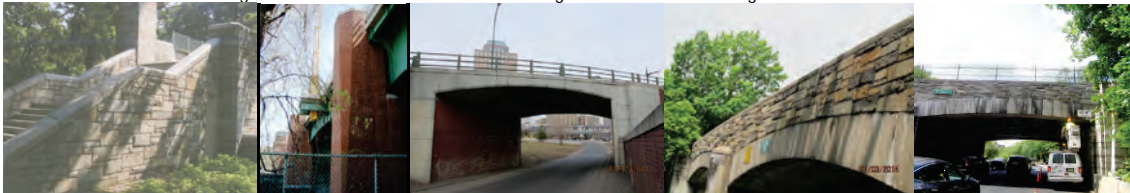
Abutment Wingwall Cladding on the West 173 rd Street Bridge. Hutchinson River Parkway Bridge. Brooklyn-Queens Expressway Over Ramp to Brooklyn-Queens Expressway (Eastbound). Right Side Fascia on the Bronx Pelham Parkway Bridge. Inspecting the Cladding Stones of the Fascia of Span 1 on West 252 nd Street Bridge Over Henry Hudson Parkway.
