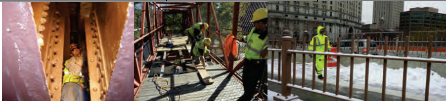
Bridge Repairer Riveter Damian Venezia Squeezing Between the Girders to Access a Floor Beam That Needed to be Reinforced on the Ed Koch Queensboro Bridge – August 2010. (Credit: Hany Soliman) Carpenters John Horgan and Ruben Urena, and Assistant Civil Engineer Fouad Althaibani Repairing the PS-5 Bridge in November 2011. (Credit: Thomas Whitehouse) Cement Mason Victor Porowski Spreading Sodium Acetate on the Walkway of the Brooklyn Bridge in 2013. (Credit: Paul Schwartz)
