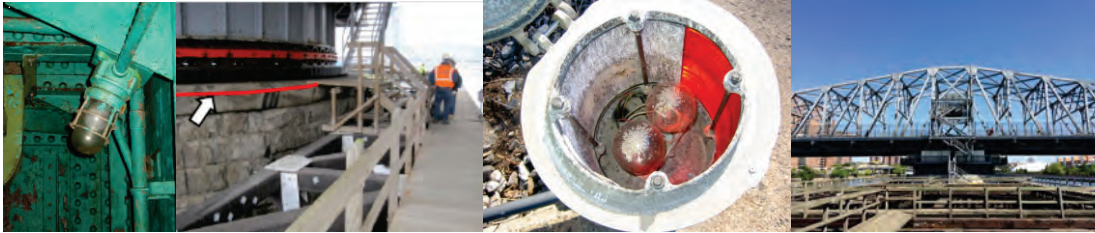
Inspection in Late 2012: Grand Street Bridge – Standing Water in the Access Light Fixture at the East Wedge Walkway. Union Street Bridge – Standing Water in East Span Maintenance Light. Madison Avenue Bridge - General View of Fender and Center Pier—the Red Line Depicts the Approximate Water Level. Macombs Dam Bridge – Pier Lighting Fixture with Cover Removed – Silt Deposit on Lamp Tops, and Corrosion on the Fixture Frame. 145 th Street Bridge in August 2015. (Credit: Lity Barreto)
