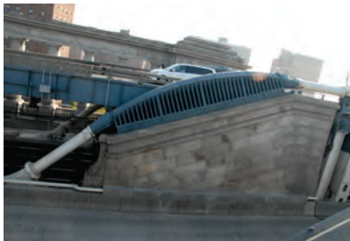
Manhattan Bridge Saddle. (Credit: Jagtar Khinda)
