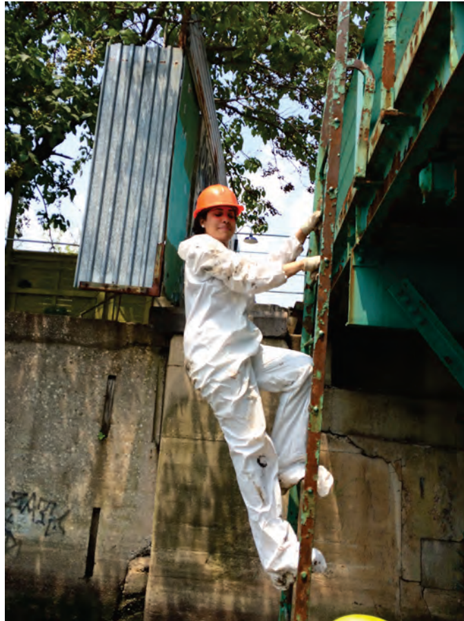
Summer College Intern Litzy Barreto on the Third Street Bridge During Strain Gauge Installation in July 2015. (Credit: Vera Ovetskaya)
