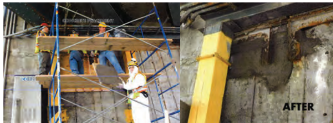
December 2015: Patching a Spall on the Beginning Abutment Stem of Brooklyn-Queens Expressway (Westbound) over Cadman Plaza.
