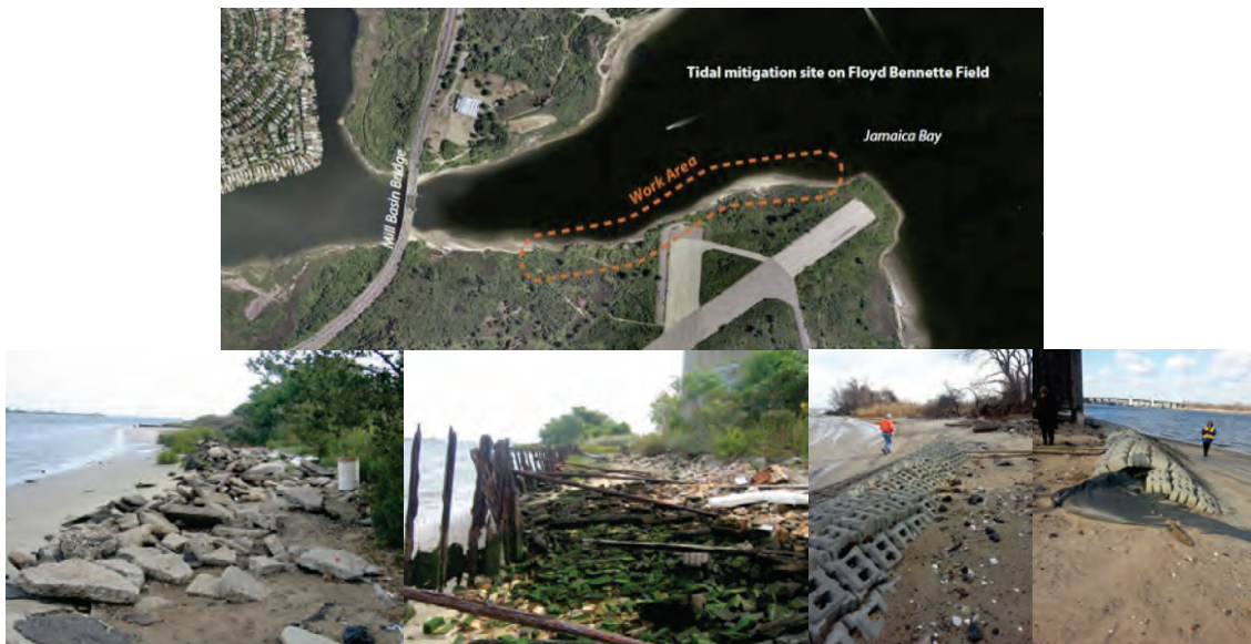
Tidal Wetland Mitigation Site. Before Mitigation – Large and Heavy Surface Debris and Deteriorated Bulkhead. Inspecting the Hurricane Sandy Damage at the Site in January 2013.
