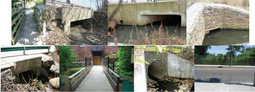
Galloway Avenue over Marianne Street – Wearing Surface, Looking Northwest. Forest Avenue over Crystal Avenue. Midland Avenue over Hylan Boulevard – Looking South. Rockland Avenue over Brielle Avenue. Forest Avenue over Randall Avenue. Gregg Place over Randall Avenue. Arthur Kill Road over Muldoon Avenue. Arthur Kill Road over Ridgewood Avenue.
