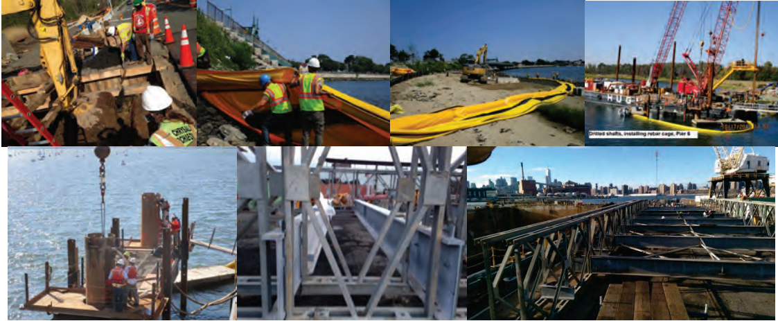
August 2014: Excavating on the West Side of the Bridge in the Presence of an Archeologist. Approximately 300 Linear Feet of a Turbidity Curtain was Installed on the Southwest Side of the Bridge to Protect the Shore During Construction. A Turbidity Curtain is a Floating Barrier Designed to Contain and Control the Dispersion of Sediment. October 2014: Drilled Shafts – Installing Rebar Cage at Pier 6. October 2014: The Contractor Airlifted Drilled Shaft Casings Into Position on a Platform Constructed Beside a Construction Barge. The Contractor Assembled the Temporary Bridge Segments at the Brooklyn Navy Yard. The Pieces Were Transported to City Island by Barge.
