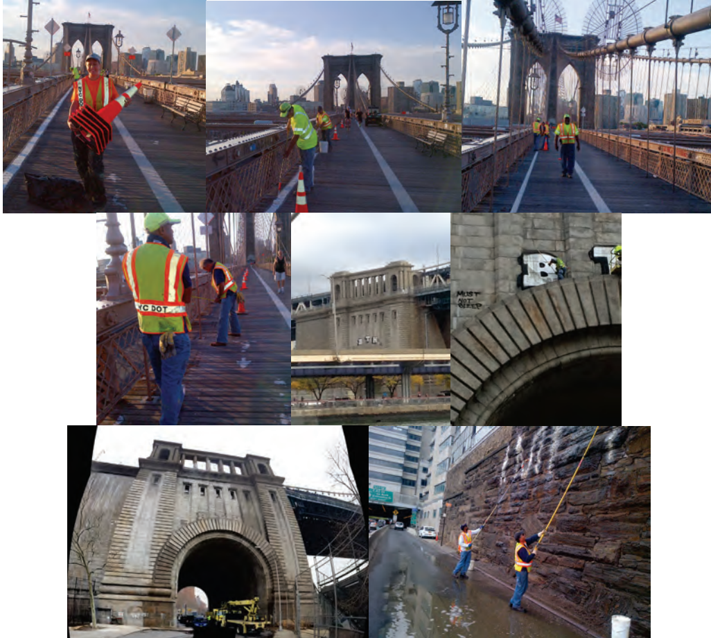
August 2015: Brooklyn Bridge Line Striping. Bridge Painter Elisangela Oliveira. Bridge Painters Arlindo Lima and Carlos Mata. Bridge Painter Willie Tyler Checking the Striping. Bridge Painter Gerson Do Rosario and Supervisor Bridge Painter Cesar Pazmino. (Credit: Earlene Powell) March 2015: Supervisor Bridge Painter Goncalo Lima Removing Graffiti on the Manhattan Bridge Arch on Cherry Street. (Credit: Cesar Pazmino) July 2015: Bridge Painters Gerson Do Rosario and Carlos Mata Removing Graffiti on the FDR Drive.
