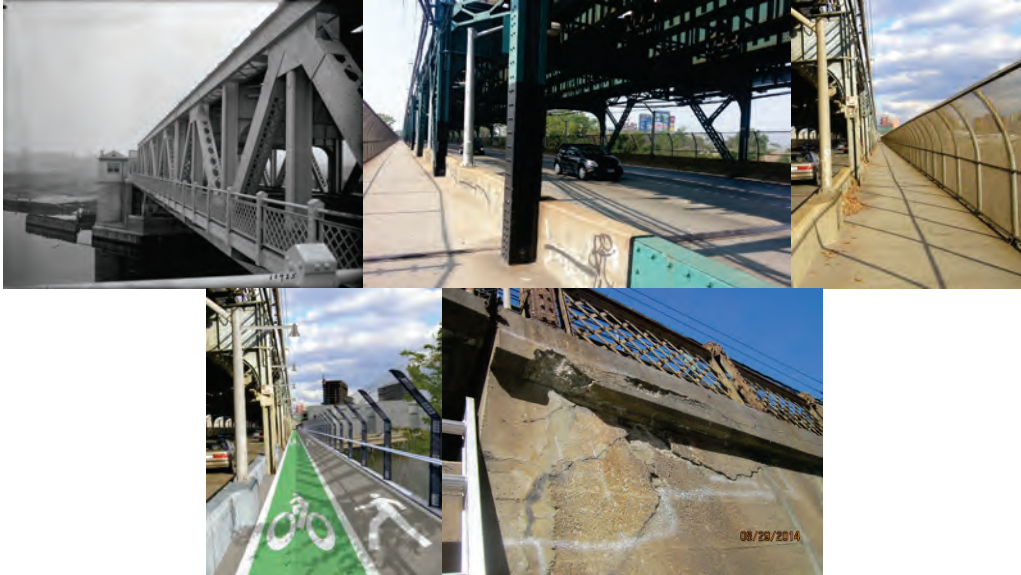
Roosevelt Avenue Bridge – In 1927. (Credit: NYC Records). Looking East. Existing and Proposed Bicycle/Pedestrian Path. 2014: Right Wingwall at the End Abutment. The Top Exhibits an area of Diagonal Cracks With Efflorescence and Spalls. The Deteriorated Concrete Areas are in Safe and Stable Condition. (Credit: NYSDOT)
