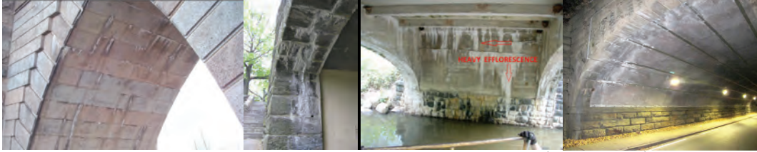
Moderate Efflorescence on the Brooklyn Bridge Brooklyn Tower North Gothic Arch in 2004. (Credit: NYSDOT) Efflorescence on the Underside of the Masonry Stones on the End Abutment of the Margaret Corbin Drive Bridge over Pedestrian Path Near Café. Heavy Efflorescence on End Abutment Stem Wall of Bridge Over Dam at Clove Lake in 2014. Efflorescent Stains on the Shielding of Span #1 of the East Drive Bridge over Transverse Road #3 in 2015.
