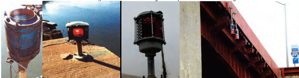
Northern Boulevard Bridge - Bridge and Pier Marine Navigational Lighting. Grand Street – Left Side Channel Light. Pulaski Bridge - Center Lights at Span #26.
