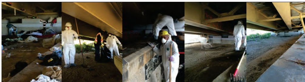
October and December 2015: Highway Repairer Abibi Ocampo Guevara Removing Debris Collected by Vagrants Under the Willis Avenue Bridge.
