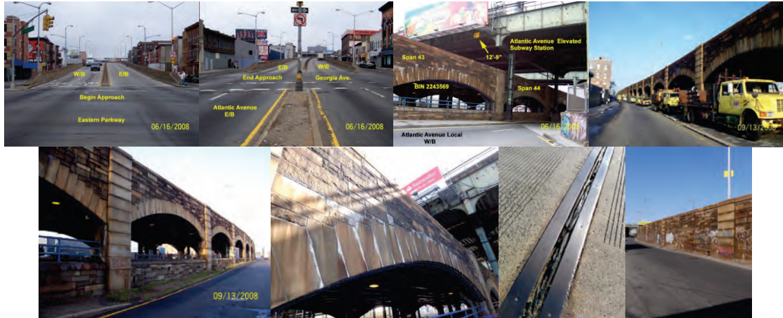
Beginning and End Approaches. Elevation Right – Spans 43 – 44. Elevation Left Spans 38 -43 and Elevation Right Spans 20 – 34. (Credit: NYSDOT) Span 43 South Arch Shows Typical Efflorescence at Mortar Joints of Ring Stones. Deteriorated and Leaking Seal at Expansion Joint. Stone Curtain Wall.
