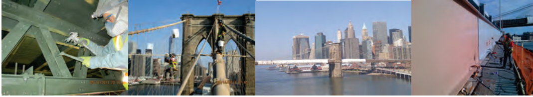
May 2013: Painter Applying Primer Stripe Coat on the Manhattan Main Span. June 2013: Painter on Sway Bracing on the Brooklyn Side Span. (View Credit: Earlene Powell) November 2013: Painting Fascia Steel on Ramp C.
