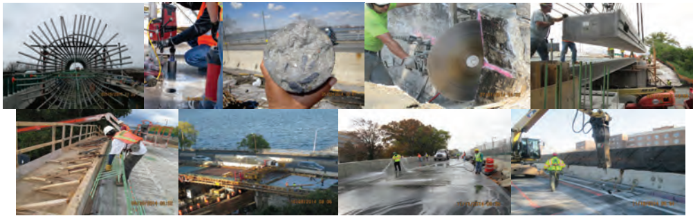
March 2014: Rebar Cage. May 2014: Core Sampling. July 2014: Saw Cutting the Existing Northwest Abutment. August 2014: Lowering the Last of the Seven Pre-cast Concrete Box Beams on the North Side Abutments. September 2014: Placing Rebar for the North Parapet. October 2014: The Main Bridge Deck Undergoing Wet Cure. November 2014: Washing the New Westbound Concrete Deck Prior to the Placement of the Temporary Barrier at Left Side Before Stage III Traffic Shift. Facing East. Demolition of the Saw Cut Westbound Bridge Deck During Stage III.
