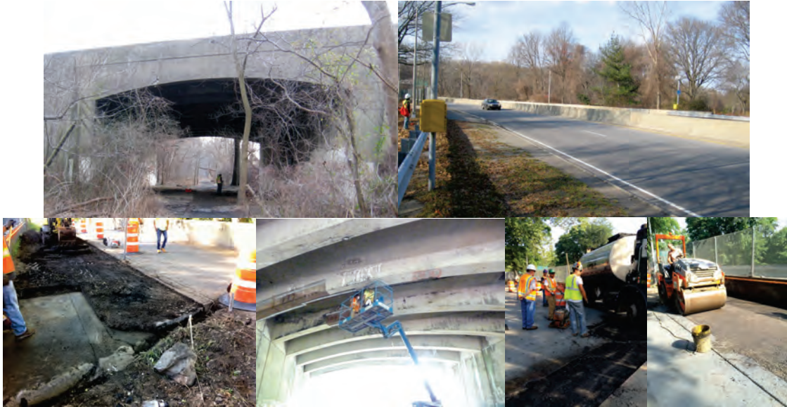
Mosholu Parkway Bridge over Conrail (Abandoned). Conditions in June 2015. Asphalt Work in July.
