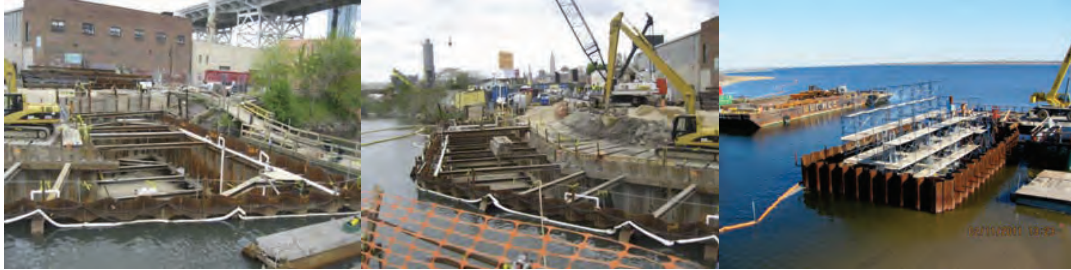
April 2010: Cofferdam With Filter Fabric and Gravel Placed Prior to Pile Driving During the Emergency Repair Project on the Borden Avenue Bridge over Dutch Kills. February 2011: Fresh Creek Cofferdam Pad.
