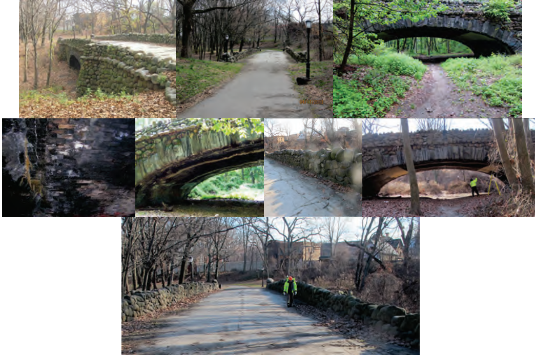
Highland Park Bridge. Dirt Pathway Under Bridge. Under-Deck Cracks and Missing Bricks - North-East Side. Under-Deck Arch Wall Showing Efflorescence Along the Cladding Stone and Brick Arch. Top of Bridge - Map Cracking, spalled, and Patched Areas. Inspecting the Bridge in December 2014.
