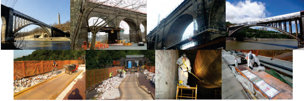
Northern View of High Bridge in 2013. Early Spring 2013: Temporary Work Platform on the Bridge. Temporary Work Platform on Sedgwick And Undercliff Avenues. Spring 2013: Mast Climber and Lead Abatement Containment on the Bridge. Summer 2013: Brick Paver Removal and Preservation. Fall 2013: Aqueduct Pipe Preservation. Reconstruction of the Walkway. (Credit: NYCDDC)
