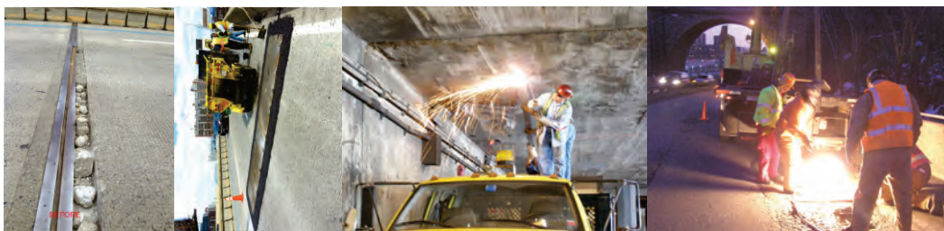
August 2014 PIA Safety Flag: Broken Joint Concrete Header And Steel Armor on the Long Island Expressway over Dutch Kills Creek. The Condition Was Made Safe By Installing Two Steel Plates. PIA Flag (Truck Wedged Under the FDR Drive at Span 41): Removing the Debris. (Credit: Victor Sandoval) PIA Flag Repair (Through Hole) on Harlem River Drive Ramp. (Credit: Bojidar Yanev)
