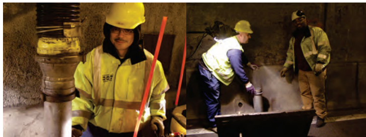
Drain Crew: Highway Repairer Anthony Irizarry, Supervisor Highway Repairer Michael Parise, and Assistant City Highway Repairer Giovonni Caballero. (Crew Credit: James Campbell)
