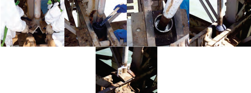
Cleaning and Lubricating the Solid Rods' Suspender Bearings on the Brooklyn Bridge.
