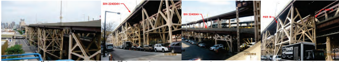
Ramp to 21 st Street From NY Over 22 nd Street. Spans 16 to 21, and Spans 22 to 38 – Right Elevation. Piers 18 and 19. (Spans and Piers Credit: NYSDOT)
