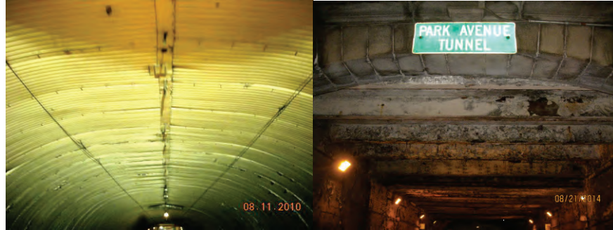
Abutment Beginning. Underside of South Arch. 2014: Framing of South Portal. (Credit: NYSDOT)
