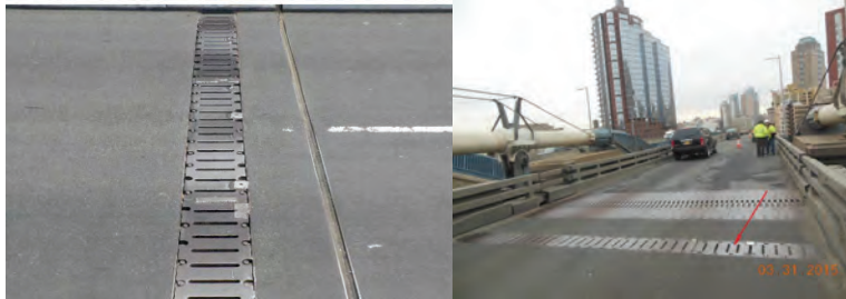
Manhattan Bridge Trench Drain.
