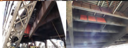
August 2013 Red Flags on the Ed Koch Queensboro Bridge. October 2013: Removing the Warped Beams. The New Beams.
