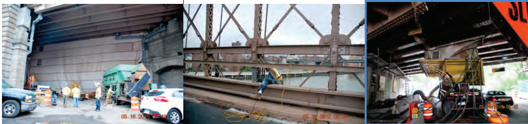
May 2015: Class 1A Abrasive Blast Containment System for the Main Street Structure Promenade Steel. Power-Tool Cleaning on Steel Repairs at the Suspended Spans. June 2015: Brooklyn Approach Structures.
