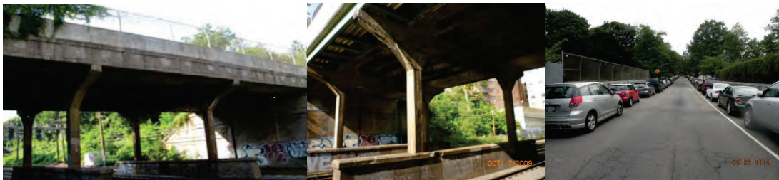
80 th Road Bridge over LIRR Main Line. Piers 1 and 2. End Approach. (Pier and Approach Credit: NYSDOT)
