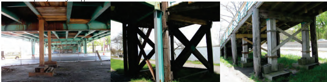
2014: Timber Shoring at Spans 7 and 8 of the Harlem River Drive over Ramp to and From Northbound Harlem River Drive. Steel Shoring of the Damaged Column at Pier 4 of the Crocheron Park Pedestrian Bridge. Timber Shoring at Piers 5 and 6.
