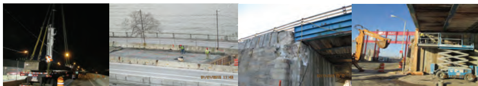
January 2015: Unloading Precast, Prestressed Concrete Box Beams During Stage III. Newly Placed Precast Box Beams in Median Area. Finished Deck From Stage II in Foreground. Existing Bridge Deck of Eastbound Roadway at Top - to be Removed in Future Stage. February 2015: Deteriorated Southwest Wingwall and Abutment of the Bridge After Dislodged Concrete Fell to the Sidewalk Below. Underdeck Timber Shielding at Right.
