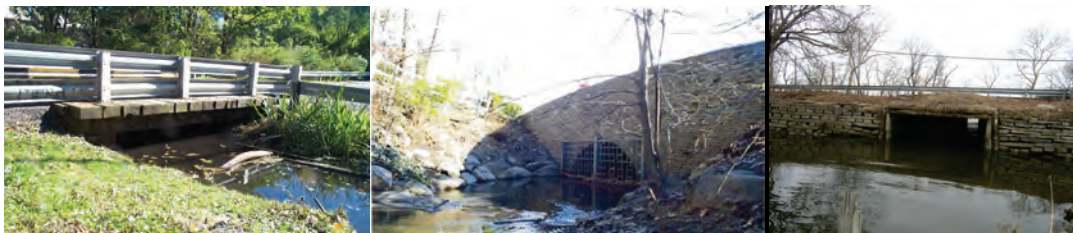
Idlesee Place Culvert. Sweet Brook Road Culvert. Richmond Terrace over Snug Harbor Culvert.
