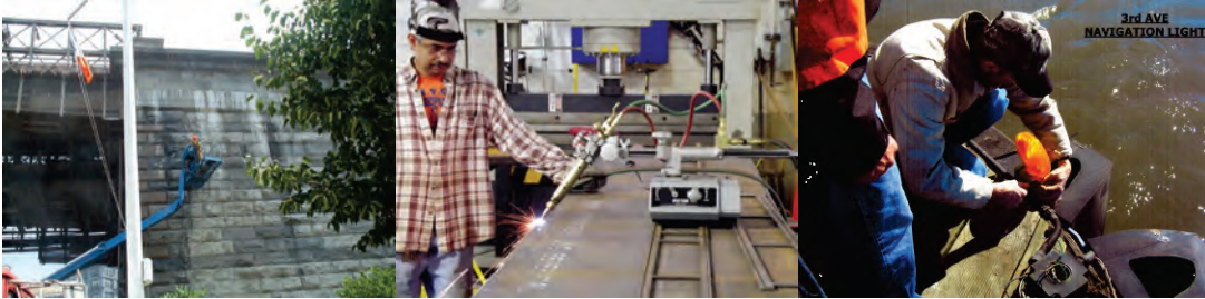
Cleaning the Brooklyn Bridge Brooklyn Anchorage in July 2007. (Credit: Serag Saad) Bridge Repairer and Riveter James Philip Using a Track-Mounted Torch to Bevel the Edge of a Steel Plate in September 2012. (Credit: Thomas Whitehouse) Checking the Navigation Lights at Pier #5 of the Third Avenue Bridge.
