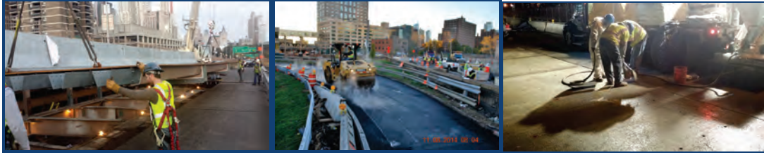
September 2014: Franklin Square Structure – New Orthotropic Deck. November 2014: Manhattan-Bound Brooklyn Approach Paving. December 2014: Super Slab Installation in Manhattan-Bound Lanes.
