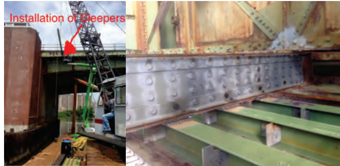
Hutchinson River Parkway Bridge - Installation of Sleeper Steel Beams to Directly Support the Steel Grating.
