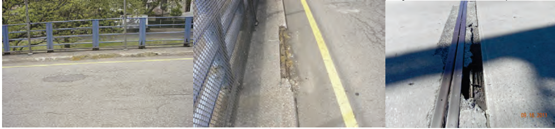
Spalled Section of Curb on the East 8 th Street Bridge in 2006. (Credit: NYSDOT) Spalling With Exposed Rebar on the Beginning Abutment Joint Header of the Westchester Avenue Bridge over the Bronx River in 2011.
