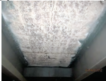
Union Street Bridge over Brooklyn-Queens Expressway in 2012 – Extensive Map Cracking With Efflorescence on the Underside of the Deck. (Credit: NYSDOT)
