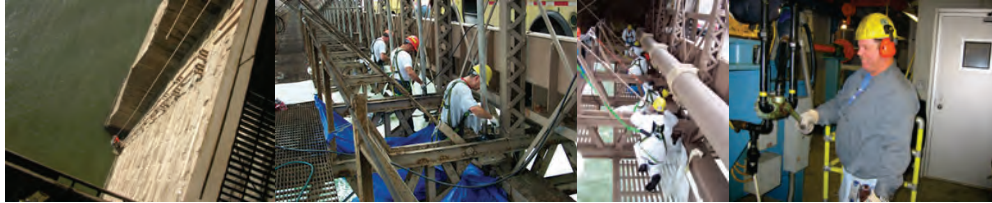
Repairing the Brooklyn Bridge Standpipe System, 130 Feet Below the Roadway. Maintenance Crew Conducting the Annual Cleaning and Lubrication of the Solid Rod Suspenders and Spherical Bearings on the Brooklyn Bridge. 2 nd Photo - Oilers Steven Marxhausen, Rene Francis, Richard Morreale, Thomas McAuliffe, and Andrew Sorrentino. (Credit: Anatoly Orlov) Oiler T. McAuliffe at the 9 th Street Bridge
