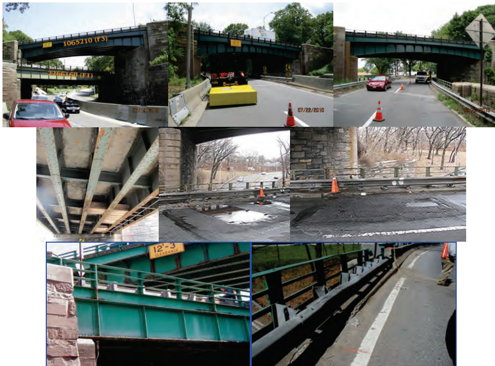
Bridge (Lower Structure) in 2010. Left and Right Elevations. (Credit: NYSDOT) August 2013: Span 1 Underside of Deck from End Abutment, Looking Northwest - Areas of Spalled Concrete Deck Are Protected With Timber Planks. March 2014: Steel Plates on Wearing Surface. South and North Fascia - Along the Fascias are Built-Up Riveted Steel Girders. The Steel Railing Posts are Welded at the Base to the Top Flange of the Fascia Steel Girders.
