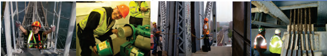
Assistant Mechanical Engineer Vera Ovetskaya Climbing to the Brooklyn Bridge Tower in 2008. (Credit: Gennadiy Kaplun) Oiler Tom Strommen Maintaining the Hydraulic Power Unit at the Hamilton Avenue Bridge in February 2010. (Credit: Vera Ovetskaya) Cleaning and Lubricating the Broadway Bridge. (Credit: Reza Taheri) Executive Director of Bridge Preventive Maintenance and Repair Thomas Whitehouse (Wearing Yellow Jacket) Inspecting the Broadway Bridge Machinery Room and Instructing the Contractor. (Credit: Albert Hong)
