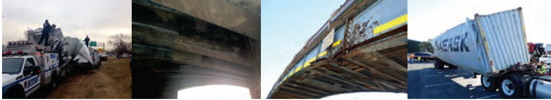
Douglaston Parkway Bridge Strike in 2015: Police Observing the Truck Damage. Underside of Bridge Concrete Beams Only Exhibited Scratches. (Credit: Artemio Angeles) 17 th Avenue Pedestrian Bridge Strike in 2015.
