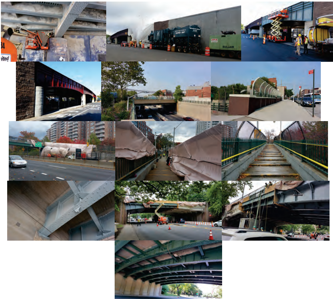
Woodhaven Boulevard Bridge over Atlantic Avenue. Associate Project Manager Vadim Sokolovsky Inspecting Site Conditions. (Credit: Vadim Sokolovsky and Sergey Parayev) Woodside Avenue over Brooklyn-Queens Expressway. West 236 th Street Pedestrian Bridge over Henry Hudson Parkway. Henry Hudson Parkway over Broadway. (Credit: Vadim Sokolovsky)
