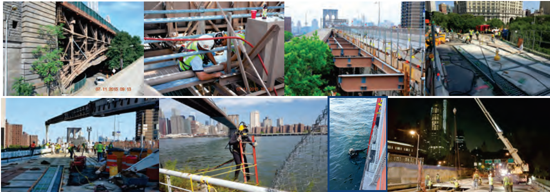
July 2015: Franklin Square Structure Seismic Retrofitting. Ironworkers Install New Railings and Toe Boards for the Inspection Catwalk Under the Promenade. New Steel Beams Installed Across the North Cantilever. This allowed for a New Grid Deck to be Set on the Manhattan Approach. Additional Deck Work was Added During a Full Weekend Closure in July to Ensure a Seamless Transition to the Two Lane Off Ramp to the FDR Drive and Pearl Street. August 2015: Concrete Closure Pours on the Manhattan Approach During a Full Weekend Closure. Diver Inspects the Fender System at the Brooklyn Tower. September 2015: Park Row Bridge – Westbound Stage II Deck Replacement.
