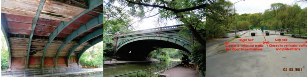
Hill Drive Bridge Span 2 Pier 1 End Face in 2013. View of Bridge in 2012. End Approach in May 2011: The Bridge is Closed to Vehicular Traffic. The Left Half of the Bridge is Closed to Pedestrians. (Credit: NYSDOT)
