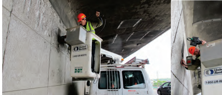
June 2015: Director of Bridge Management Kevin McNulty Inspecting the Brooklyn-Queens Expressway Between Cadman Plaza and Atlantic Avenue With a Borescope. (Credit: Bojdar Yanev)
