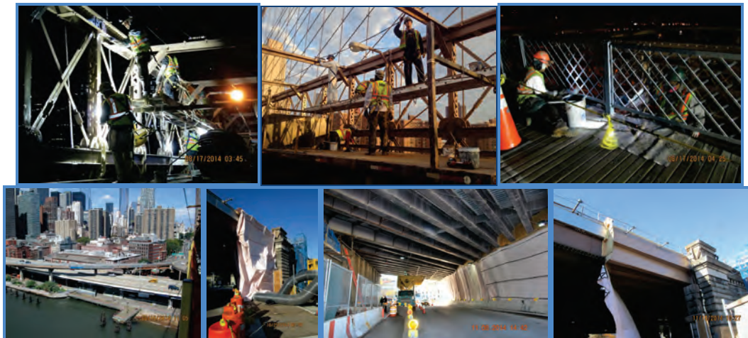
August 2014: Main Bridge Touch-Up Painting, and Painting Manhattan Main Span Promenade Railing. August 2014: Painted Manhattan Ramps. October and November 2014: Blasting and Painting – Brooklyn Approach Structures.
