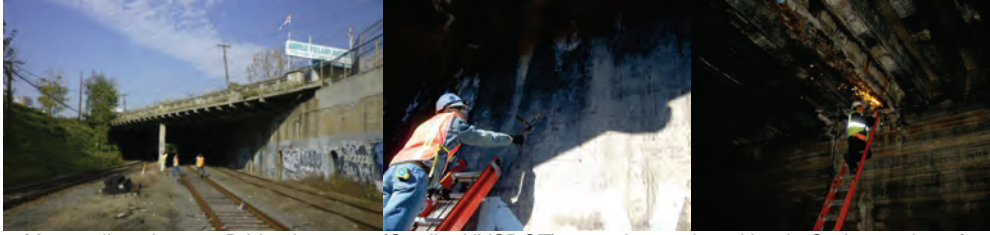
Metropolitan Avenue Bridge in 2009. (Credit: NYSDOT) 2010 Inspection - Hands-On Inspection of A Pier. Obtaining a Steel Coupon Sample From a Stringer.
