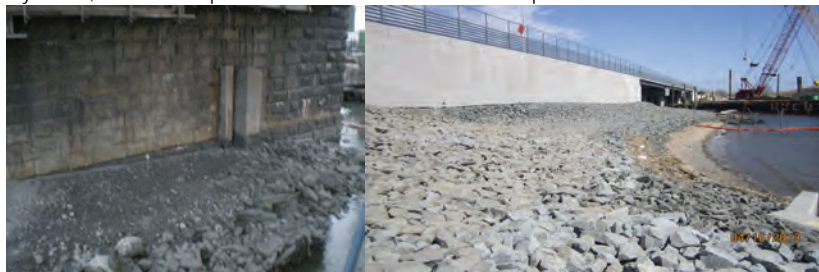
Eroded Riprap Pier Protection at Pier 11 of Old Willis Avenue Bridge in 2008. (Credit: NYSDOT) Riprap Installed in 2013 on South Side of Belt Parkway Bridge over Fresh Creek, Facing East.
