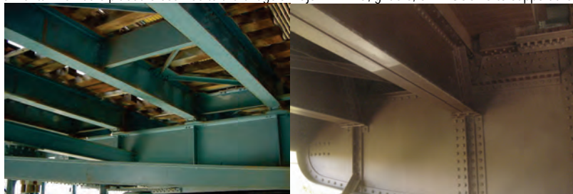
South Transit Floorbeams, Stringers, and Bracing Members on the Manhattan Bridge. Ed Koch Queensboro Bridge North Outer Roadway Floorbeam. (Credit: NYSDOT)
