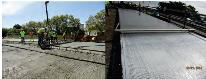
Screed at East 8 th Street Ramp in 2011, and at West Approach of Gerritsen Inlet Bridge in 2014.
