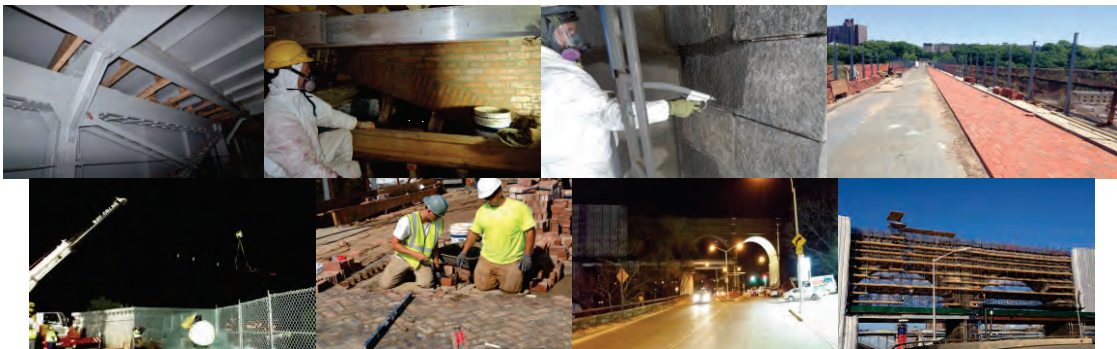
Winter 2014: Steel Stringer Installation. Spring 2014: Brick Repairs and Stone Cleaning. Summer 2014: Brick Installation. ADA Ramp Steel Installation. Summer 2014: Brick Installation. Winter 2015: LED Lighting on the Arch. Scaffolding. (Credit: NYCDDC)
