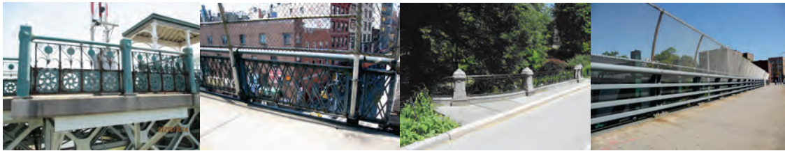
University Heights Bridge Railing. (Credit: NYSDOT) Manhattan Bridge Railing. (Credit: Russell Holcomb) Greywacke Arch Railing. 37 th Street Bridge over Brooklyn-Queens Expressway Railing.
