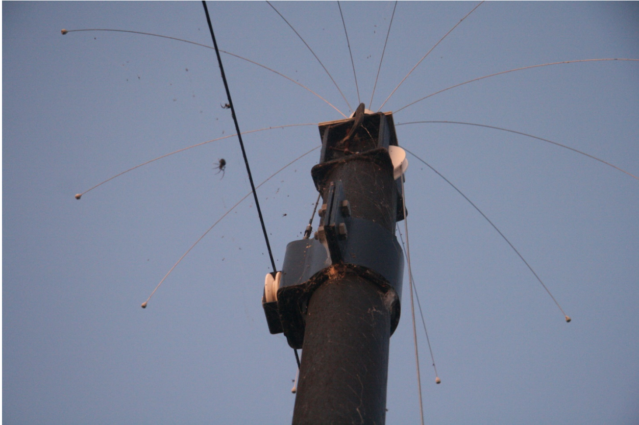
Figure 29. Overhead bird deterrent wires installed on 15' high stanchions with Daddy-Long-Legs installed to prevent waterbirds from roosting and loafing.
