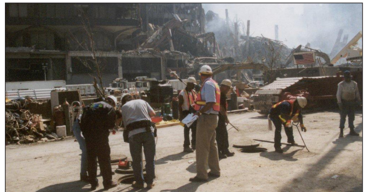
Assistant Commissioner Ed Coleman and BWSO field operations staff inspect damage to the water and sewer infrastructure.
