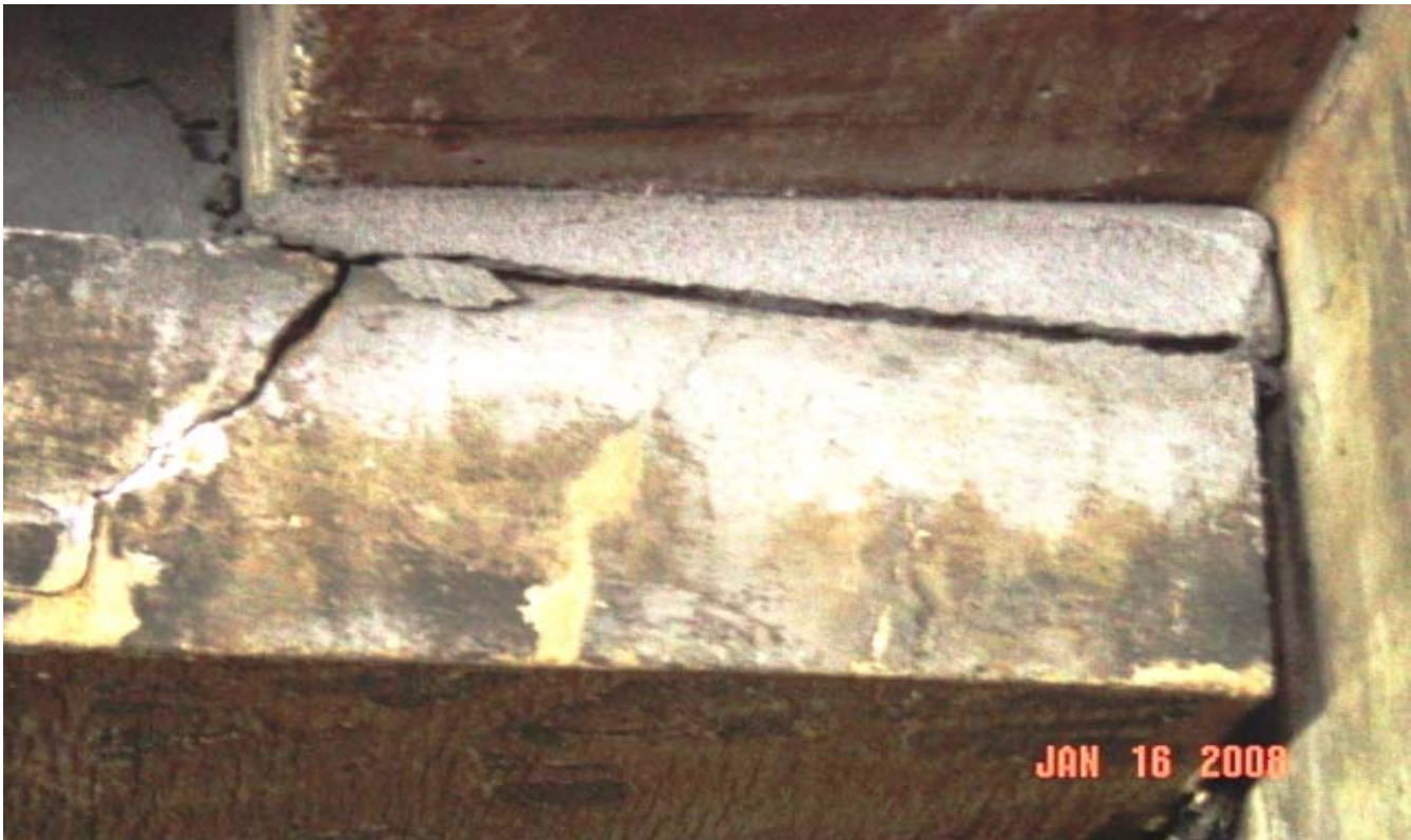
Picture 3: Cracked Concrete Support
