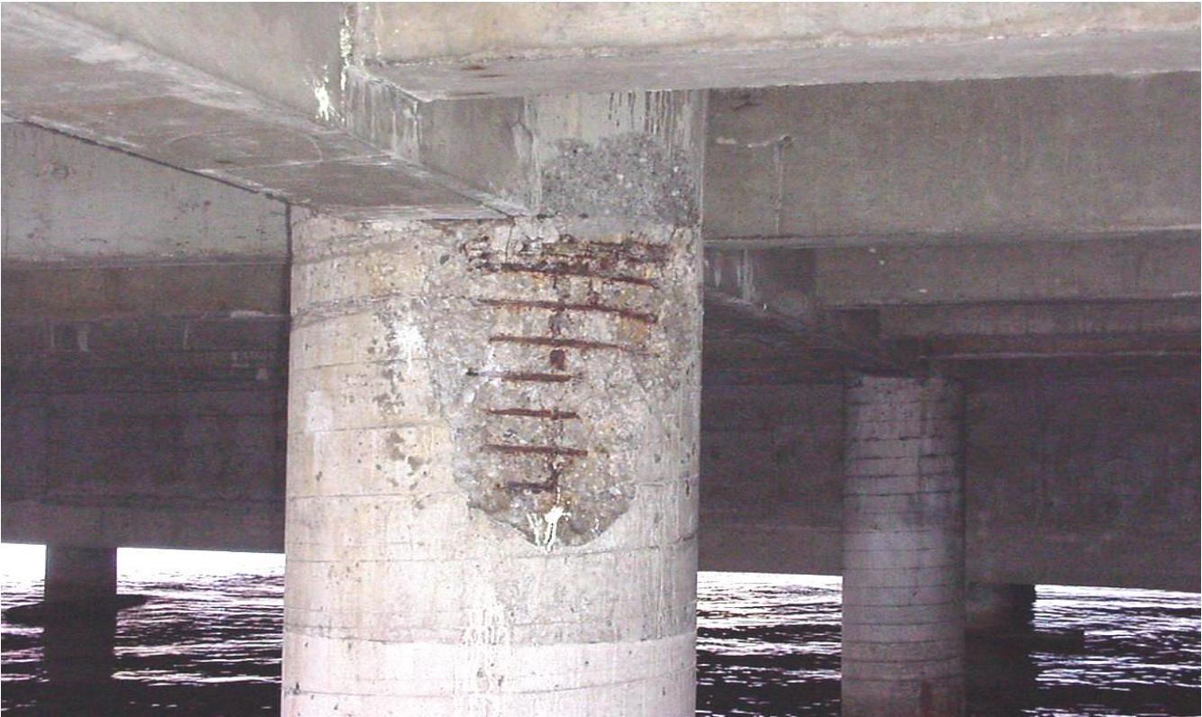
Picture # 1: Degraded Concrete Pier with Exposed, Corroded Reinforcing Steel
