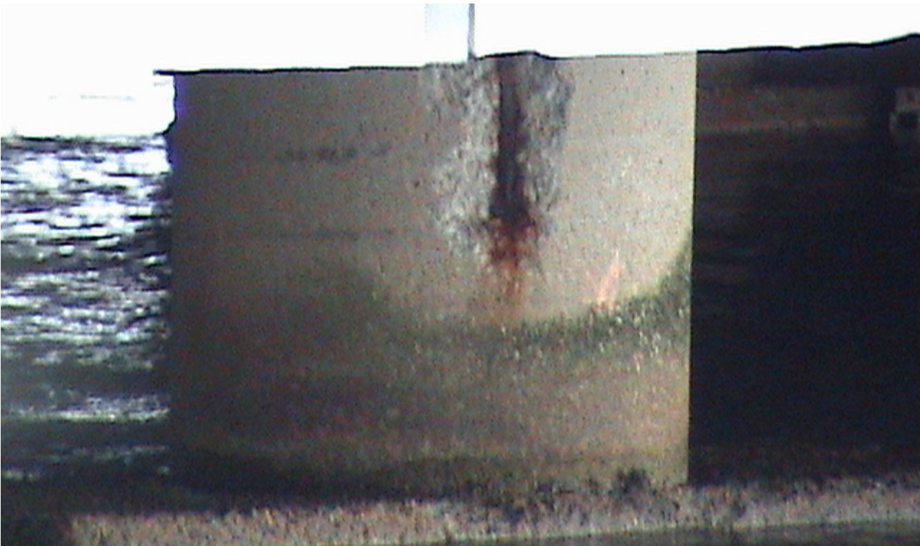
Picture # 2: Degraded Concrete Pier with Exposed, Corroded Reinforcing Steel
