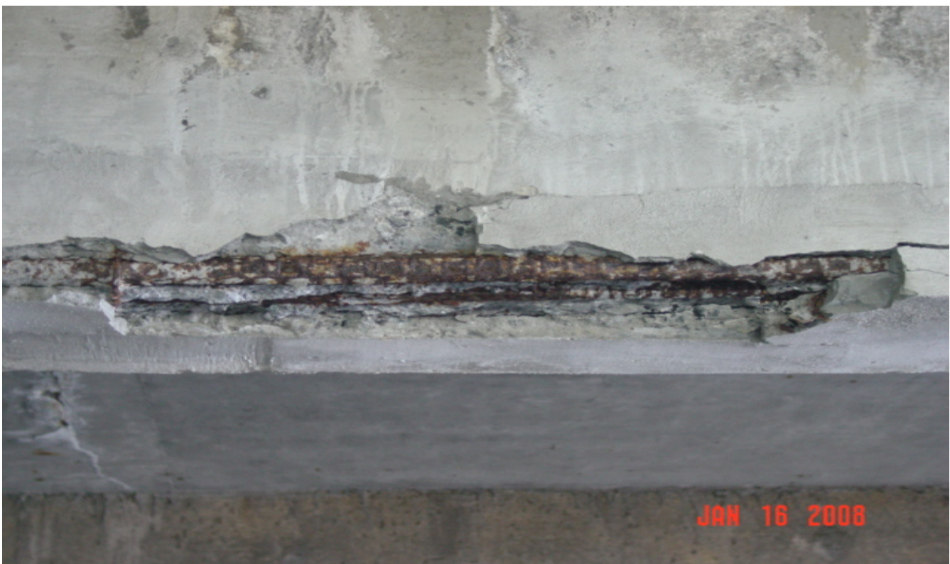
Picture # 4: Chipped and Cracked Concrete, with Exposed, Corroded Reinforcing Steel
