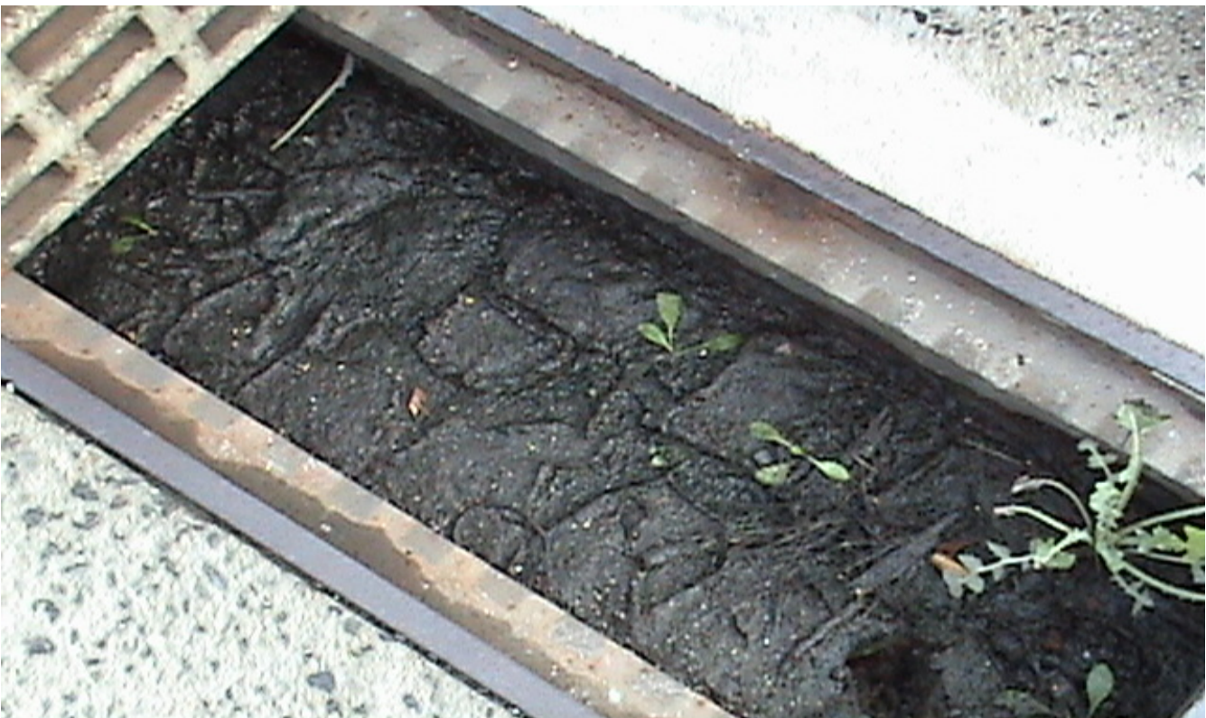
Picture # 6: Two Inches of Sludge Buildup in Drain
