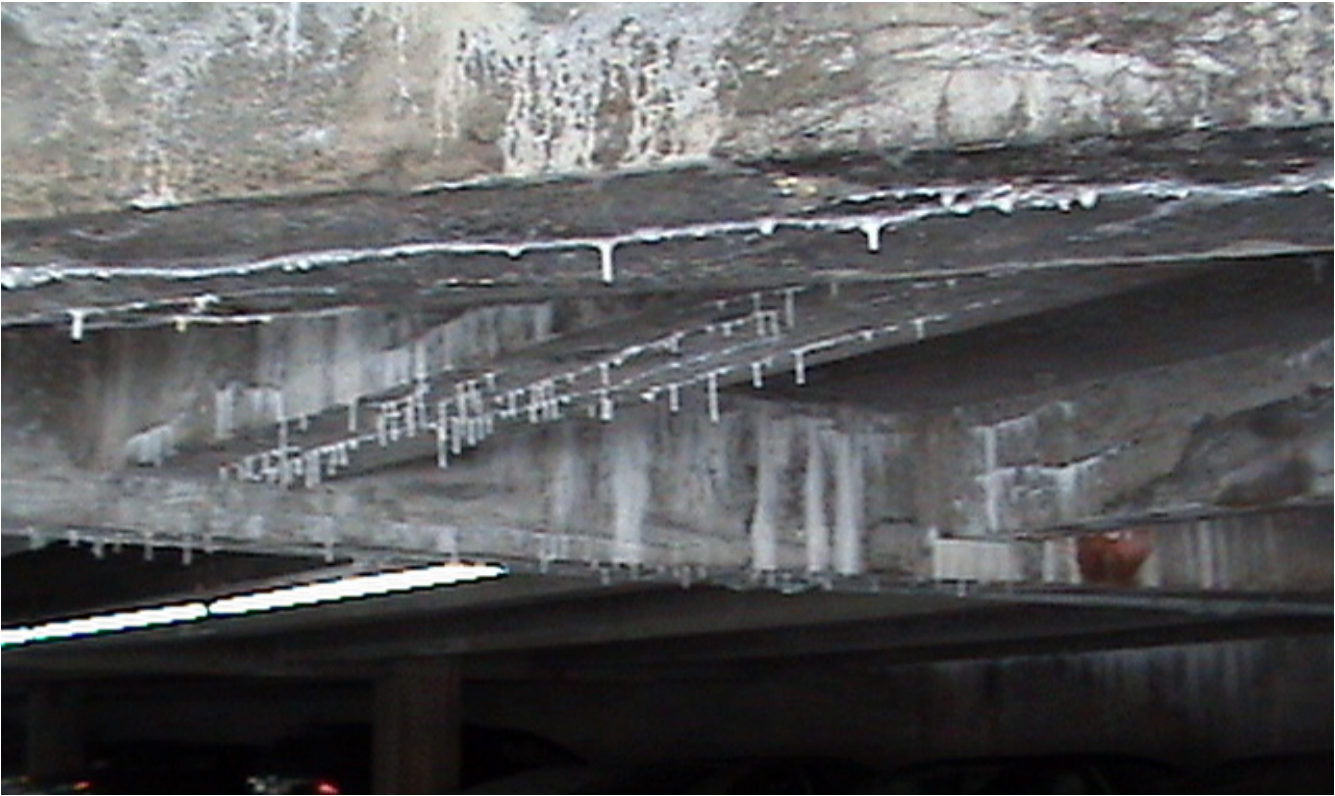
Picture # 5: Chipping and Spalling of the Concrete Surface
