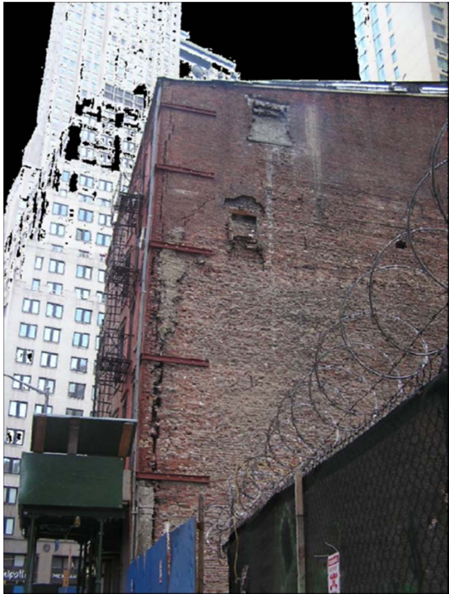
Crack at Corner
