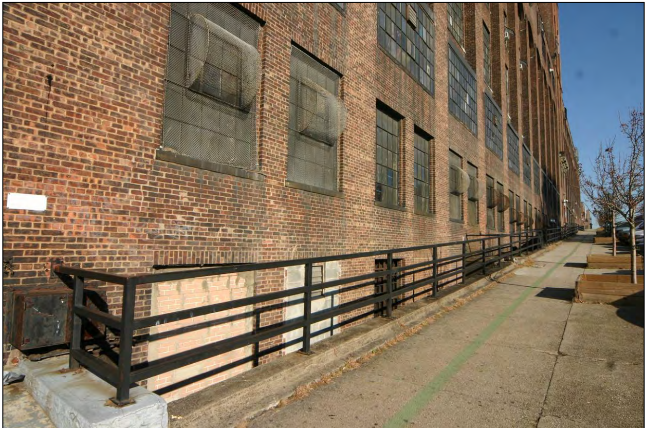
American Bank Note Company Printing Plant (Figure 9): Lafayette Avenue wing, south facade (Photo: Carl Forster)
