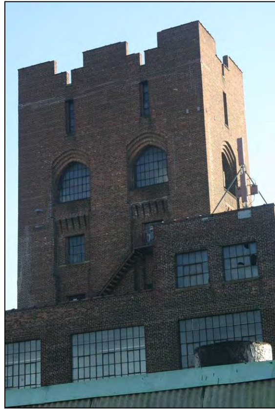
American Bank Note Company Printing Plant (Figure 8): Lafayette Avenue wing, tower, north facade (Photo: Carl Forster)
