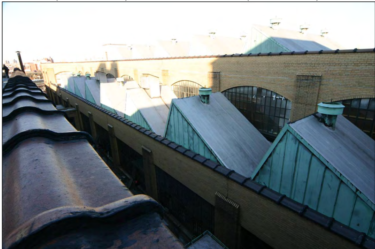
American Bank Note Company Printing Plant (Figure 25): Barretto Street wing, west facade, and coping of Lafayette Avenue wing (Photo: Carl Forster)
