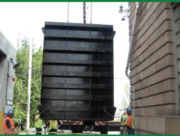
“Reservoir Operations personnel installed three stop shutters and closed three sluice gates on the Downtake 1 side. On the Downtake 2 side, an enormous stop shutter was installed using a crane.” – BWSO EHS Staff
