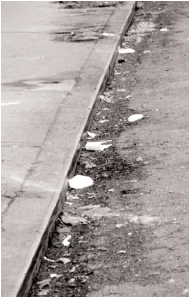
Failure to Sweep 18 Inches into the Street See "Sidewalks and Gutters"
