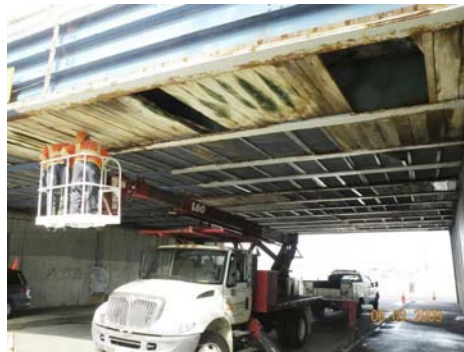
2009 Inspection: The Entire Underside of the Bay Ridge Avenue Bridge Deck is Shielded With Timber Planking and Steel Wire Mesh Netting. The Shielding was Temporary Removed to Perform the Inspection of the Deck. Shielding was Replaced After the Inspection. (Credit: NYSDOT)
