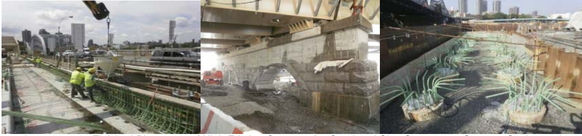
August 2010: Finished Placement of High Friction Concrete for Overhead Sign Structure at Span 9. Setting and Grouting Granite Stone Facing at Pier 8. Finished Placement of Caisson Concrete to New Higher Elevation at Bronx Relieving Platform "B".
