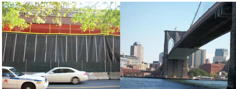
The Abrasive Blasting Operation at Franklin Square Began on August 26, 2010. Pearl Street Abrasive Blasting. Installing the Platform Under the Main Span.
