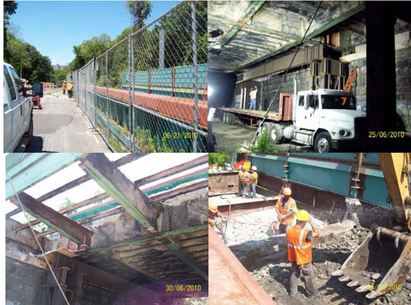
Shore Road Circle Bridge: Preparation of MPT and Work Zone, Installation of Temporary Shoring Towers, and Partial Steel Removal in June 2010.
