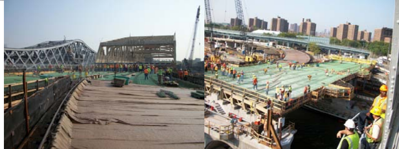
August 2010: Removal of Lead Based Paint From Structural Steel Cutline Locations Within a Class 3P Containment at the Manhattan End Span. Concrete Placement for Decks at Spans A10, A11, and 3.
