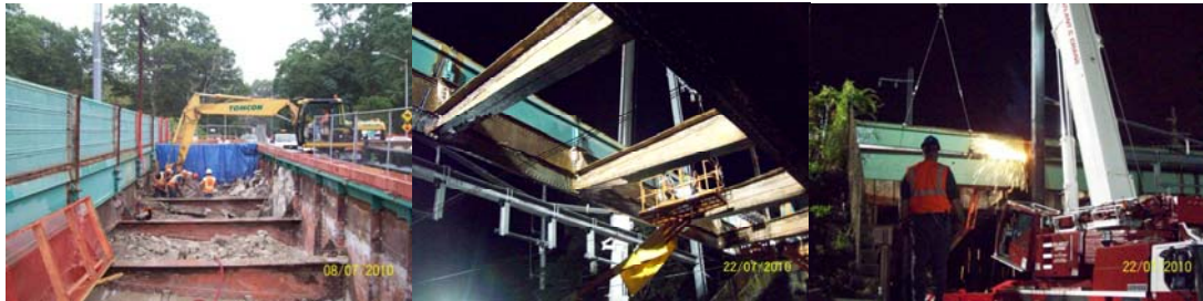
Shore Road Circle Bridge: Clearing Structural Steel for Demolition and Disassembling Steel Members in July 2010.
