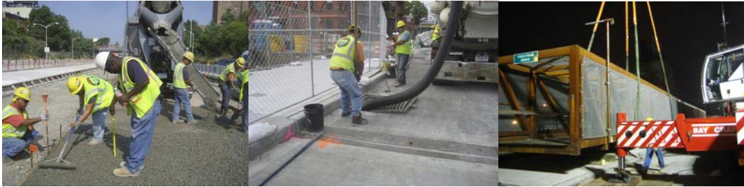
August 2010: Placing Concrete on the Northbound Left Lane. Cleaning the Drainage Structures in the Northbound and Southbound Approaches. Removed the Temporary Pedestrian Bridge, Allowing Pedestrians to Access the South Sidewalk of the New Bridge.
