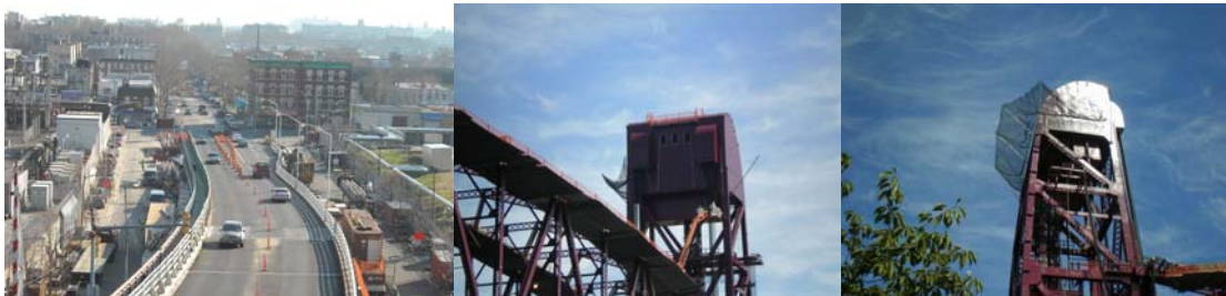
Open Queens Approach Roadway of the Roosevelt Island Bridge in December 2008. September 2009: Preparation for Tower Roof Dismantling. Nets, Tarps and Fences were Installed to Catch any Debris.
