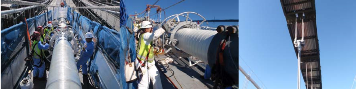
October and November 2010: New Cable Guard Installed on Cable C. November 2010: New Suspender Installed on Main Cable C.
