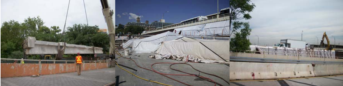
July 2010: Removing Concrete Support Beams From Ramp A. Preparing for Power Hand-Tool Operation at Ramp D. Class 3P Containment at Ramp D.
