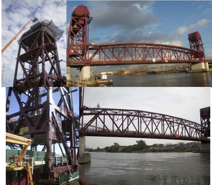
January 2010: Delivering Machinery Components to the East and West Machinery Rooms. February 2010: Removing Railing From the Roosevelt Island Side of the Bridge. July 2010: Cleaning and Dismantling of the Platform Under the Main Span.
