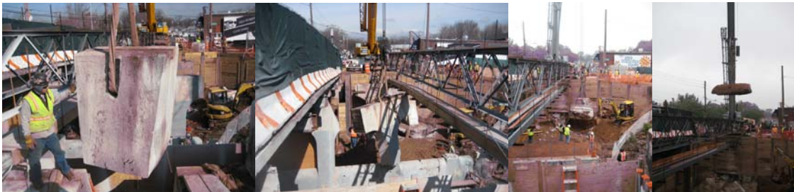
Annadale Road Bridge: Removing the South Abutment and Center Pier in March 2009. : Removing the North Abutment Footing and the Partly Embedded Abandoned Sewer Pipe Containing Asbestos in May 2009.
