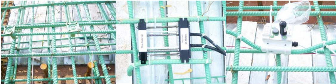
Three Types of Sensors Installed During Phase I: Vetek, CPMP, and EC11 (Embedded Corrosion Instrument).
