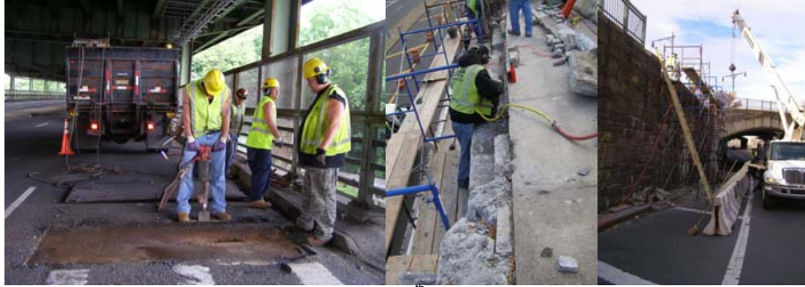
Replacing Asphalt Around a Plate on the 5 th Avenue Bridge in June 2010: Highway Repairer Robert Tuite, Bridge Repairer and Riveter Ignazio Trapani, and Assistant City Highway Repairers Umberto Fava and Thomas McKenzie II. (Credit: Joseph Flood) Cement Masons Repairing the Retaining Wall at the Southern Boulevard Bridge over East Fordham Road in November 2010. (Credit: Sohrab Hossain)
