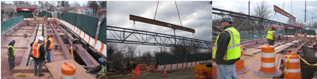
Annadale Road Bridge: Stage I Construction in February 2009. Saw Cutting the Diaphragms, Removing the Stringers, And Placing a Temporary Truss to Support Utility Conduits.
