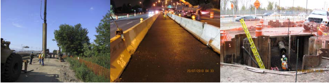
Fresh Creek Bridge in July 2010: Installing Sheathing Along the Southwest Area of the Shoreline. The Nighttime Installation of Temporary Asphalt Pavement in the Median of the Belt Parkway. November 2010: The Installation of the New Ductile Iron Sludge Force Main Being Installed Through a Jacking Sleeve that Crosses Under the Existing Roadway. (Sludge Force Main Credit: Eric Callender)
