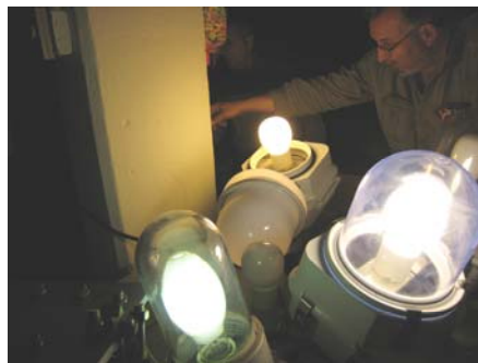
Supervisor Electrician Ben Cipriano in October 2008 With Both Mild and Bright Induction Light Fixtures for Testing. For Comparison Purposes, There is a Mix of Clear and Frosted Globes. (Credit: Russell Holcomb)
