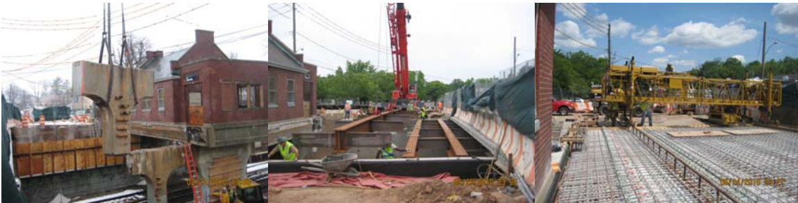
Annadale Road Bridge: Substructure Removal of Pier in Stage II in February 2010. Structural Steel Removal of Stringer in May 2010. Finishing Machine Used in Dry Run in June 2010.
