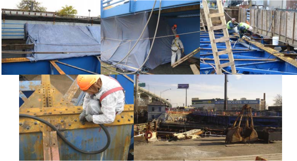
October and November 2009: Paint Removal with Vacuum Shrouded Power Hand Tool Under a Class 3P Containment. Ironworkers Removing Rivets and Dismantling Steel. December 2009. (Credit: NYSDOT)
