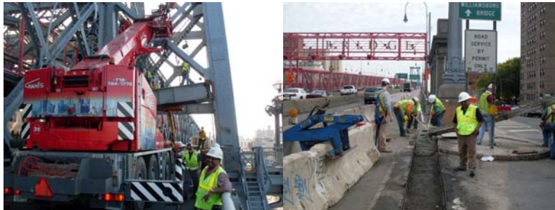
July 2010: Looking East at Damaged Brooklyn Tower (South Outer Roadway) Strut Replacement. October 2010: Looking East at the Lane 8 Precast Barrier Concrete Foundation Placement at Manhattan Plaza.
