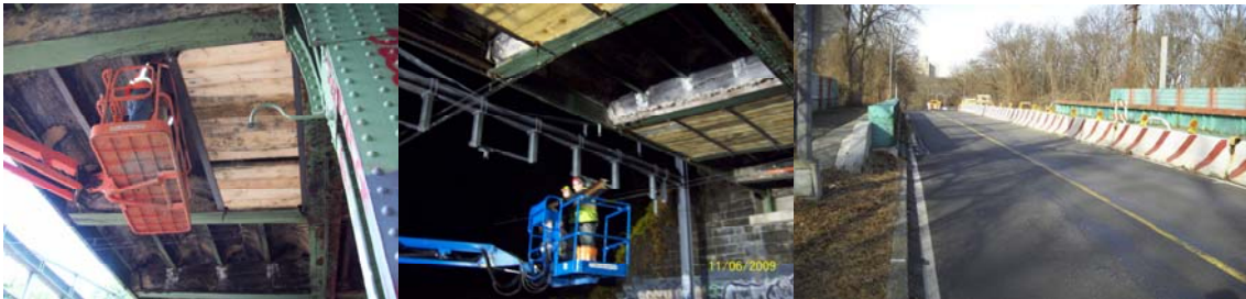
Shore Road Circle Bridge: Installing a Reinforcing Timber Beam Underneath the Existing Floor-Beam in Preparation for Stage 1A Construction in June 2009. Installing the Demolition Shielding Over Track #1 for Stage 1A in November 2009. Left Roadway in December 2009. (December Credit: NYSDOT)
