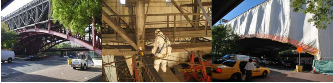
Franklin Square Arch. Inspection of Blasting Surfaces Inside the Containment in September 2010. Containment Installed at Arch in October 2010.
