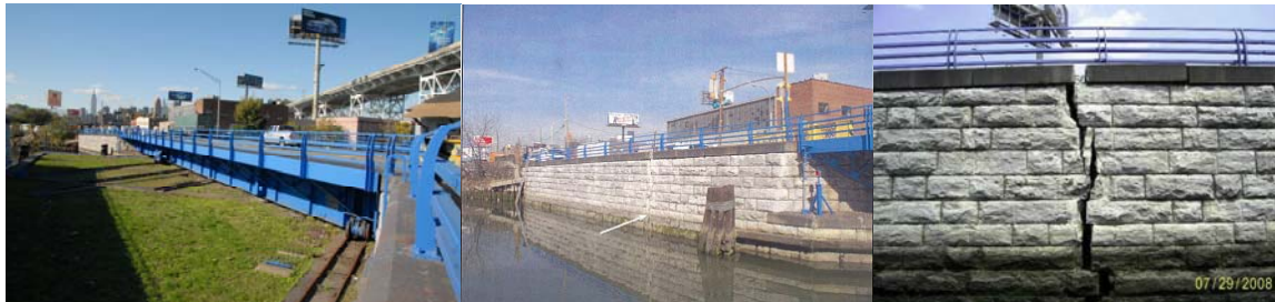
Borden Avenue Bridge. (Credit: Peter Basich) General and Close Up View of the Crack in the Wingwall. (2 nd View Credit: NYSDOT)
