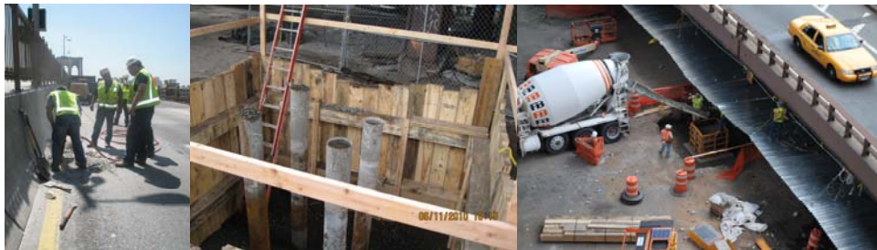
May 2010: Test Pit on Brooklyn-Bound Manhattan Approach. June and July 2010: Excavation and Concrete Placement for Pile Cap at Ramp A Bent 7A.
