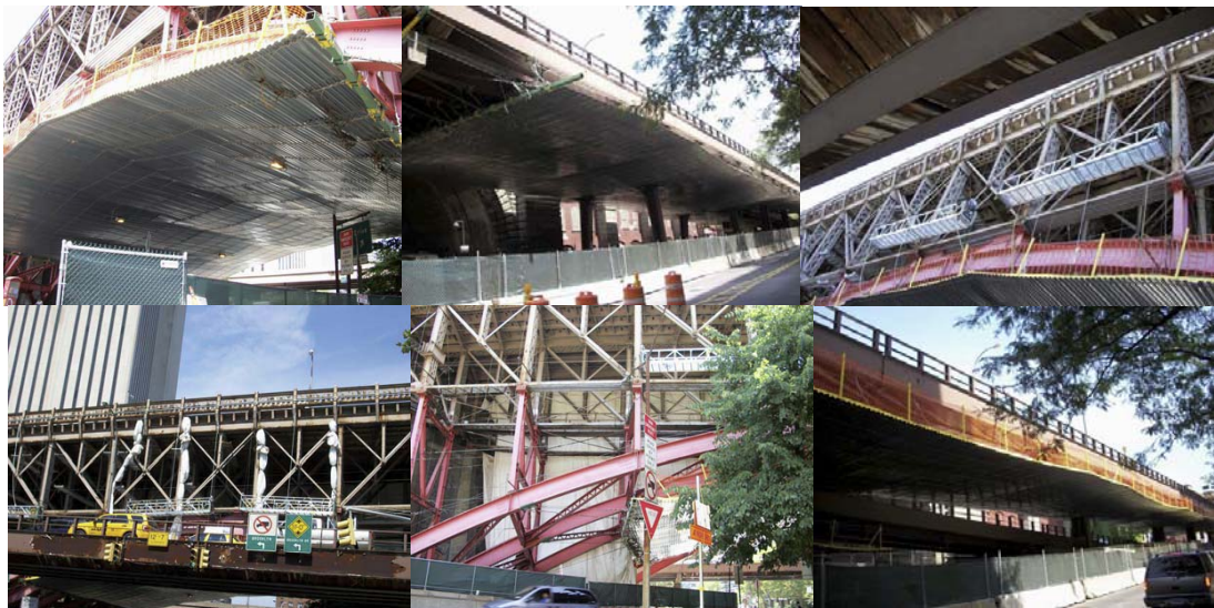
July 2010: Installation of the Platform for the Abrasive Blasting Operation at Franklin Square and the Containment Rigging at Pearl Street.
