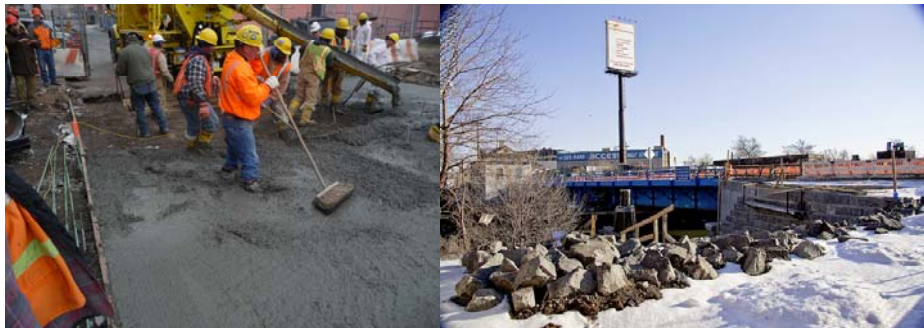
December 2010: Concrete Work. (Credit: Leonid Gitis) Late December 2010: Bridge Open to Vehicular Traffic. (Credit: Mitch Waxman)
