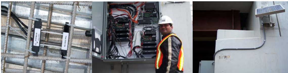
CPMP (Corrosion Penetration Monitoring Probe) Unit Installed on Clad Reinforcing Bars. Data Box and the Solar Panel.
