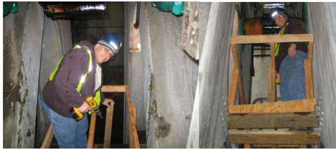
Carpenter John Green Installing a Platform for Strain Gauge Measurement at the Hamilton Avenue Bridge in March 2010. (Credit: Vera Ovetskaya)
