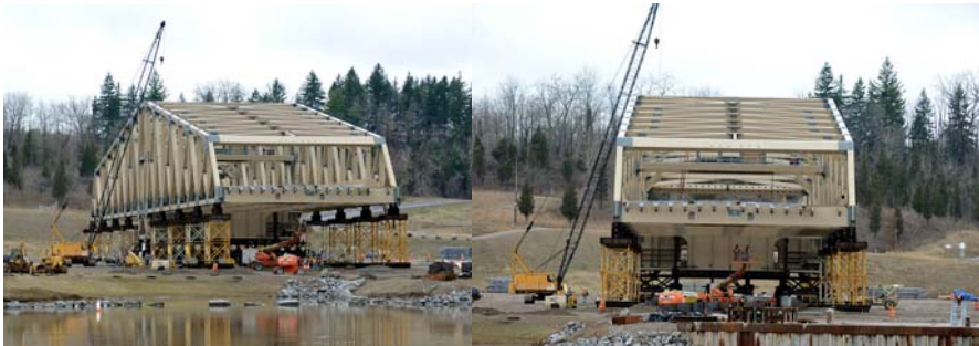
Late March 2010: Assembling the Willis Avenue Bridge Swing Span near Albany, New York. (Credit: Bernard Ente)
