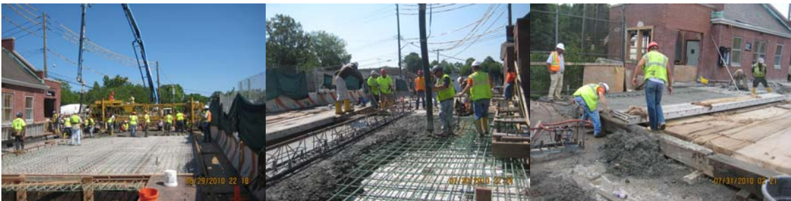
Annadale Road Bridge Stage II: Concrete Placement of the Deck Slab in June 2010 and of the Approach Slabs in July 2010.
