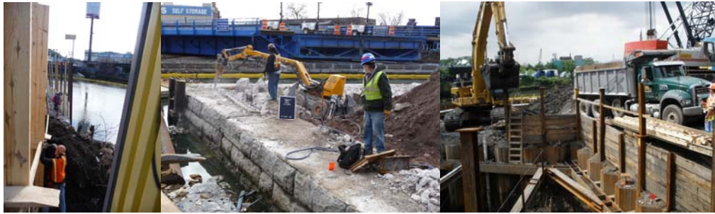
Borden Avenue Bridge in March 2009. (Credit: Tamara Berlyavsky) Demolition and Disposal of West Abutment Wall. (Credit: Reza Lotfi)
