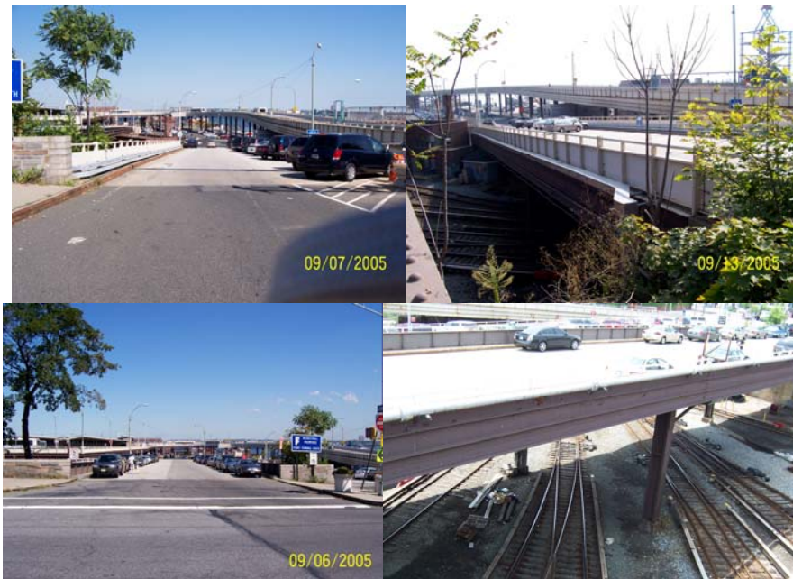
Ramp C - Commuter Entrance over SIRT Tracks. Ramp D - Commuter Exit over SIRT Tracks & Employee Parking Lot.
