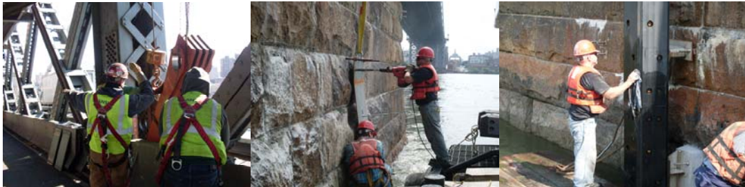
2009: Looking Southeast at the Installation of the Triangular Jacking Frame for the Intermediate Tower Bearing Replacement in January 2009. Main Tower Pier Fender System Installation in July 2009.
