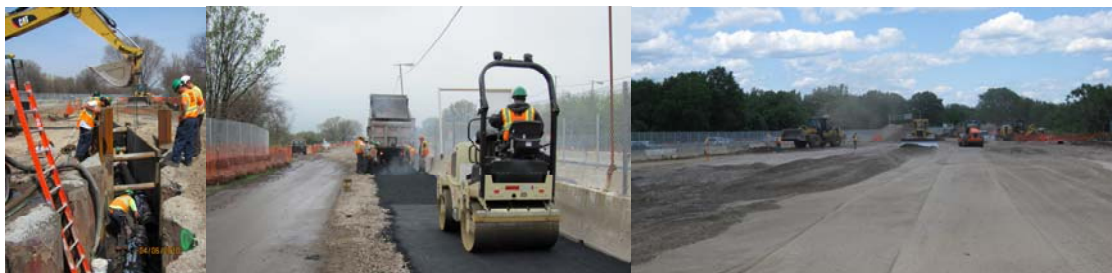
Paerdegat Basin Bridge in April 2010: The New Ductile Iron Sludge Force Main Being Installed in a Trench. The Placement and Rolling of Temporary Asphalt for the Temporary Pedestrian/Bicycle Path. June 2010: The Grading in Advance of the Placement of Embankment Material on the Eastern Approach to the New Bridge.
