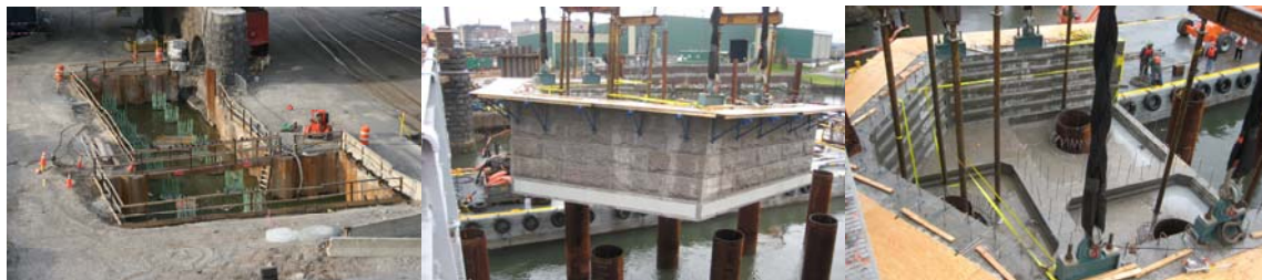
Pier 9 Drilled Shaft Footing in November 2008. The First River Pier in November 2008.
