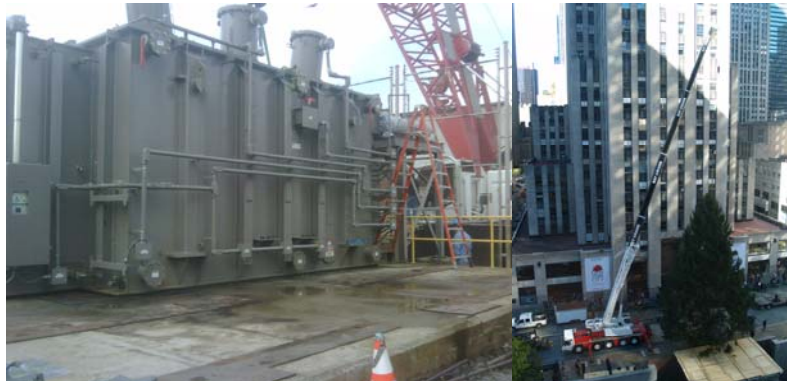
In Early June 2010, We Coordinated a Super-Sized Move for Con Edison, in Conjunction with Bay Crane Service, to Transport a 228,500 Pound Transformer, at a Gross Vehicle Weight of 428,280. In Early November 2010, a Permit Was Issued for the Double-Headed Crane That Lifted the Rockefeller Center Christmas Tree and the Trailer That Brought the Crane. (Tree Photo Credit: Bay Crane Service)
