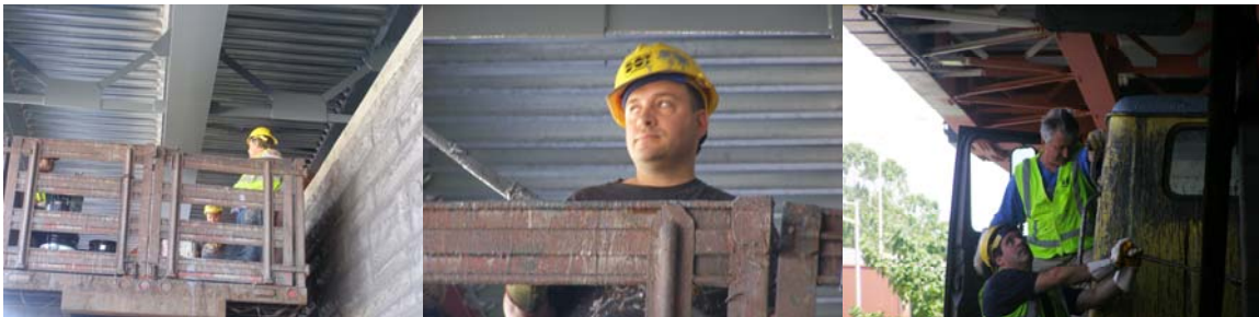
Painting the BQE Bridges in 2010: Bridge Painters Henry Bollin (Obscured), Thomas Jones (Obscured), and Michael Scotti. Bridge Painter Michael Scotti. Bridge Painters Anthony Attore and Branko Grzancic. (Credit: Earlene Powell)
