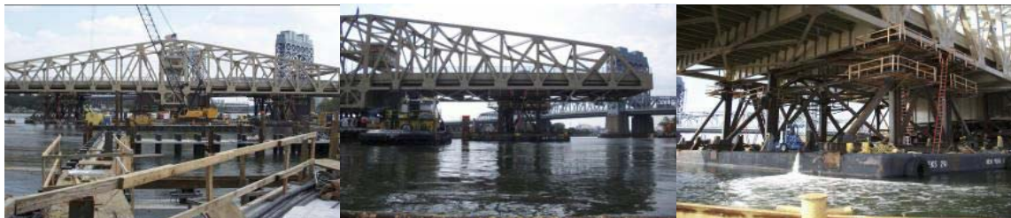
August 2010: Ballasting of Barges and Transferring the Swing Span From Twin Barge to Two Single Barges.
