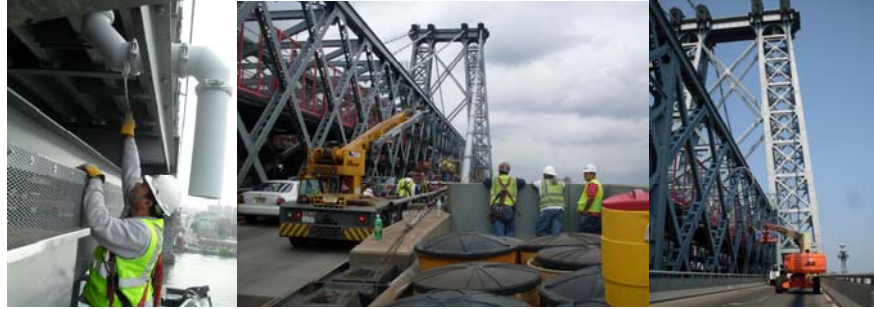
May 2010: Looking East at the Application of the Intermediate Coat on the South Outer Roadway Downspout Between PP50W and PP51W. June 2010: Looking East at the Replacement of the One Rail Bridge Rail at the Manhattan End Span. June 2010: Looking West at the Touch-Up Painting of North Truss at Brooklyn End Span.
