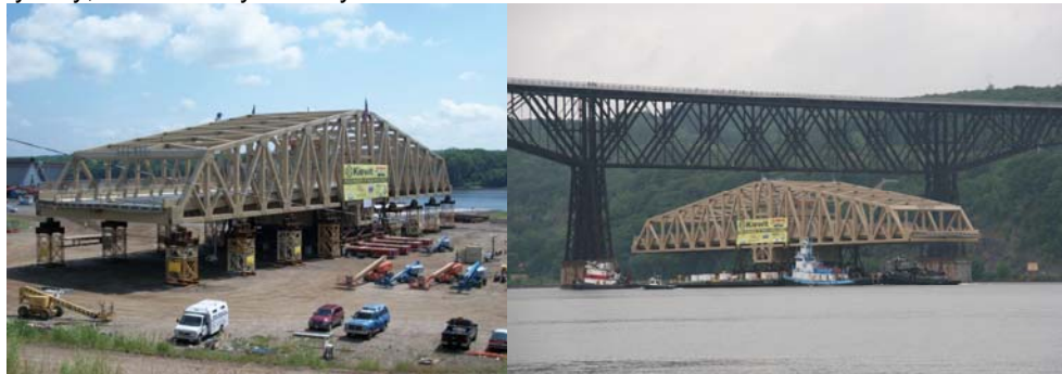
Preparing to Move the New Willis Avenue Span. Passing Under the Poughkeepsie Railroad Bridge, now a Pedestrian Bridge and State Park.
