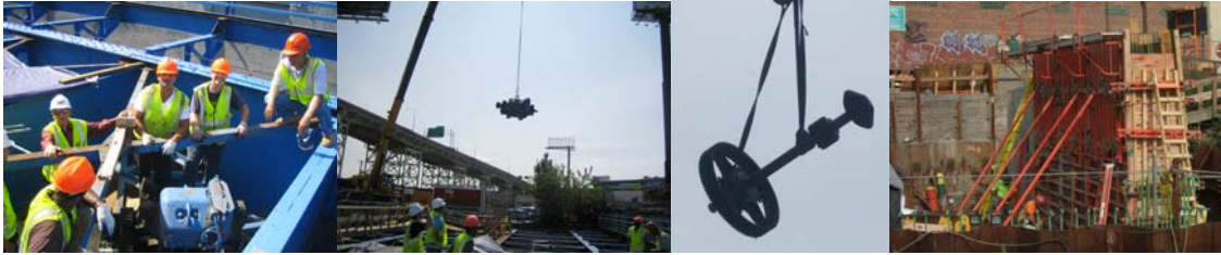
June 2010: Removing the Motor for Replacement and the Main Machinery Shaft for Rehabilitation. Oiler Carl Wharton, Mechanical Engineer Ibrahim Ibrahim, Oilers Tom Strommen and Richard Morreale, and Construction Project Manager Ali Mozaffari. (Credit: Vera Ovetskaya) September 2010: Steel repairs and concrete placement for the west abutment wall.
