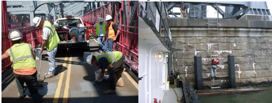
May 2009: Looking West at the Repair of the North Footwalk Overlay between PP10W and PP11W. August 2009: Looking North at Installation of the Fender System at the Manhattan Main Tower.
