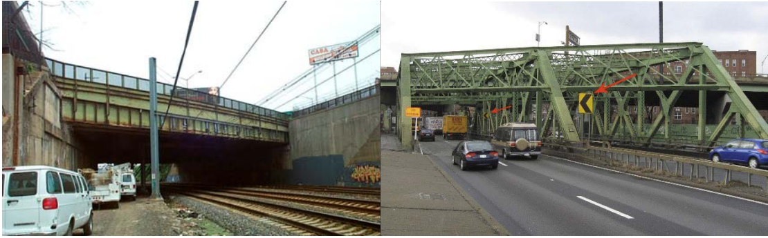
Bruckner Expressway Bridge NB in 2002. Bruckner Expressway Bridge SB in 2008. (Credit: NYSDOT)
