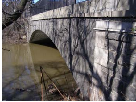
Snuff Mill Road Bridge is One of the Bridges Investigated for Scour Vulnerability and Found to be Structurally Sound, But it Remains Under Surveillance During Heavy Rains and Floods.
