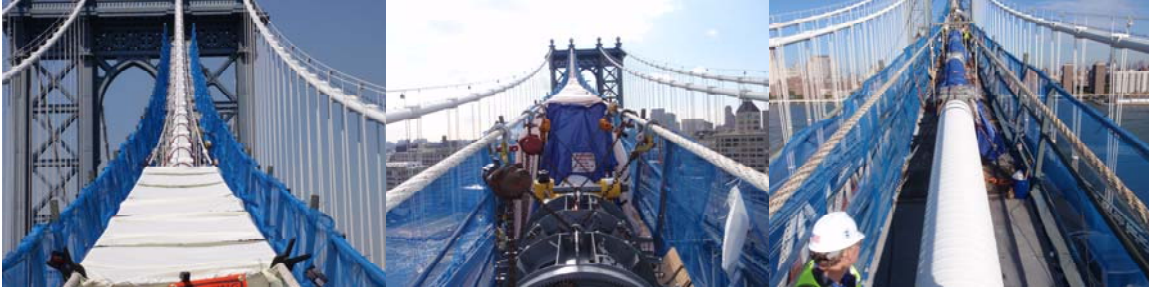
August 2010: Main Cable Work Platform With Containment Tarps. September 2010: View of Cable C With Wrapping Machine. October and November 2010: New Cable Guard Installed on Cable C.
