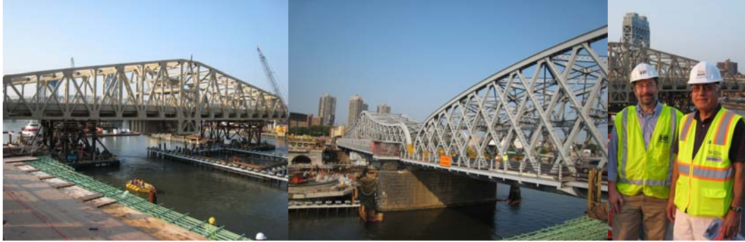
The New and Old Spans. (Credit: Russell Holcomb) Deputy Chief Engineer Russell Holcomb and Resident Engineer Abdi Hedayati.
