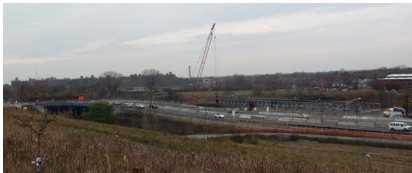
Fresh Creek Bridge in November: Overview of the Existing Bridge and the Installation of the Temporary Bridge and Approaches North of the Existing Roadway. (Credit: Eric Callender)
