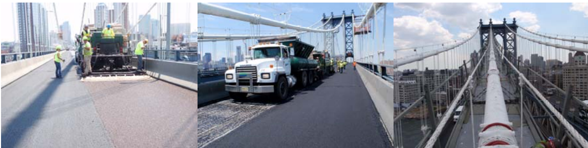
June 2010: Placement of Micro-Surfacing Layer on North Upper Roadway. July 2010: Main Cable Work Platform for Cable C.
