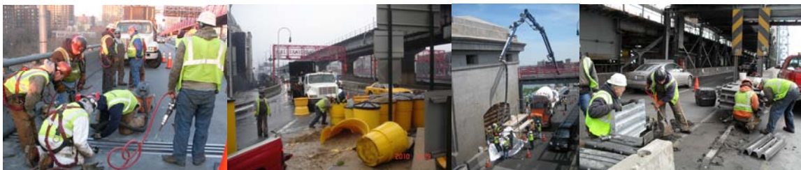
January 2010: Looking West at the Modular Joint Try-Out on the Manhattan Approach. March 2010: Looking West at the Replacement of Damaged Sand Drums at the Brooklyn Plaza. May 2010: Looking North at the Concrete Placement at the Manhattan North Comfort Station for the Wall Enclosure. March 2010: Looking East - Repairing Damaged Impact Attenuator at the Manhattan Anchorage.
