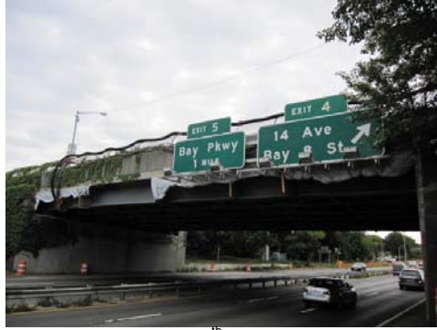
Contract Painting of Bay 8 th Street over Belt Parkway in August 2010. All Abrasive Blasting Activities Were Conducted During the Nightshift. Prior to the Abrasive Blasting Operation the Environmental Inspector Conducted Air Flow Measurements and Measured the Negative Pressure Inside of the Class 1A Containment System.
