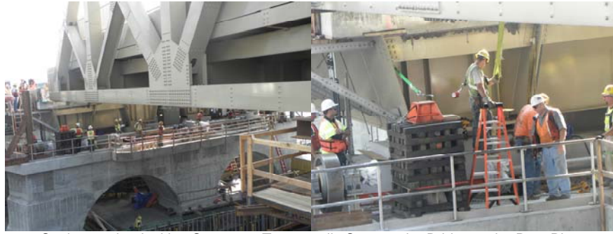
Setting up the Jacking System to Temporarily Support the Bridge at the Rest Pier. (Credit: Thomas Whitehouse)
