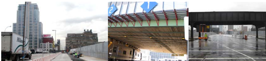
11 th Avenue Viaduct Stage 1A Construction in 2009. Installed Railroad Protective Shields. Traffic Enforcement Agent on Duty During Stage 1B Construction.
