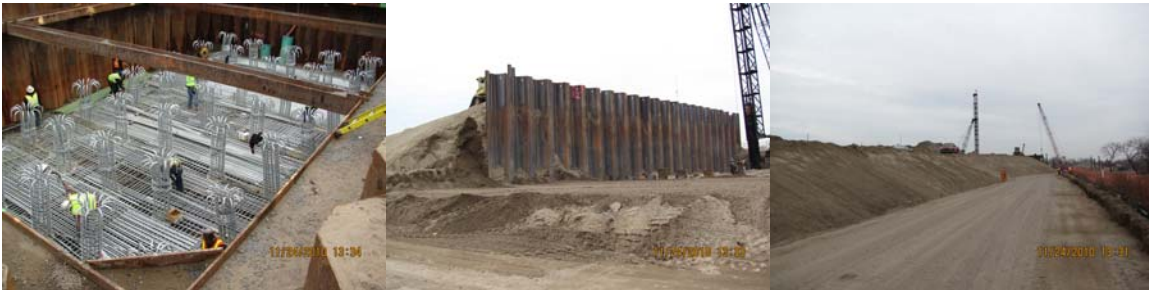
Paerdegat Basin Bridge in November 2010: The Installation of Steel Reinforcement for the New Pier Piles and Footing. The Installation of Steel Sheet Piling and Piles at the New Bridge Abutment. The New West Embankment for the Approach Roadway to the New Eastbound Bridge. (Credit: Eric Callender)
