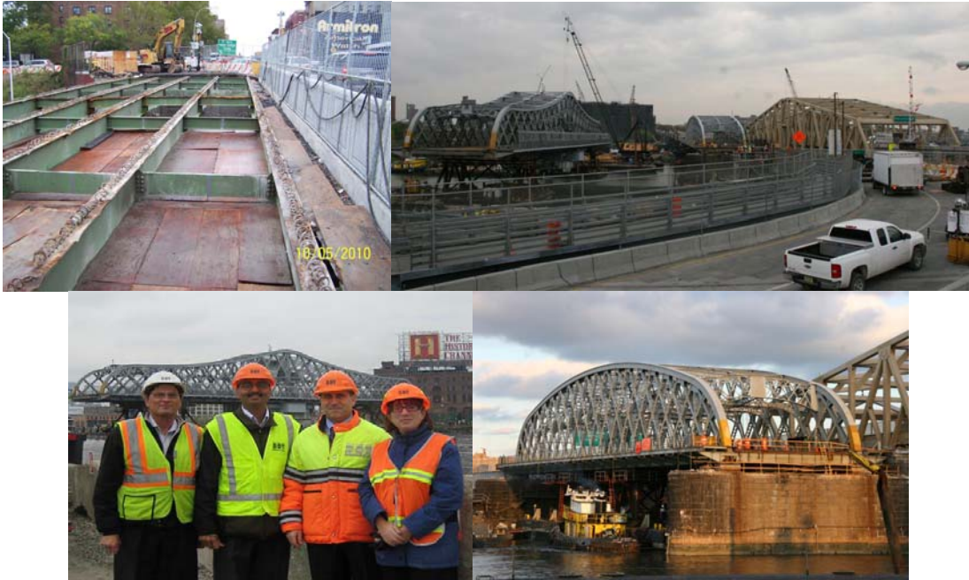
October 2010: Contractor Completed the Removal of the Concrete Deck of the Bridge over the Major Deegan Expressway. October and November 2010: Floating Out the Bridge Spans. At the Float-Out: Assistant Civil Engineer Syed Naqvi, Project Manager Ghanshyam Patel, Interim Director of Movable Bridges Hani Faouri, and Civil Engineer Simona Finkelstein. The Old Arch Span.
