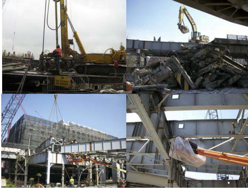
January 2010: Installing Caissons at the First Avenue On-Ramp. April 2010: Roadway and Steel Structure Demolition. Removal of Lead Based Paint From Structural Steel Cutline Locations Within a Class 3P Containment.
