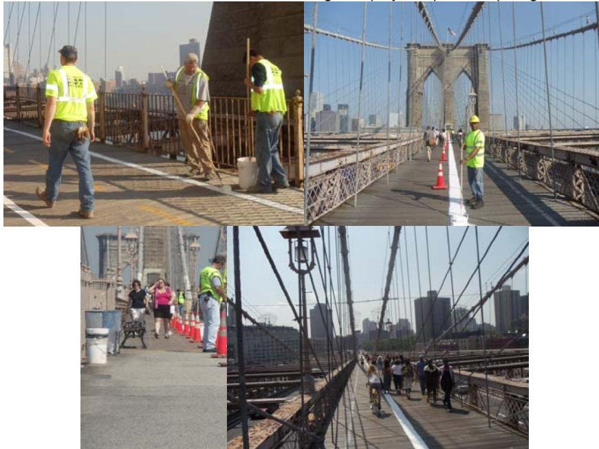
Painting the White Line on the Brooklyn Bridge Walkway/Bikeway in June 2010. Bridge Painters Frank Duic, Russell Newme, and Vlatko Zic. Bridge Painter Frank Pinheiro Painting his Last White Line Before Retiring. Supervisor Bridge Painter Cesar Pazmino Checking the Line. The Freshly Painted Line. (Credit: Earlene Powell)
