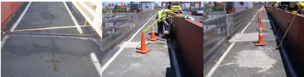
April 2010: Repairing Spalled Asphalt (a Tripping Condition) Near a Finger Joint on the Pulaski Bridge. (Credit: Samuel Teaw)
