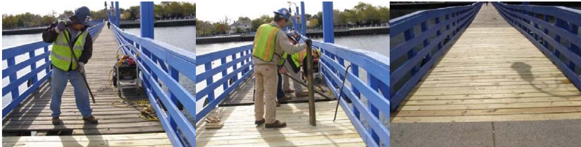
Replacing Planks on the Ocean Avenue Bridge: Carpenters John Green, Mark Pavia, Michael Short, and Andrew Myjer. (Credit: Pinakin Patel)
