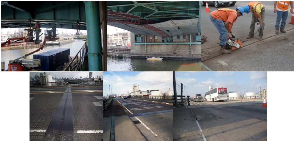
Installing Temporary Shielding Under the Main Span and Deck Joint Repair Work in June 2010. Before Construction. Stage I Complete in October 2010.
