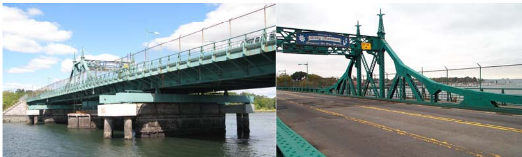
City Island Road Bridge in 2010. (Credit: Bojidar Yanev) Vertical Clearance Posting. (Credit: NYSDOT)
