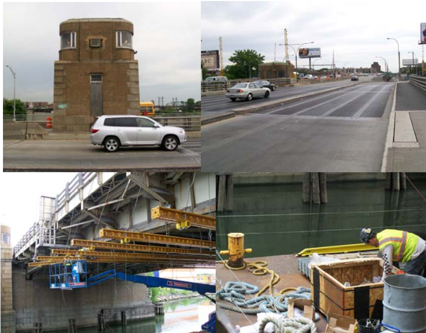
Contract Painting of Bruckner Expressway (Eastbound) Bridge over Bronx River in June 2010.
