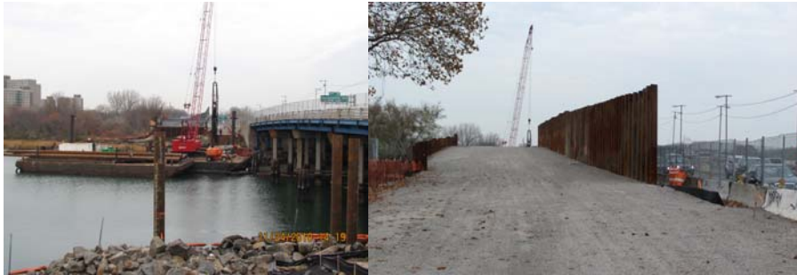
Fresh Creek Bridge in November 2010: The Installation of the Temporary Taper Tube Steel Piles via a Barge-Mounted Crane. The Piles are Designed and Installed to Support the Temporary Bridge. The Temporary Approach Roadway to the Temporary Bridge. (Credit: Eric Callender)
