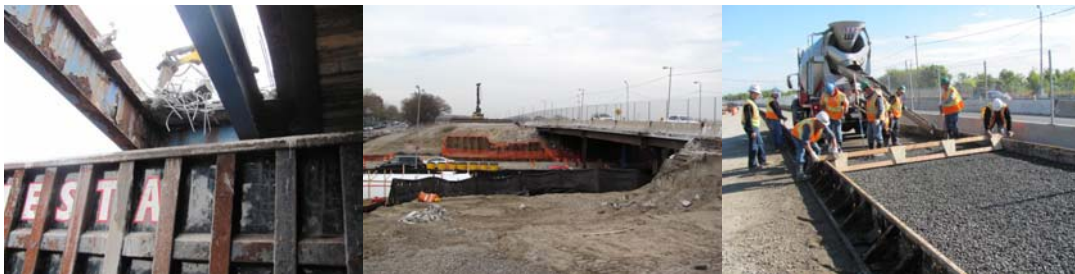
Rockaway Parkway Bridge in November 2010: Stage II Demolition of the Existing Bridge Concrete Deck. Overview of the Stage II Demolition. The Asbestos Abatement Operation is in the Foreground. The Installation of New PCC Roadway for the Westbound Off Ramp.
