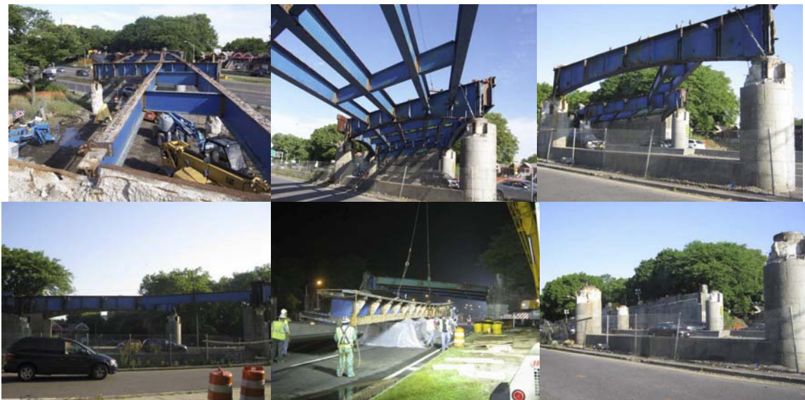
East 8 th Street Bridge Superstructure Steel Removal in June 2010. Loading a Fascia Girder on a Trailer. North View After Completion of Steel Removal.
