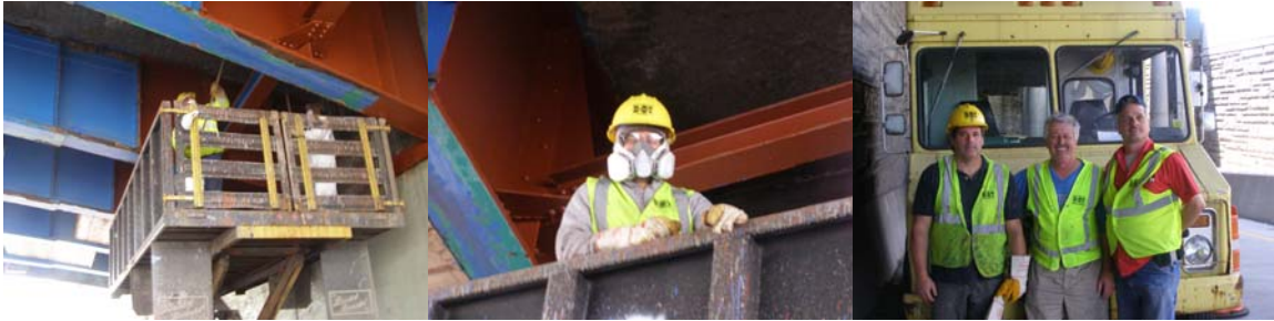
Painting a Belt Parkway Overpass in April 2010: Bridge Painters Osvaldo Lima and Julio Perez. Painting the BQE Bridges in 2010: Bridge Painters Anthony Attore, Branko Grzancic, and Supervisor Bridge Painter David Yanolatos. (Credit: Earlene Powell)
