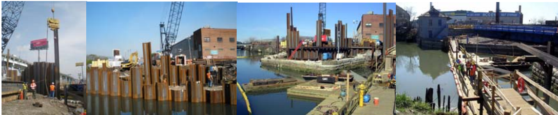
Sheet Piling of Cofferdam. Closeup of Sheet Pile Driving Operation for the West Abutment. (West Abutment Credit: Reza Lotfi) Reconstruction of West Abutment of the Borden Avenue Bridge in April 2009. (Credit: Bernard Ente)
