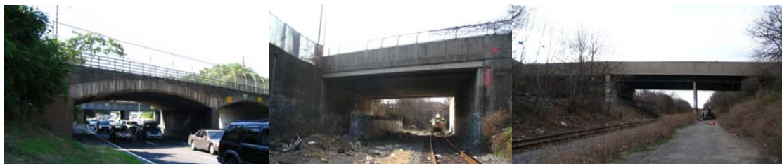
Superior Road Bridge over Cross Island Parkway, 15 th Avenue Bridge over LIRR Bay Ridge, 13 th Avenue Bridge over LIRR & Sea Beach.
