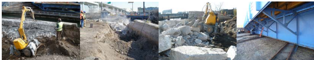
Demolition of the West Abutment and Wingwall in February 2009. (Third View Credit: Reza Lotfi) February 2009. (Credit: Tamara Berlyavsky)
