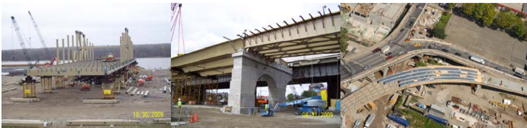
October 2009: Assembling the Willis Avenue Bridge Swing Span near Albany, New York. Willis Avenue Bridge August 2009: Installation of Tub Girders on Temporary Supports. September 2009: Existing and New Ramps to Bruckner Boulevard.
