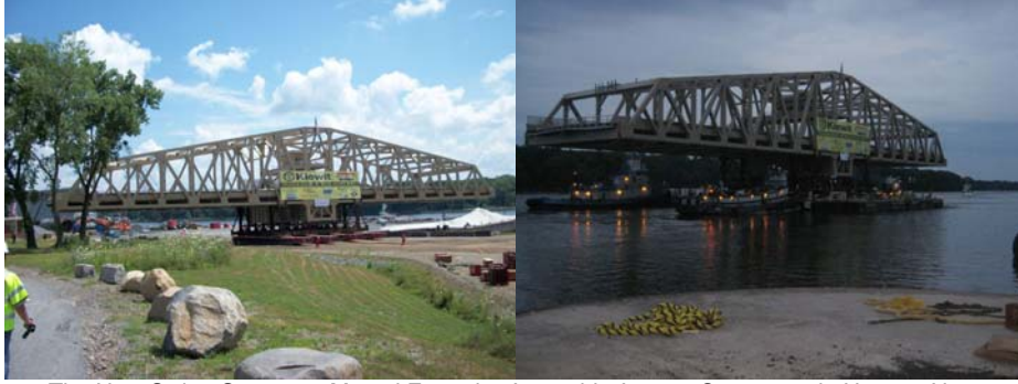
The New Swing Span was Moved From the Assembly Area at Coeymans in Upstate New York to the Twin Barges on July 11 and 12, 2010. It was Then Delivered by Barge to the Contractor Facility in Jersey City, New Jersey on July 14.
