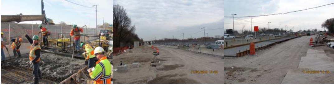
Rockaway Parkway Bridge in November 2010: The Consolidation Operation for the New PCC Roadway for the Westbound Off Ramp. The Installation of New Concrete Curbing, Catch Basin and Electrical Facilities for the New Westbound Roadway. The Installation of Formwork in Advance of the Installation of the New Westbound Roadway. (Westbound Roadway Credit: Eric Callender)
