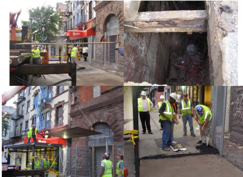
Bridge Repairer and Riveter Joseph Hickey Operating a Boom Truck Hoisting a Plate, While Executive Director of Bridge Preventive Maintenance and Repair Thomas Whitehouse (in the Background) Dumps Bags of Cold Patch. The Exposed Vault. Bridge Repairer and Riveter Chris Mauldin Atop the Bus Shelter Guiding the Placement of the Steel Plate; Executive Director of Bridge Preventive Maintenance and Repair Thomas Whitehouse and Bridge Repairer and Riveter Scott Mahaffey (Behind the Shelter); Bridge Repairer and Riveter James Wright III and Supervisor Bridge Repairer and Riveter Gean Pilipiak; and Bridge Repairer and Riveter Joseph Hickey (Obscured). EDC Representatives (Back Row); EDC's Emergency When and Where Contractor Laborer and Supervisor (Front Left); Supervisor Bridge Repairer and Riveter Gean Pilipiak (Middle); and Executive Director of Bridge Preventive Maintenance and Repair Thomas Whitehouse Leveling the Cold Patch to Set the Steel Plate. (Credit: Reza Taheri)
