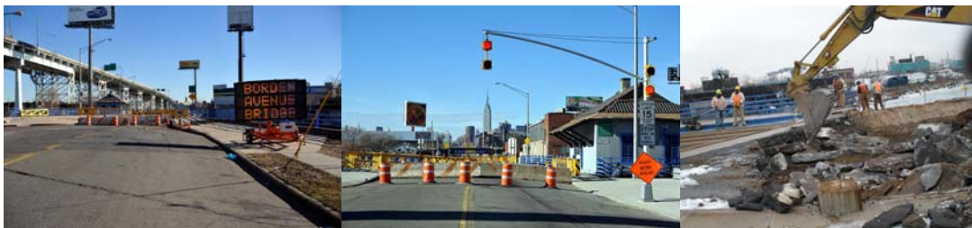
Borden Avenue Bridge Closed for Emergency Repairs in January 2009. (Credit: Bernard Ente) Roadway Excavation in January 2009.
