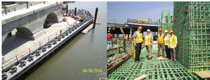
April 2010: Pier 7 Construction. At Pier 4: FHWA Area Engineer David Hart, Engineer-in-Charge James Cusack, FHWA Structural Engineer Earl Dubin, Resident Engineer Abdi Hedayati, and Interim Director of Movable Bridges Hani Faouri.
