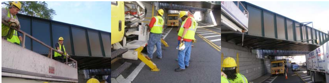
Painting the BQE Bridges in 2010: Bridge Painters Thomas Jones and Anthony Attore. Operating the Lift: Bridge Painter Brian Casey, Supervisor Bridge Painter David Yanolatos, and Bridge Painter Henry Bollin (Obscured). Completed Paint Job. (Credit: Earlene Powell)
