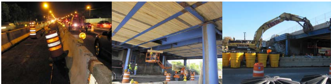
Rockaway Parkway Bridge in July 2010: The Nighttime Installation of Temporary Asphalt Pavement in the Median of the Belt Parkway. September 2010: Installing Planks Along the Lower Flanges of the Stringers. November 2010: Stage II Demolition of the Existing Bridge Superstructure.
