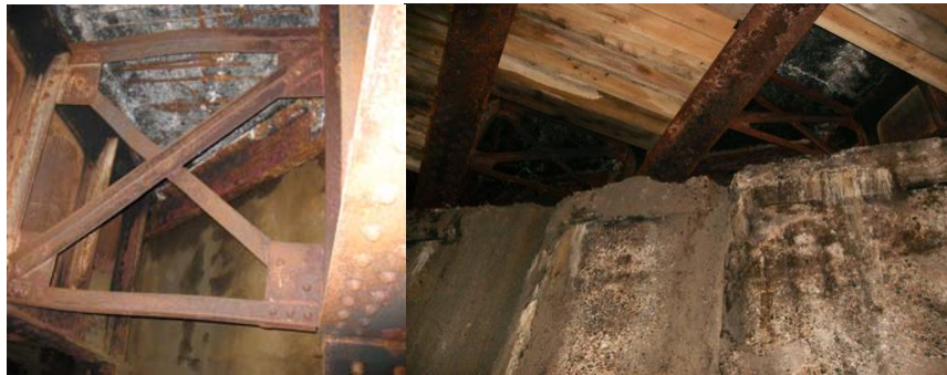
Deteriorated Bridge Deck With Exposed Rebar and Warped Steel Bracing Due to the Heat From the Fire. Timber Shielding on the Underside of the Bridge.
