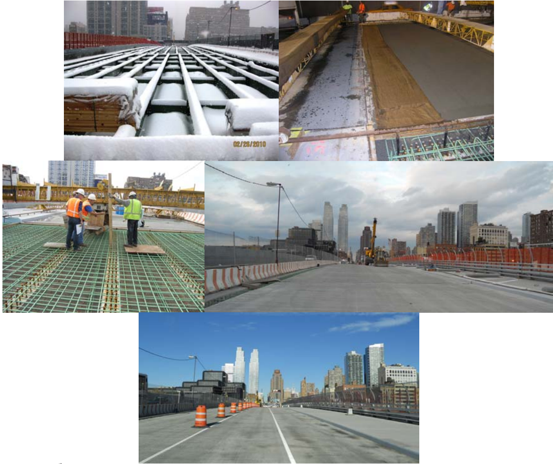
11 th Avenue Viaduct: Demolition of the Old Deck in February 2010. Inspecting Machine Setup Prior to Placing the New Deck Slab Concrete in October 2010. First Concrete Pour in August 2010. (Credit: Hui Yang) Working on Bridge Rail and Pedestrian Fencing in November 2010. (2 nd Rail Credit: Hui Yang)
