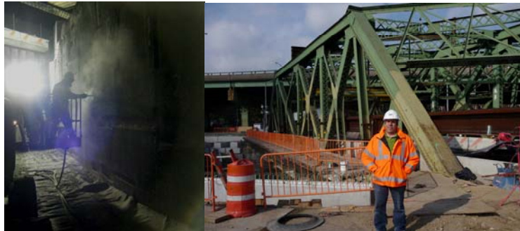
May 2010: Removing Hollow Concrete Along the Abutment Wall. (Credit: Richard Solomon) Associate Project Manager Richard Solomon at the Bridge in October 2010.
