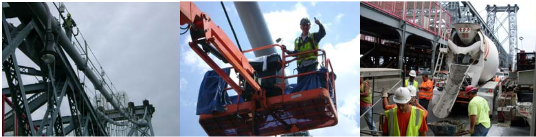
July 2010: Looking West From the North Outer Roadway at Painting on Cable A. Looking East From the North Outer Roadway at the Painting of Cable D. Looking West at the Concrete Placement at the Brooklyn North Comfort Station for the Wall Enclosure.
