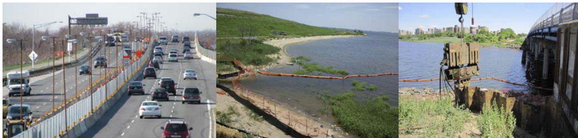
Fresh Creek Bridge in March 2010: The Temporary Lighting System Installed on the Temporary Median Barrier Leading up the Eastern Approach to the Bridge. May 2010: Turbidity Curtain Along the Shoreline. June 2010: Equipment for Driving in Sheet Metal Piling.
