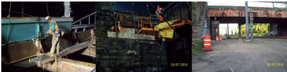
Shore Road Circle Bridge: Steel Demolition and Structural Steel After Paint Removal in July 2010.
