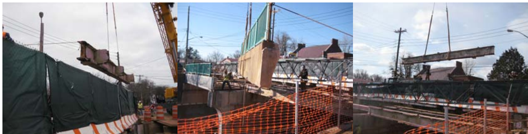
Annadale Road Bridge: Stage I Construction in February 2009. Placing a Temporary Truss to Support Utility Conduits. Removing the Eastern Bridge Railing Fence and the Stringer.
