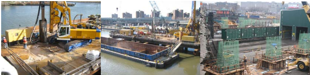
2009: The Primary Equipment Utilized During Caisson Installation was an Augering System Driven Into the River Bottom. Water From the Harlem River was Pumped Into the Augering System. All Augered Waste was Pumped out of the Caisson Into a Weir Barge. All of the Water Within the Weir Barge was Filtered Through a Fabric Medium and Pumped Back into the Harlem River. This System Effectively Removed all of the Solids From the Wastewater. April 2009: Willis Avenue Bridge Pier 9 Rebar Columns.
