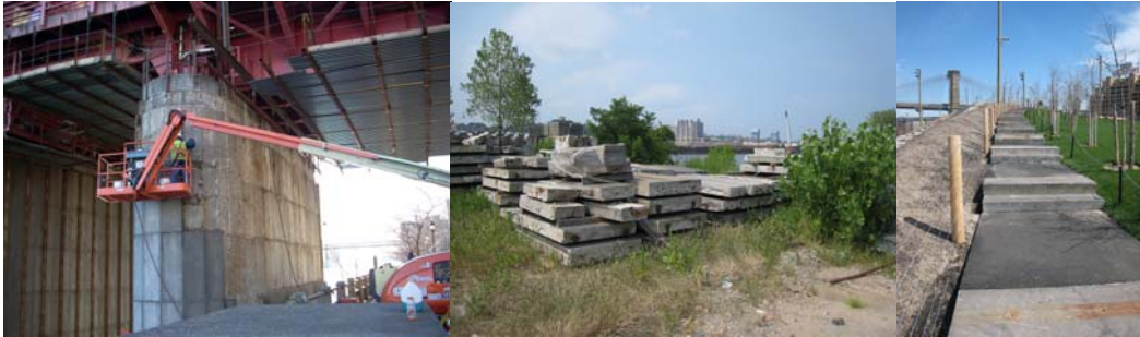
Removing the Roosevelt Island Bridge Panels. Piled Panels Awaiting Transfer to the Park.
