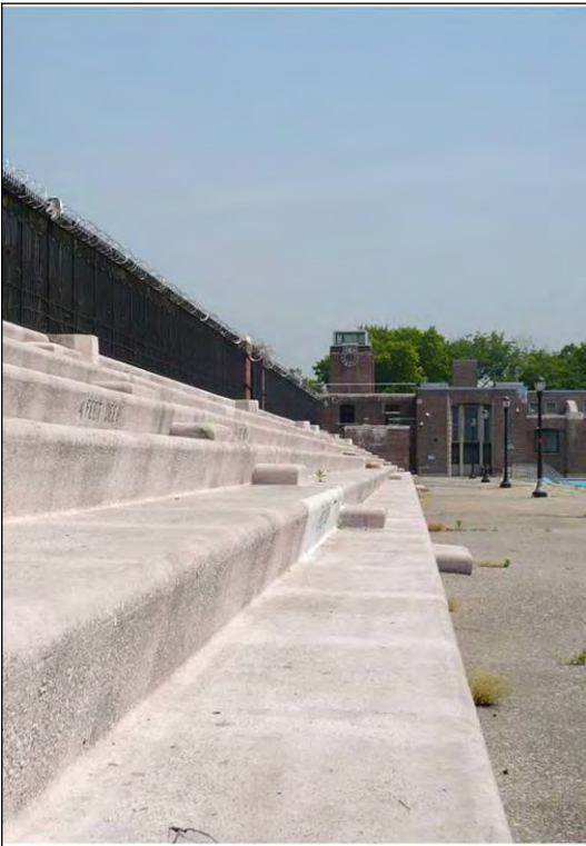
Crotona Play Center: Pool Deck Area Bleachers (view north) (l); Bleachers & Filter House South Facade (view northeast) (r), Borough of the Bronx
