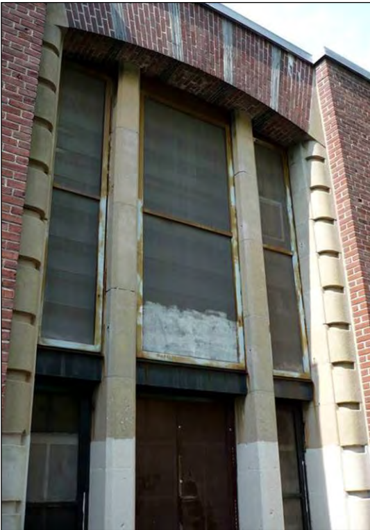
Crotona Play Center: Bath House North Facade (view south) (l); East Facade (view southwest) (r), Borough of the Bronx
