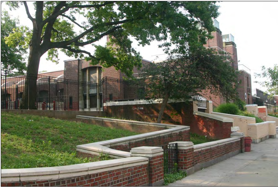
Crotona Play Center: Retaining Wall near Former Wading Pool Area (view southeast), Borough of the Bronx
