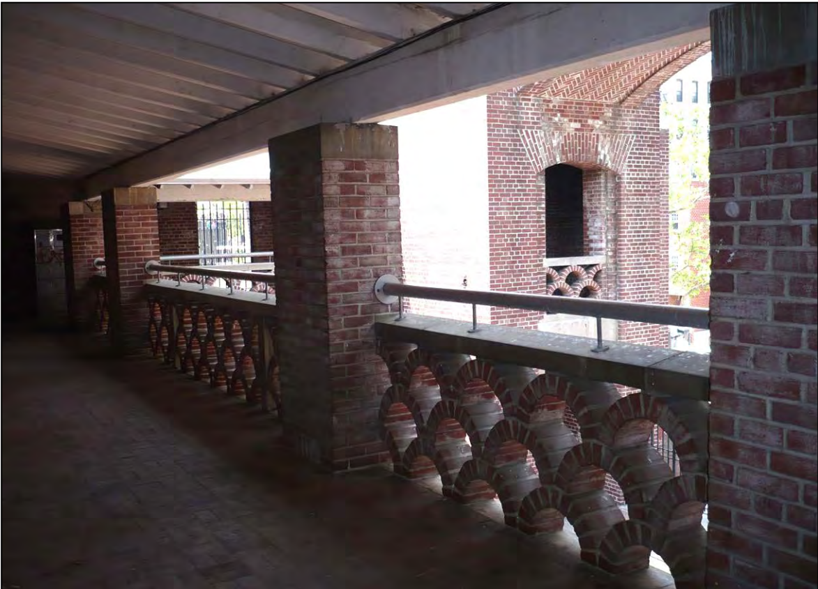
Crotona Play Center: Entrance Courtyard, Second Story Gallery (view southwest), Borough of the Bronx
