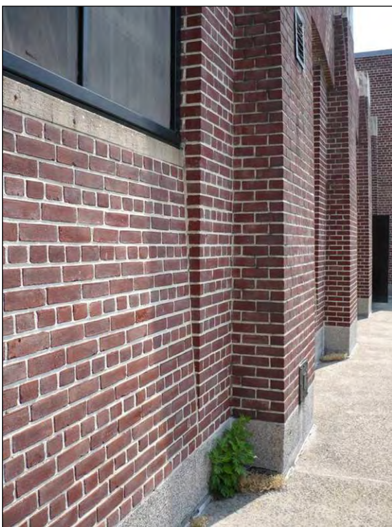
Crotona Play Center: Bath House South Facade Details, Brickwork (l); Frederick G. R. Roth Ibis Sculpture (r), Borough of the Bronx
