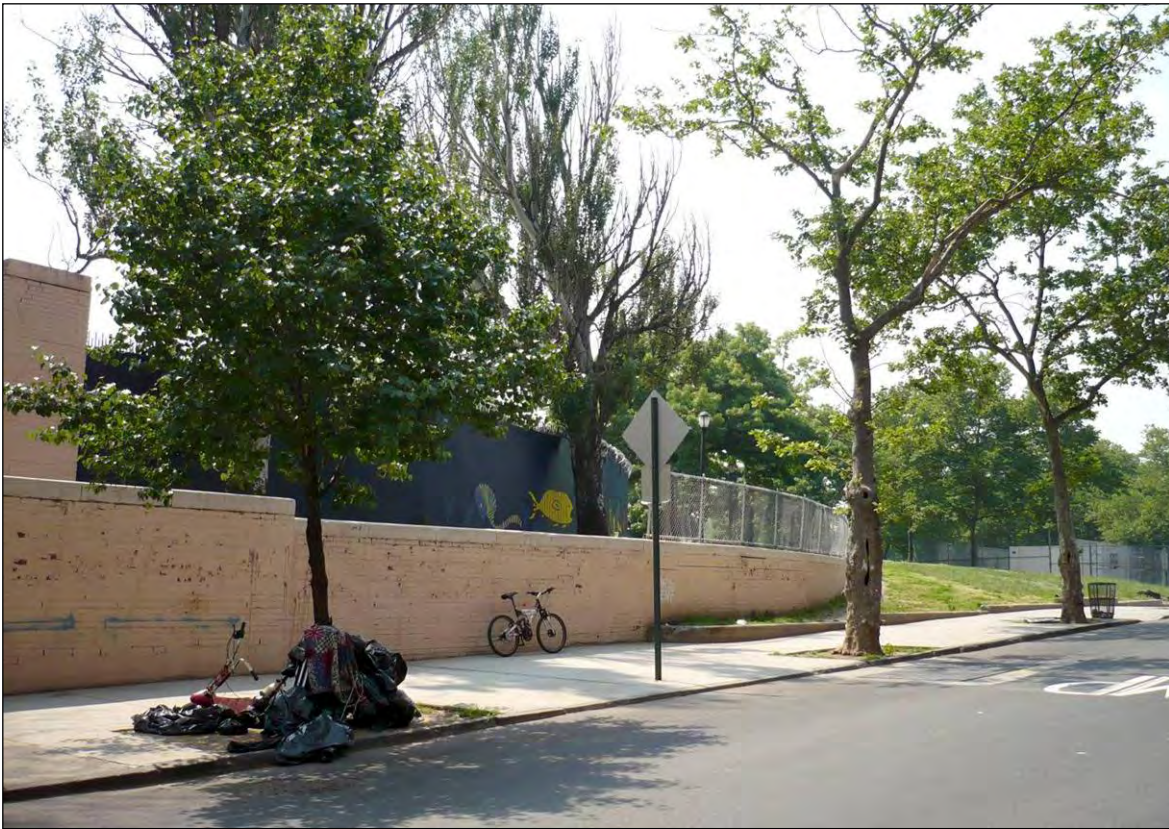
Crotona Play Center: Fulton Avenue Retaining Wall (view southeast), Borough of the Bronx
