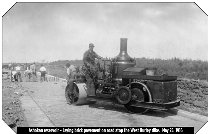
Ashokan reservoir - Laying brick pavement on road atop the West Hurley dike. May 25, 1916
