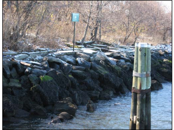
Outfall ID: PR-007 Location: SAILOR SNUG HR. (BRENTWOOD AVE) Latitude: 40° 38' 44" Longitude: 74° 6' 14" Outfall Size: 15" DIA Receiving Water: KILL VAN KULL
