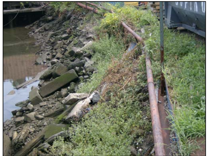
Outfall ID: PR-025 Location: SOUTH AVENUE Latitude: 40° 38' 29" Longitude: 74° 9' 57" Outfall Size: 10" DIA Receiving Water: NEWARK BAY
