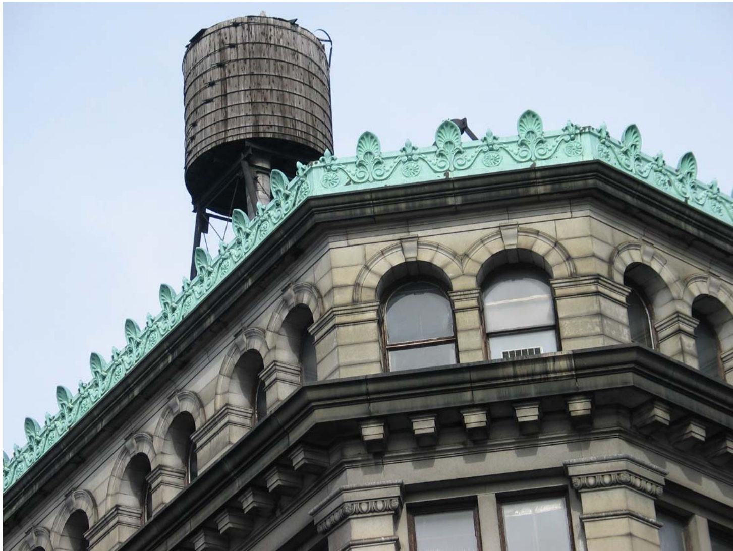
(FORMER) GERMANIA BANK BUILDING , 190 Bowery (aka 1-3 Spring Street), Manhattan. Built 1898-99; Robert Maynicke, architect; Marc Eidlitz and Son, builders. Roof detail. Photo: Donald G. Presa, 2005.
