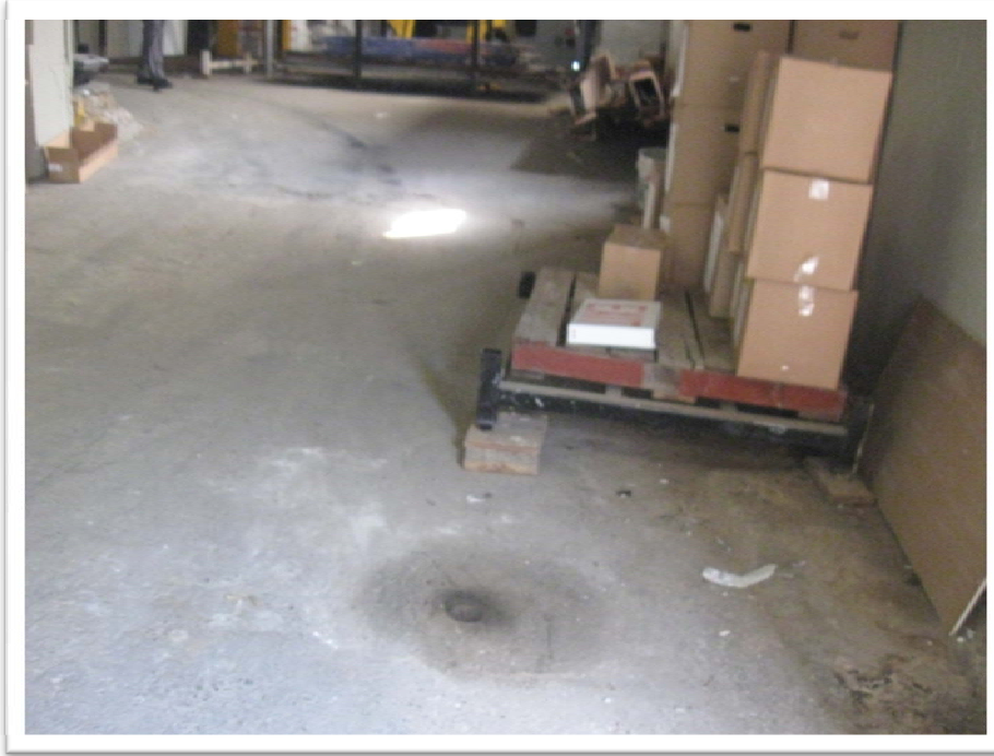
3. Suspect fill pipe inside Building F-Wall Supply Location
