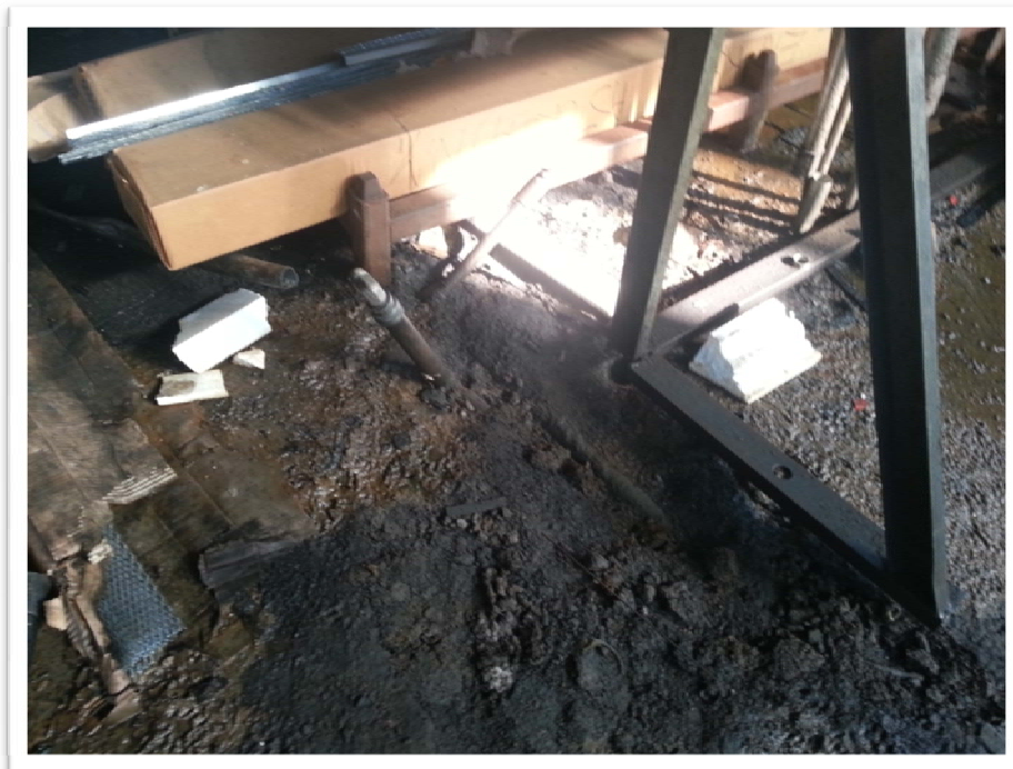
4. Oil fill lines & Staining- Building C
