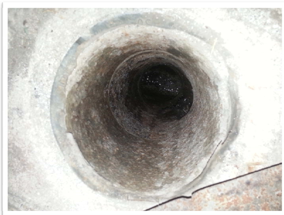
6. Suspect Floor Drains
