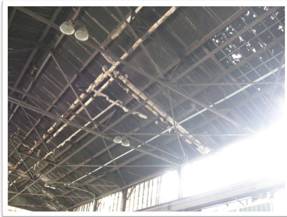
5. Suspect Asbestos- Pipe Chases
