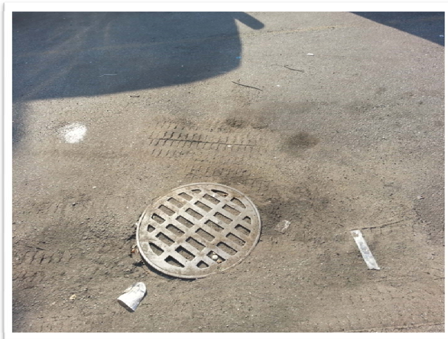
6. Typical Storm Drains of the Site
