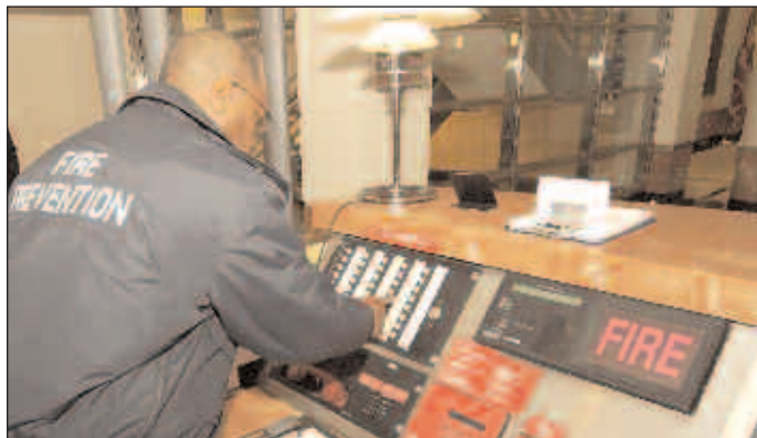
Bureau of Fire Prevention Inspector examines and tests fire alarm warning system in high-rise office building.
