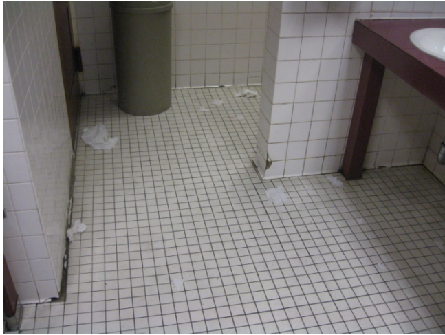
Dirty conditions in a walk-in center restroom.
