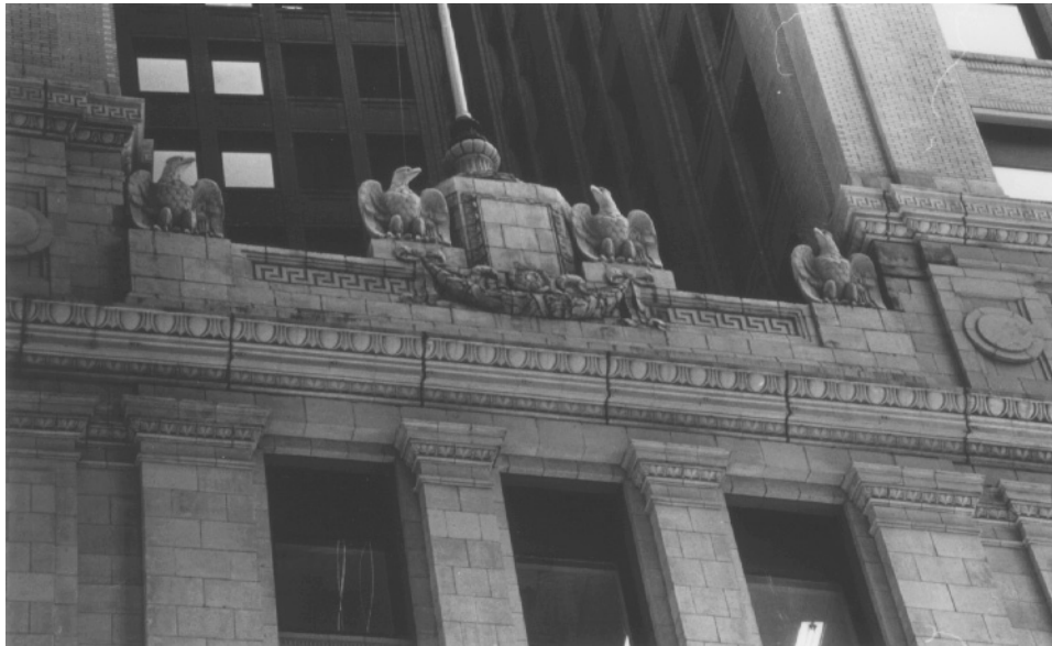
Fig. 9, Detail of the inscription above the main entrance Fig. 10, Detail of the sculpted eagles and flagpole base on the seventh story parapet Photo: Carl Forster
