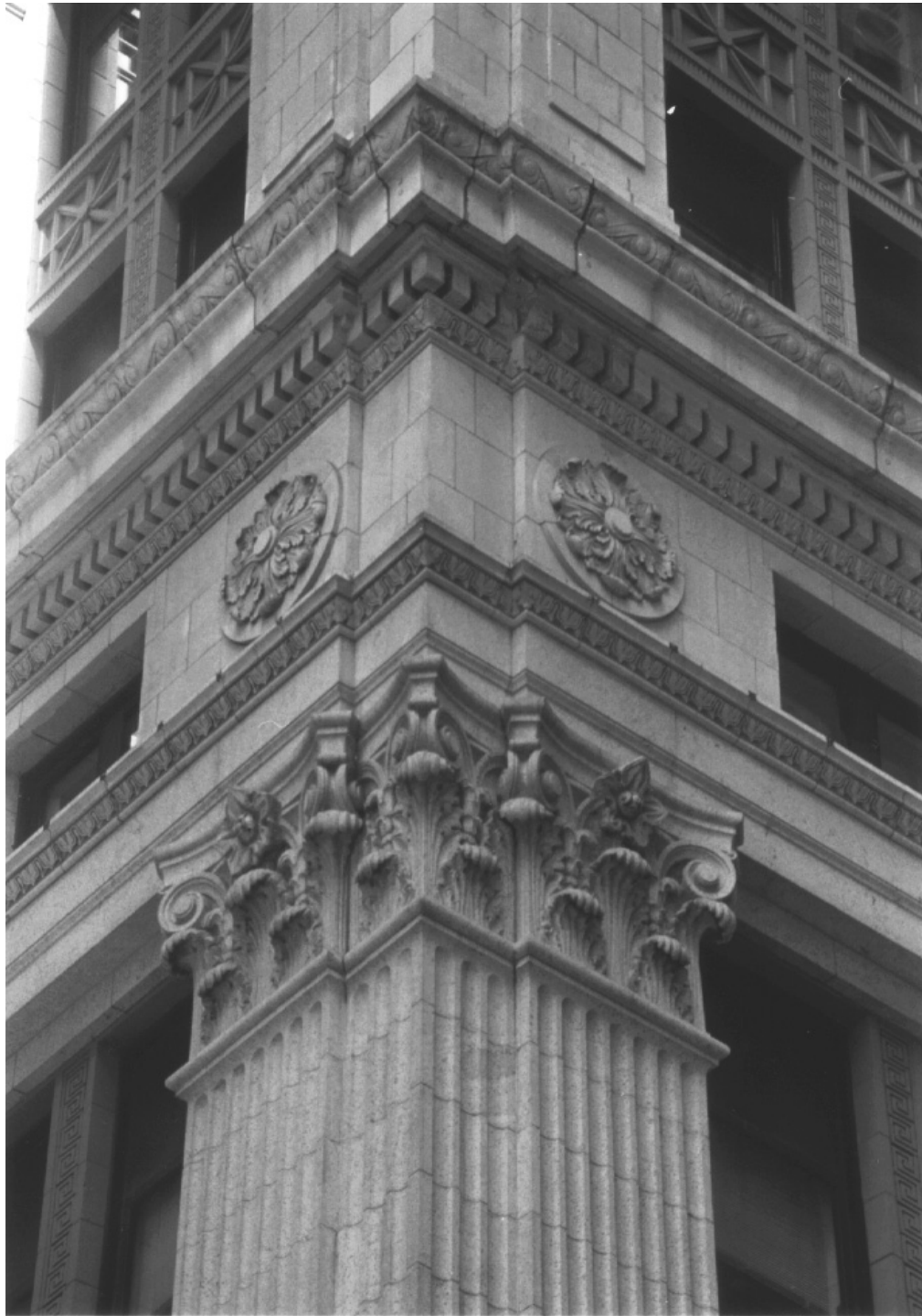
Fig. 5 Detail of the moldings on the fourth story bandcourse Photo: Carl Forster
