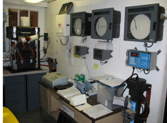
Figure 3-2 Continuous monitoring instrumentation at Kensico Reservoir (Catskill Lower Effluent Chamber).
