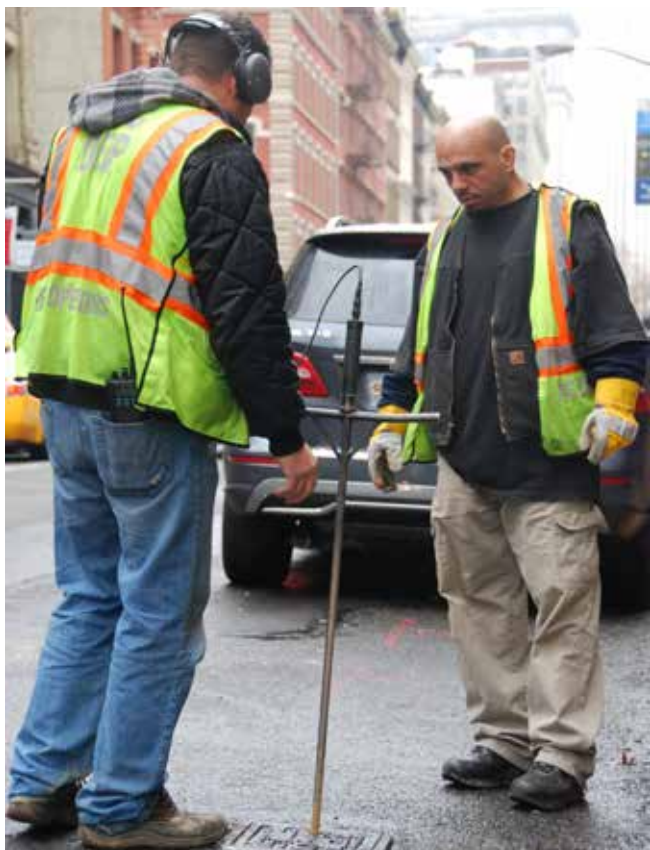
Figure 21: Sonar hearing detection for leaks
