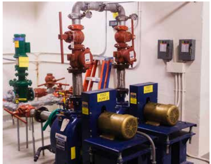
Figure 19: Water reuse system at the Solaire Building in Manhattan Photo Credit: Natural Systems Utilities
