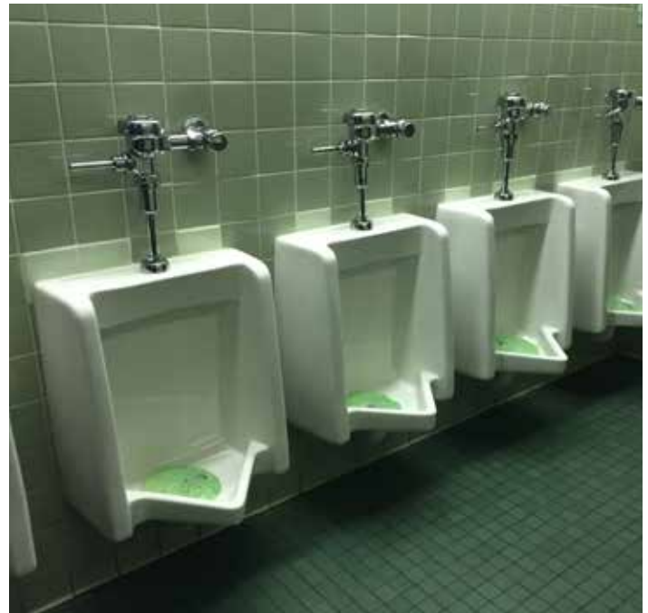
Figure 5: Retrofitted urinals at P.S.1 in Staten Island
