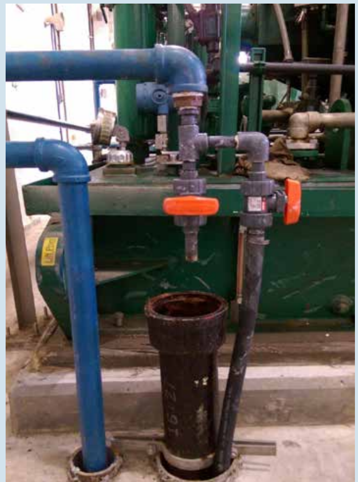
Figure 3: New equipment allows water to be recycled rather than discharged
