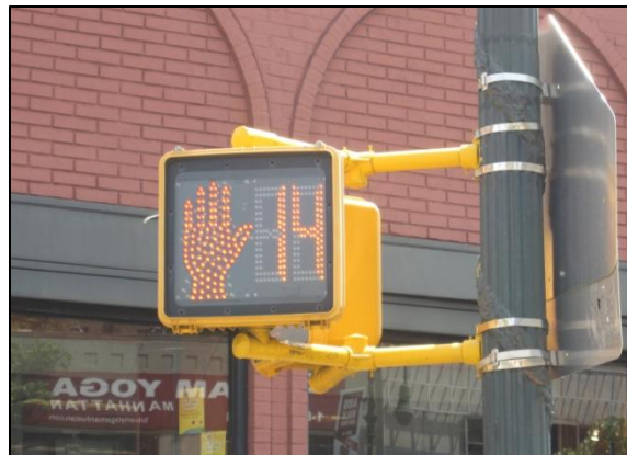
Countdown Signals: Tell pedestrians how much more time they have to cross
