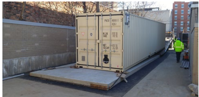
An enclosed lithium-ion battery energy storage system being installed as part of a microgrid at the Marcus Garvey Village in Brownsville, Brooklyn in March 2017
