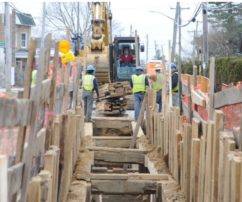
DEP installing new storm sewers in Rosedale, as part of the City’s $1.7B effort to address flooding in southeast Queens
