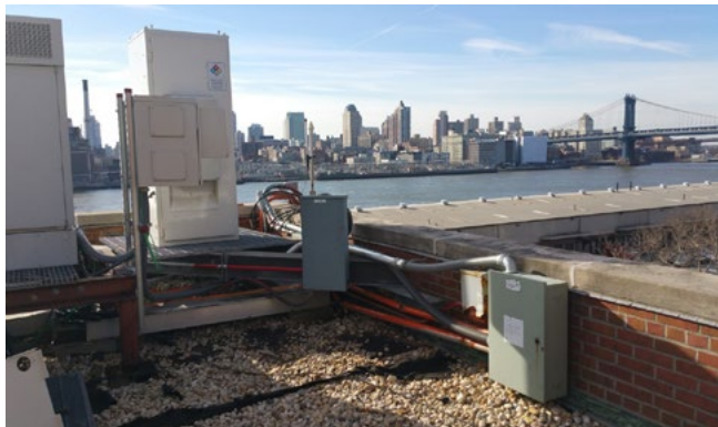
A hydrogen fuel cell, powered by methanol, sits atop a building on the East River overlooking lower Manhattan and Brooklyn.
