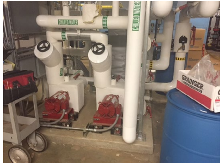
New chilled water loop and pumps installed at their office in Ozone Park, Queens.
