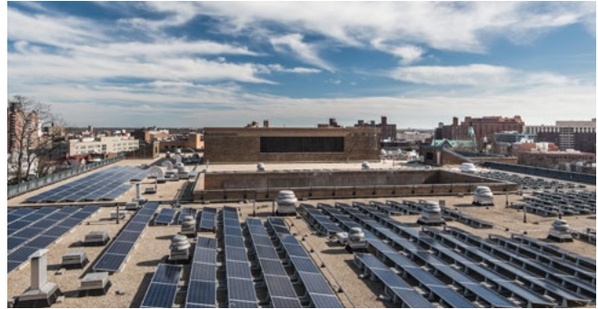
A 362 kW solar installation on Hillcrest High School in Jamaica Queens
