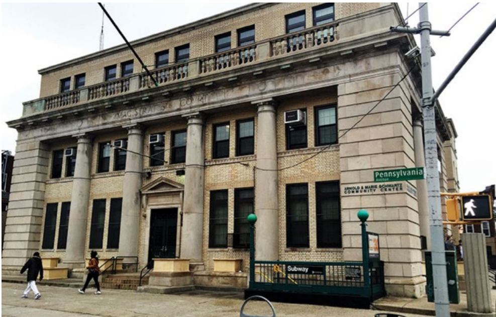
Construction began for improvements to the multi-purpose NYPD community center at 127 Pennsylvania Avenue
