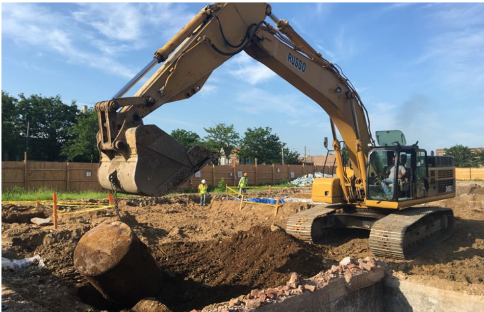
Buried tank removal at environmental remediation project in Jamaica, Queens in OER’s Vacant Land Jumpstart program
