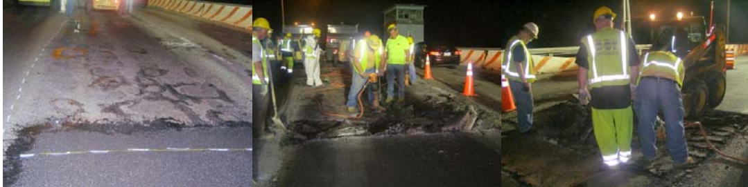
Resurfacing the Belt Parkway Bridge over Mill Basin on August 3, 2009. The Crew Completed a 13'x29' Cut in the Eastbound Center Lane, West Approach Spans. The Area Before Breakout, Exhibiting Rutting, Cracking and Excessive Patching. Breakout and Removal of Deteriorated Wearing Surface.
