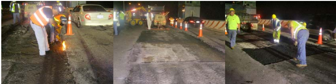
Belt Parkway Bridge over Mill Basin: Ironworker Assisting the Crew. Prepped Cut, Ready for Asphalt. Installation of New Asphalt. (Credit: Yousef Demis)
