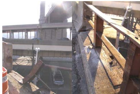
FDR Drive Safety Flag Condition - Before and After. (Credit: Bojidar Yanev)
