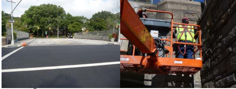
West 246 th Street Bridge in August 2009. Re-pointing the Abutment Walls and Wing Walls in October 2009.
