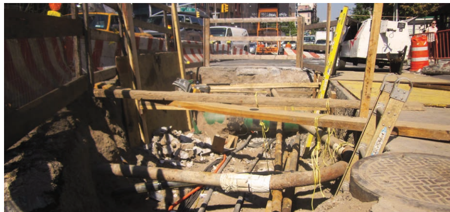
Pipe installation as part of street reconstruction. Capital projects can impact sub-surface conditions and are more comprehensive. They are managed by the Department of Design and Construction (DDC): Second Avenue at East Houston Street, Manhattan
