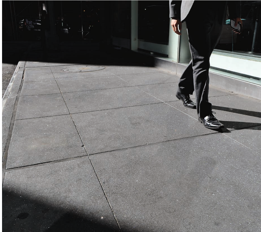
Pigmented concrete sidewalk with silicon carbide treatment, shown with non-standard flag size: Hanover Square at Pearl Street, Manhattan
