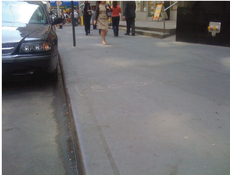
Typical pigmented concrete curb with steel facing: Beaver Street at Hanover Street, Manhattan
