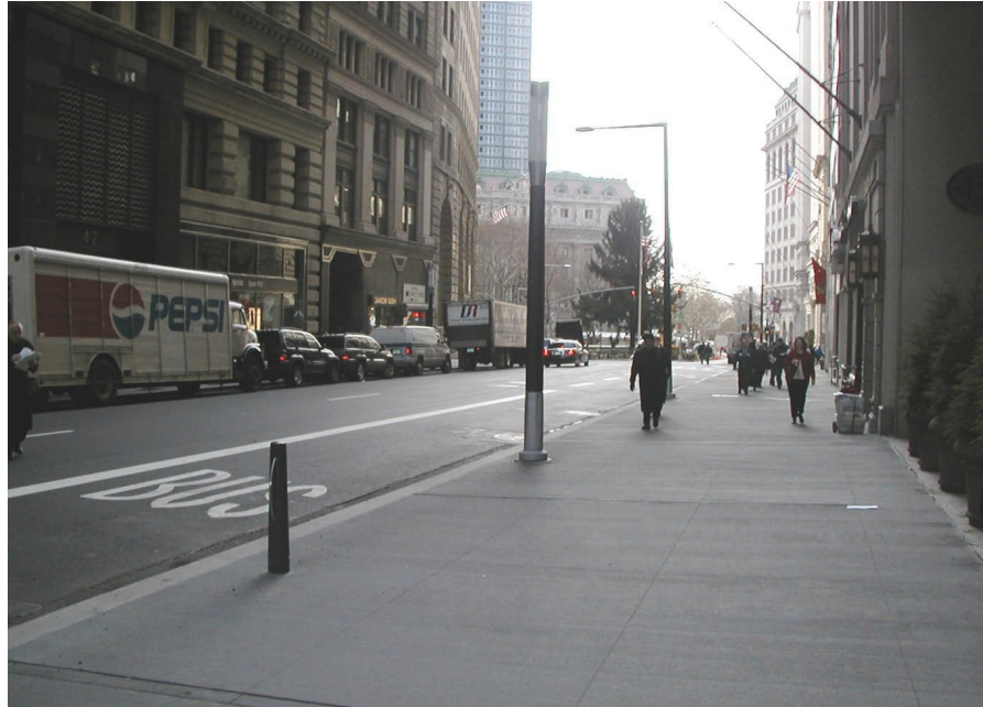
Typical dark pigmented concrete sidewalk with simulated saw-cut joint scoring: Broadway at Exchange Place, Manhattan
