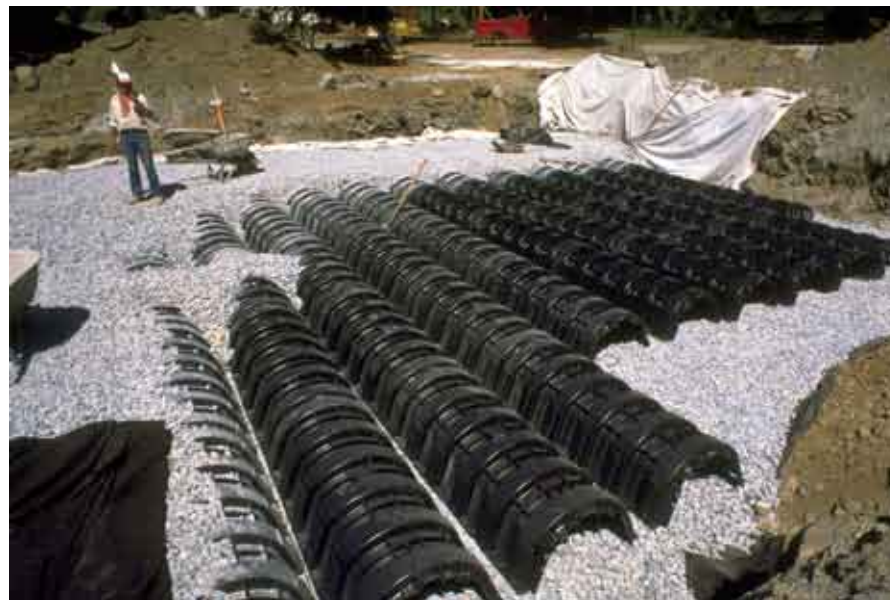
Riverdale Country School, Lower Campus – Bronx, New York Construction of recycled HDPE infiltrators below a parking lot.
