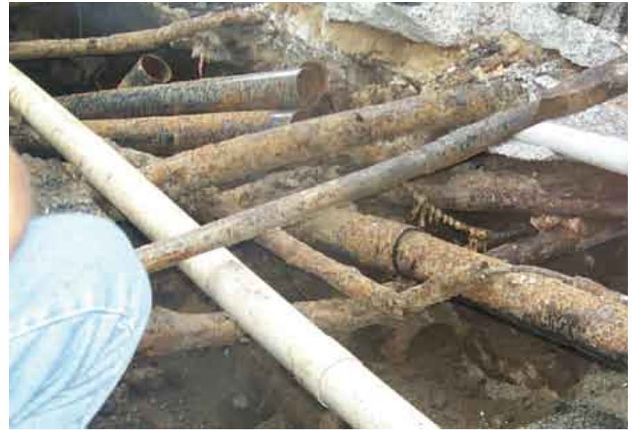
A typical situation in Manhattan in which active subsurface utilities are surrounded by abandoned and forgotten conduits, making coordination and repair difficult.
